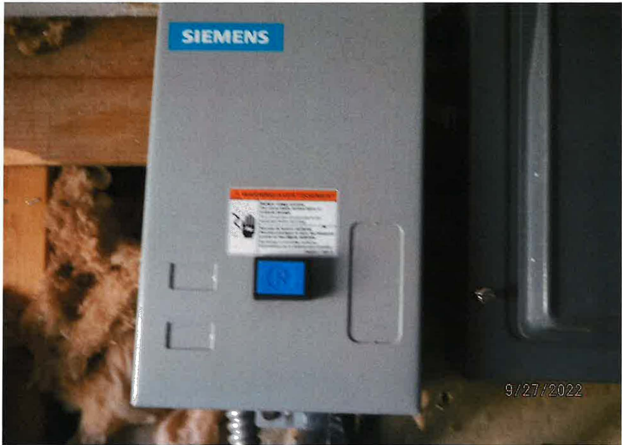
5 HP PUMP INSTALLED IN WELL
