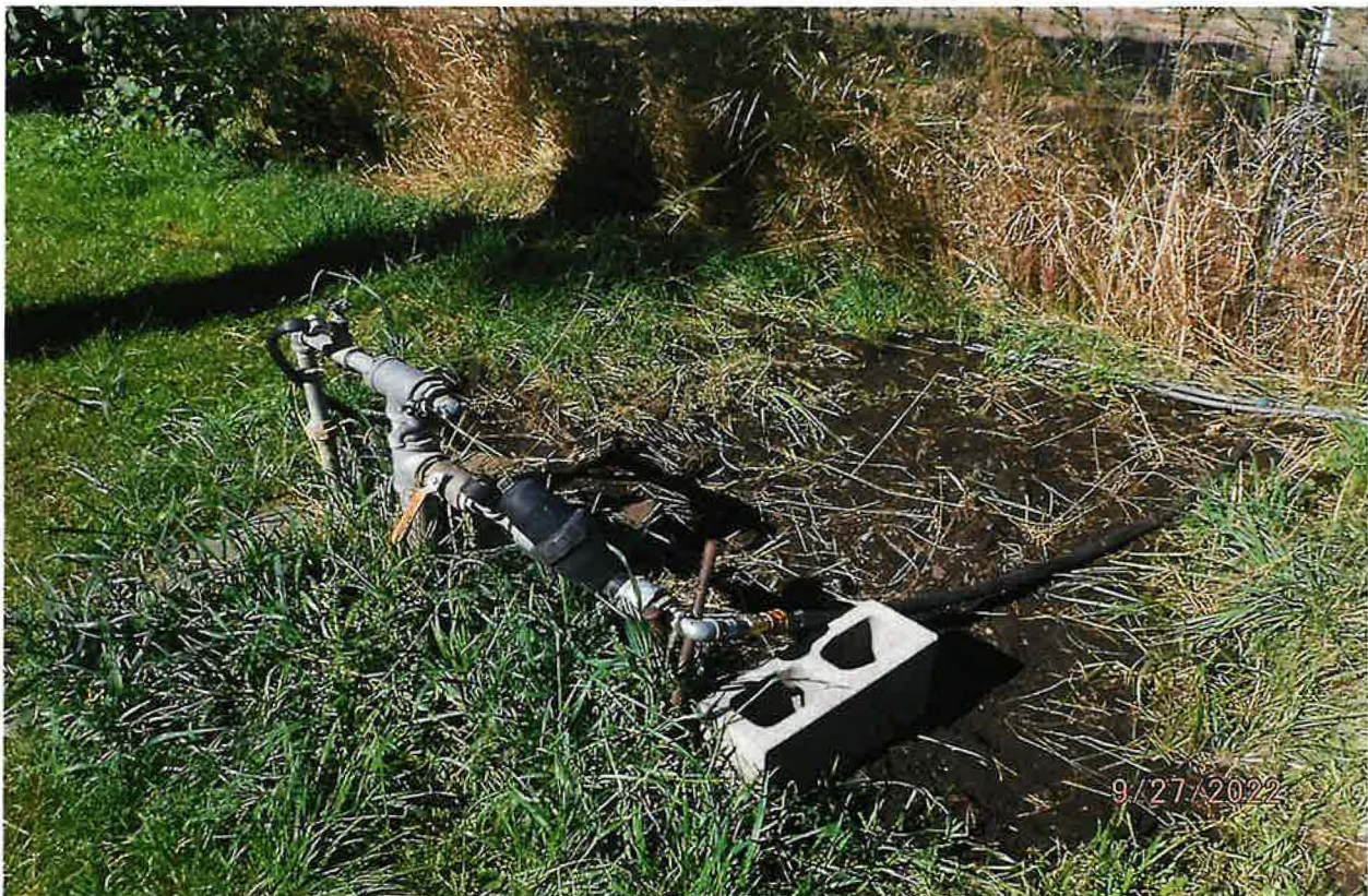
IRRIGATION RISER WITH HOSE SPLITTERS LOCATED NEAR MAIN RESIDENCE
