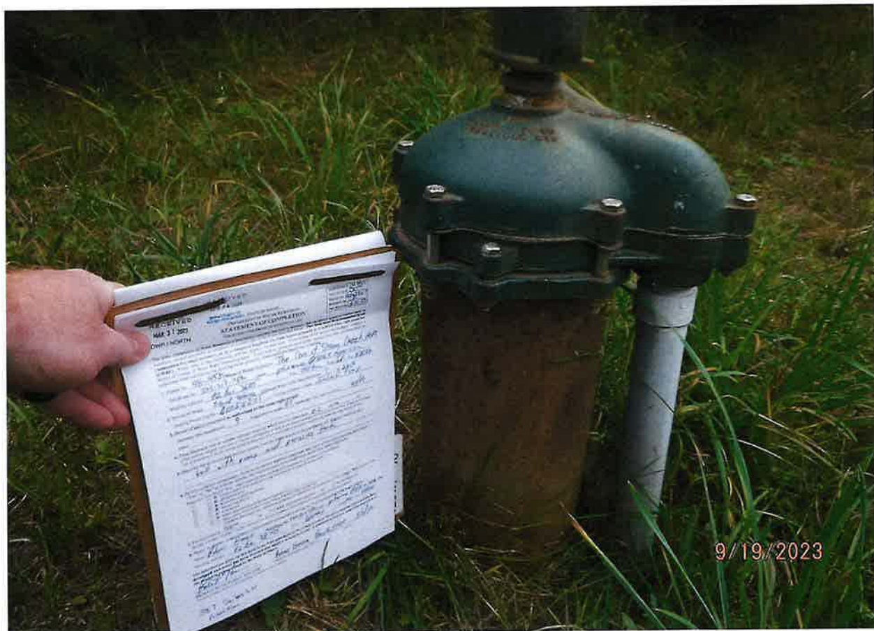
POD – GROUNDWATER WELL D0058075 (NO D-TAG VISIBLE ON UPPER 12' OF CASING)
