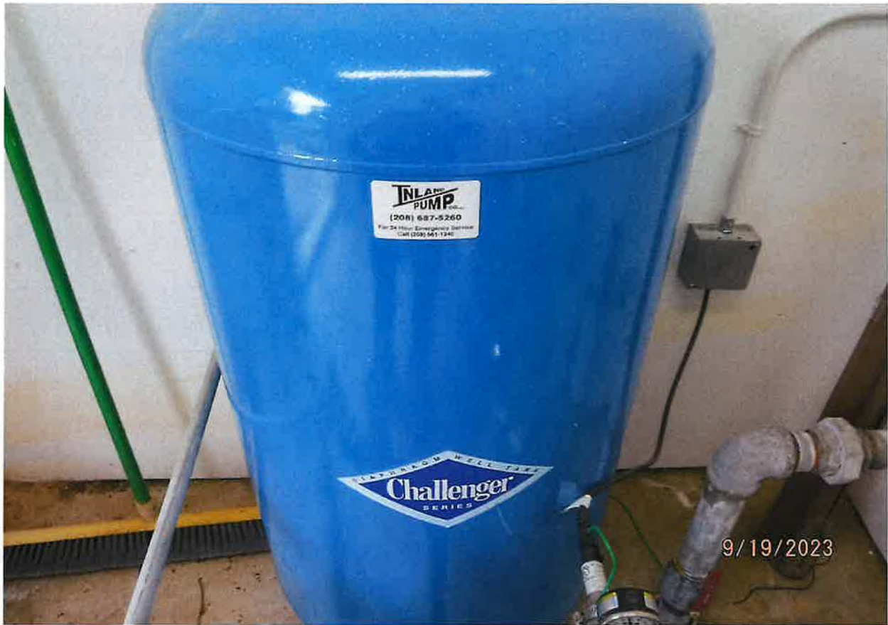
ONE 62 GAL PRESSURE TANK INSTALLED FOR DISTRIBUTION OF WATER TO NINE(9) HOMES USE
