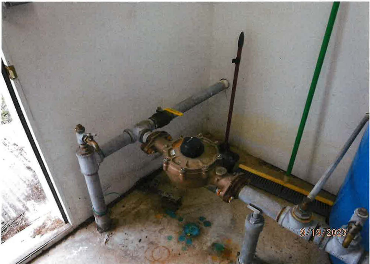
INFLOW MAIN SERVICE LINE FROM WELL (ROUTES DIRECT TO BLOWOUT VALVE PRIOR TO FLOW METER)
