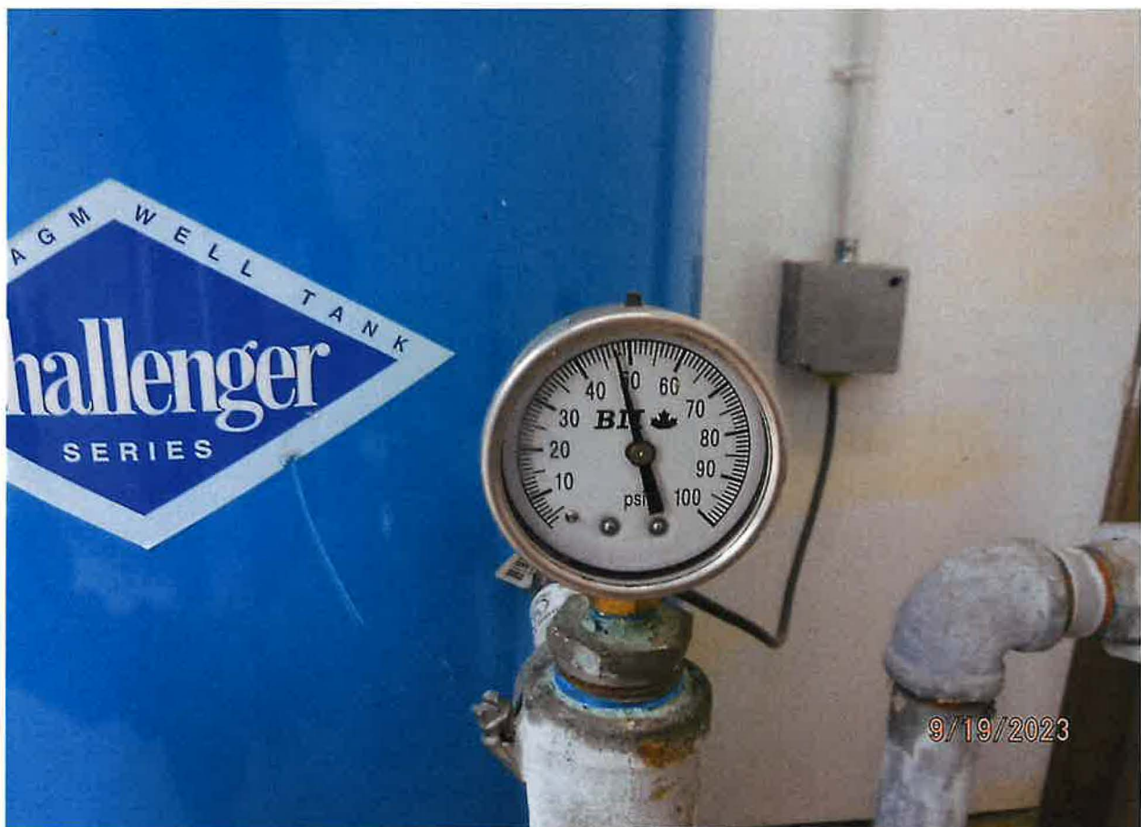
45 PSI OPERATING PRESSURE MAINTAINED IN STEADY STATE
