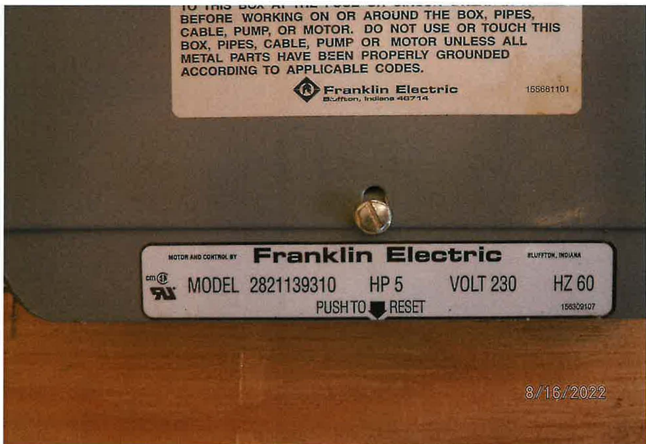
5 HP PUMP MOTOR INSTALLED IN WELL
