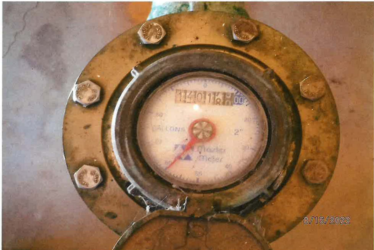
MASTER METER FLOWMETER INSTALLED
