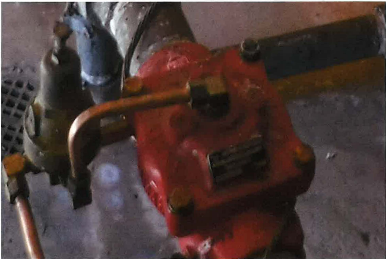
RED CYCLE STOP VALVE INSTALLED ON WATER MAIN LINE FROM WELL PRIOR TO FLOWMETER – LIMITS FLOW RATE ON SYSTEM TO APPROXIMATELY 30 GPM
