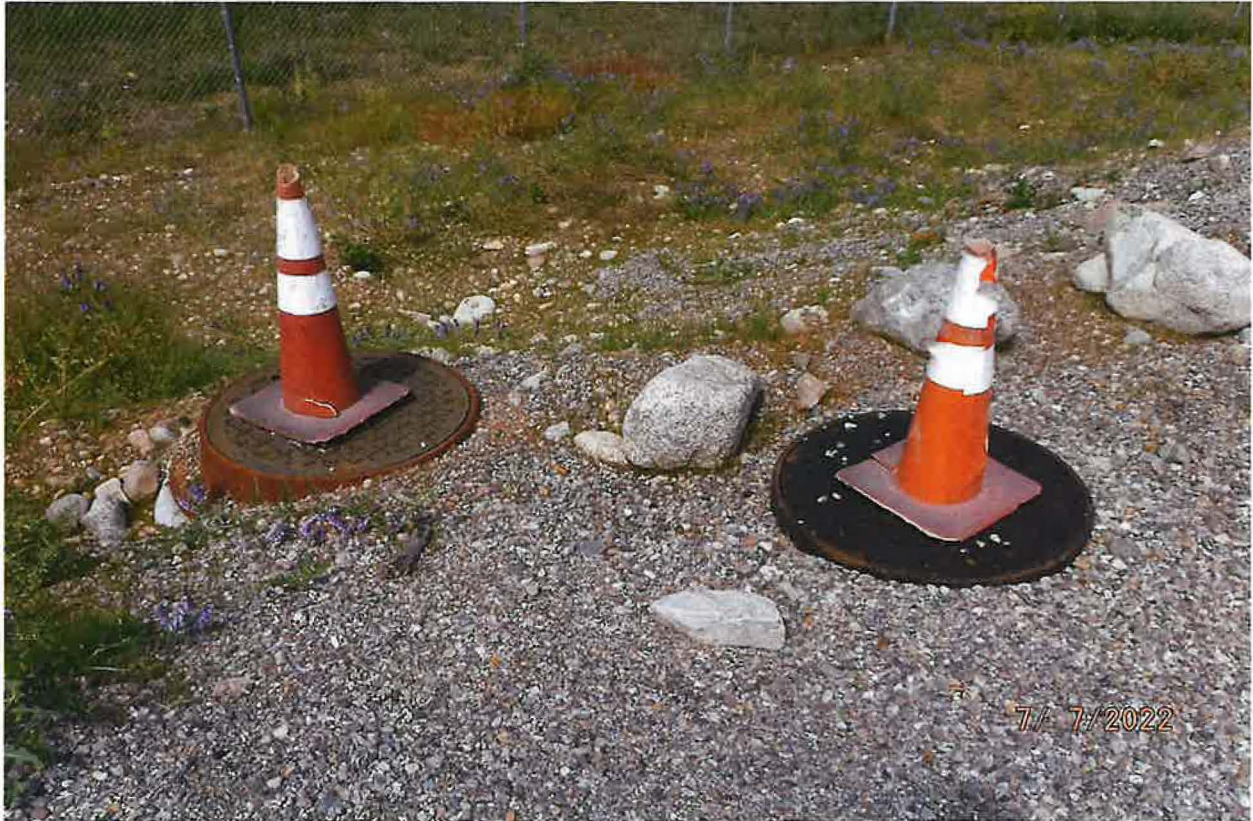
WELL HEAD VAULTED UNDER MANHOLE COVER ON R/H SIDE OF PHOTO
