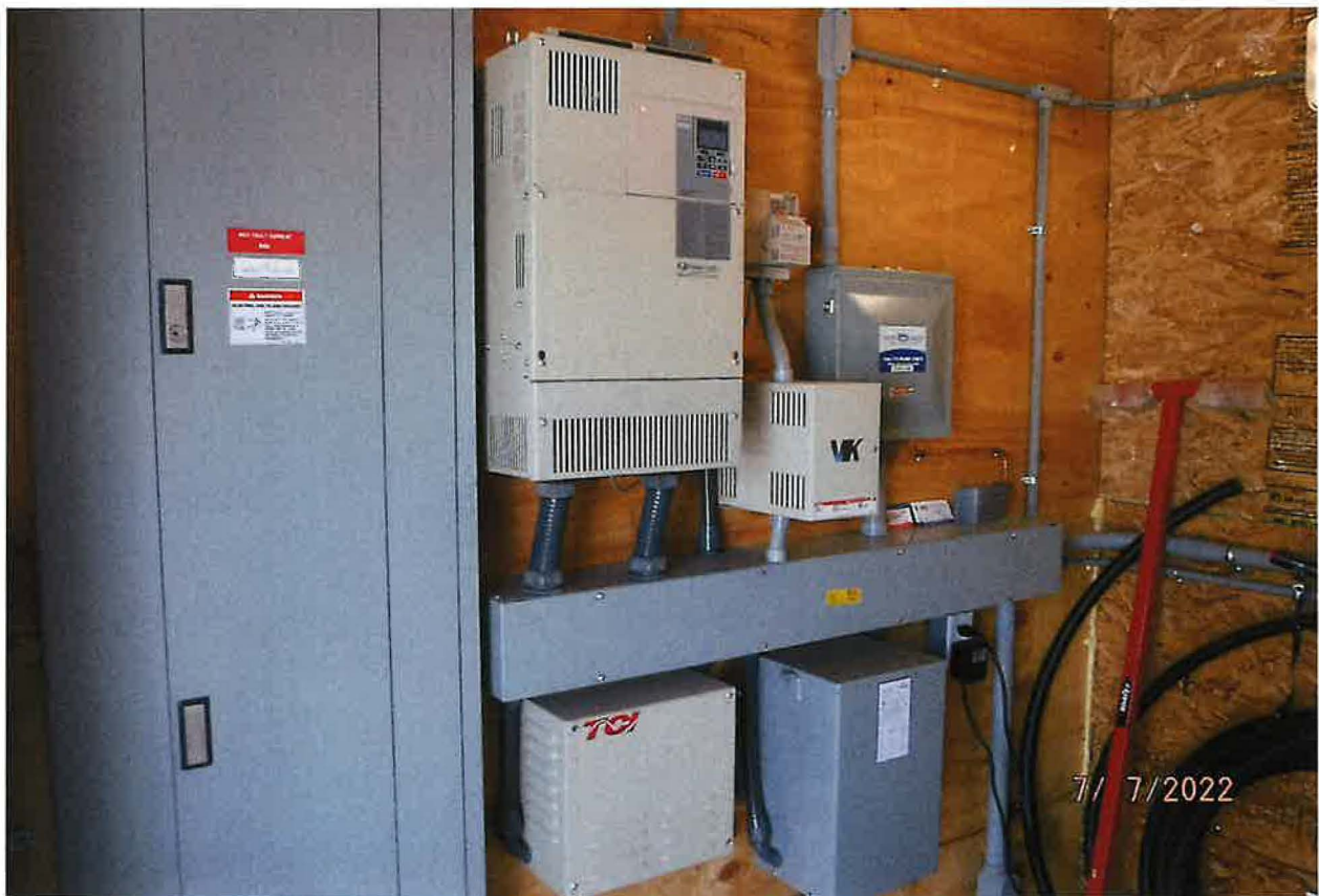
5 HP VARIABLE FREQUENCY DRIVE PUMP MOTOR INSTALLED IN WELL
