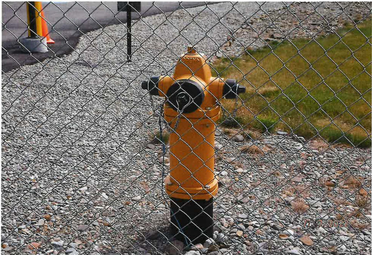
FIRE PROTECTION FROM STORAGE POU – 3EA HYDRANTS INSTALLED IN SYSTEM
