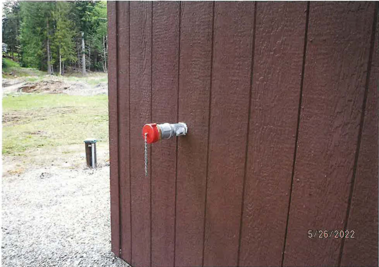
SYSTEM DEVELOPED WITH A FIRE PROTECTION CONNECTION POINT AT POWER STATION.
