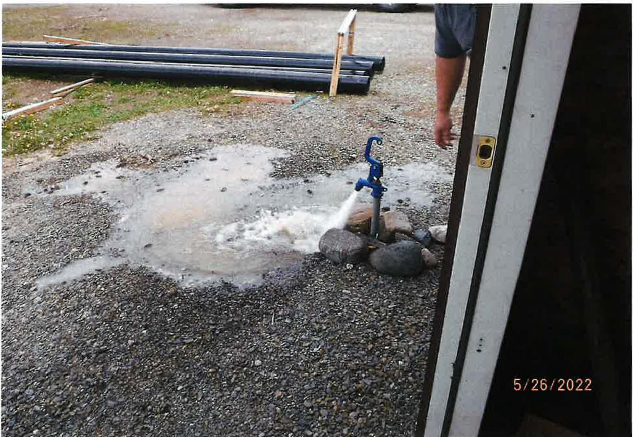
FROST FREE HYDRANT LOCATED OUTSIDE PUMP STATION
