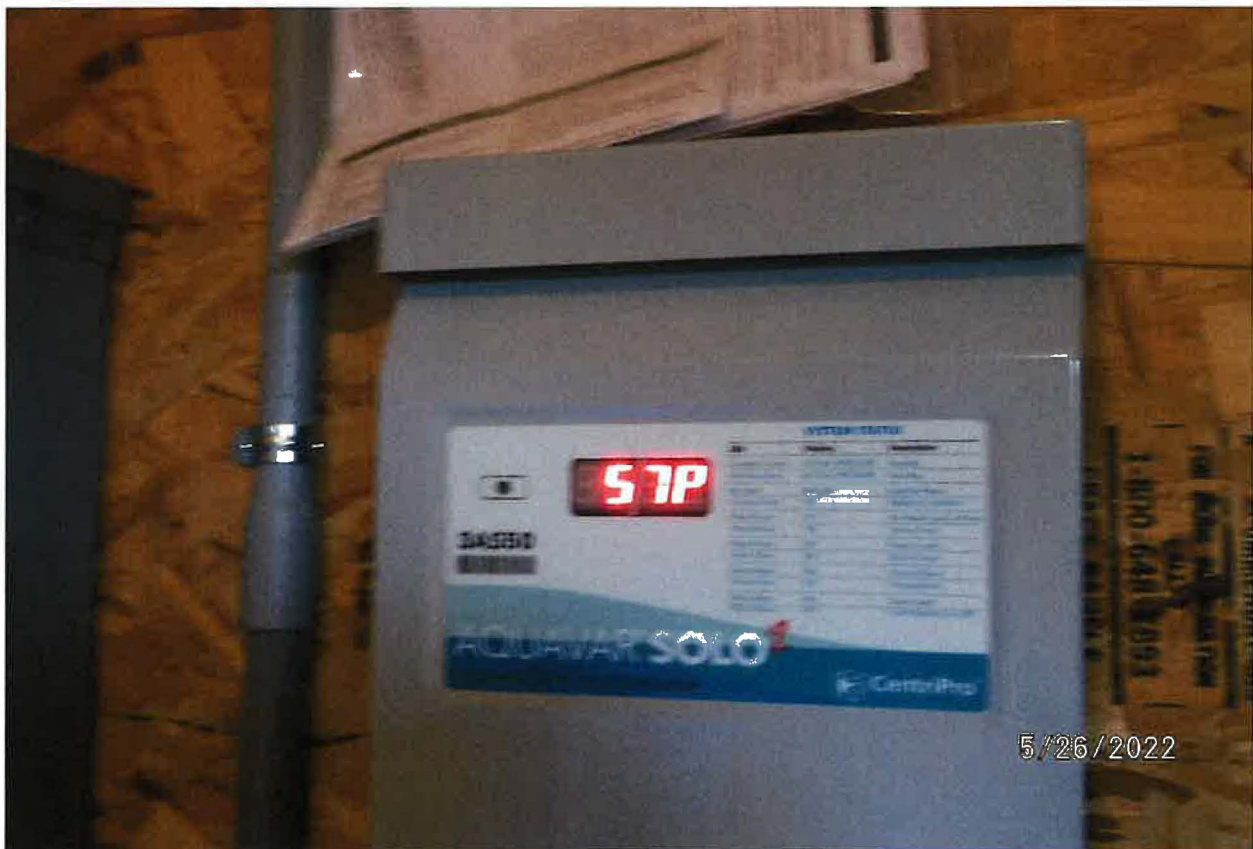
VARIABLE FREQ DRIVE WELL PUMP INSTALLED – 3 HP
