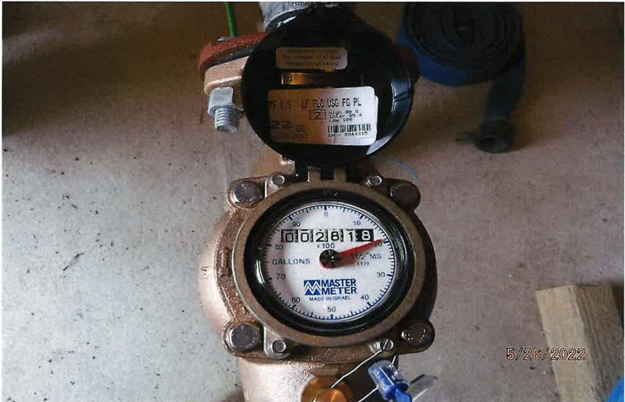
METER MASTER FLOWMETER INSTALLED IN SYSTEM, INSTANTANEOUS FLOW MEASUREMENTS TAKEN FROM THIS METER WITH PRESSURE TANKS ISOLATED FROM SYSTEM
