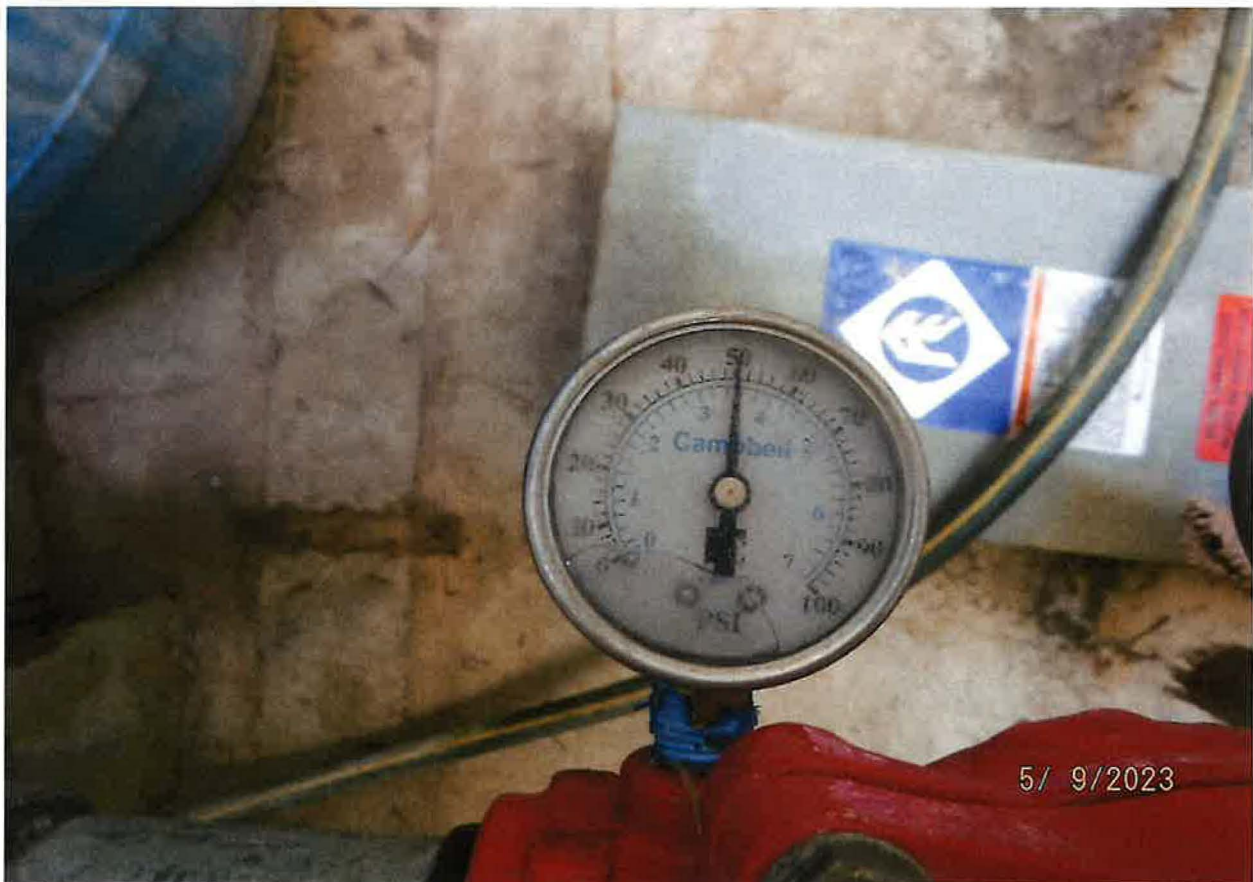
50 PSI WATER SYSTEM OPERATING PRESSURE
