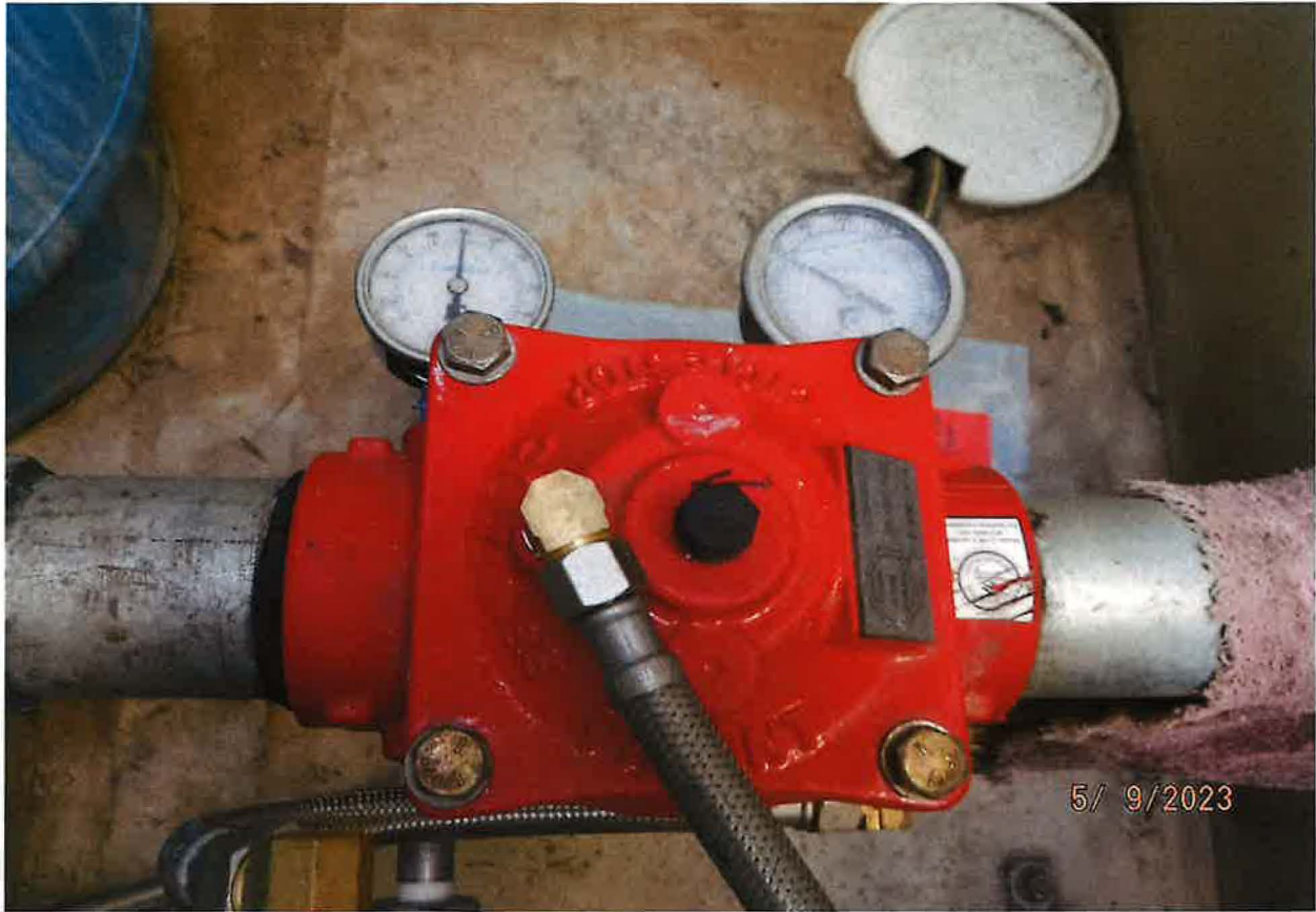
WATER CONVEYANCE SYSTEM INCORPORATES A CYCLE STOP VALVE, WHICH REGULATES FLOWRATE TO APPROXIMATELY 50 GPM
