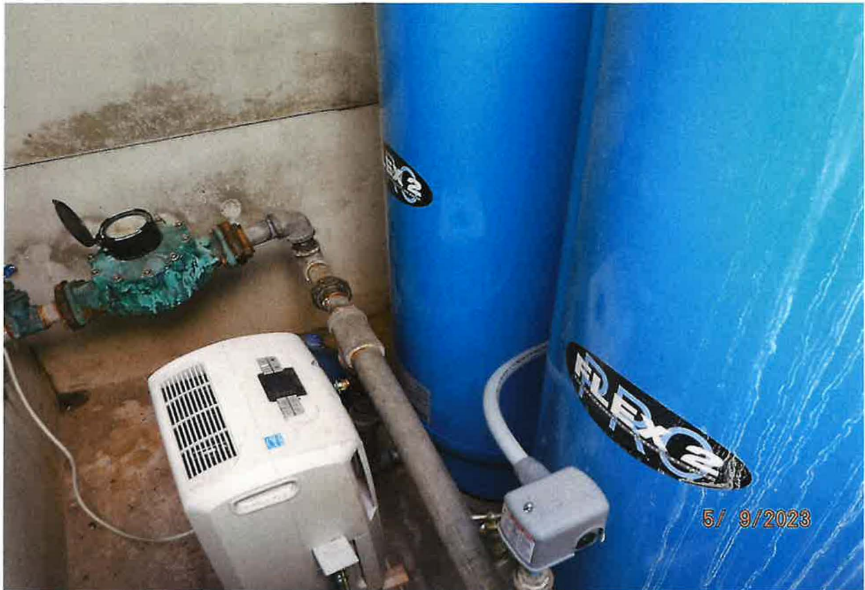
TWO PRESSURE TANKS INCLUDED IN DIVERTING WORKS FOUND IN VAULT
