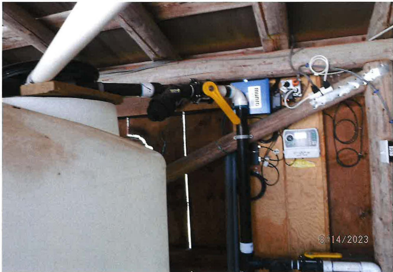
INFLOW BLACK PIPE FROM CREEK DIVERSION TO TANK – BALL VALVE TO REGULATE FLOW
