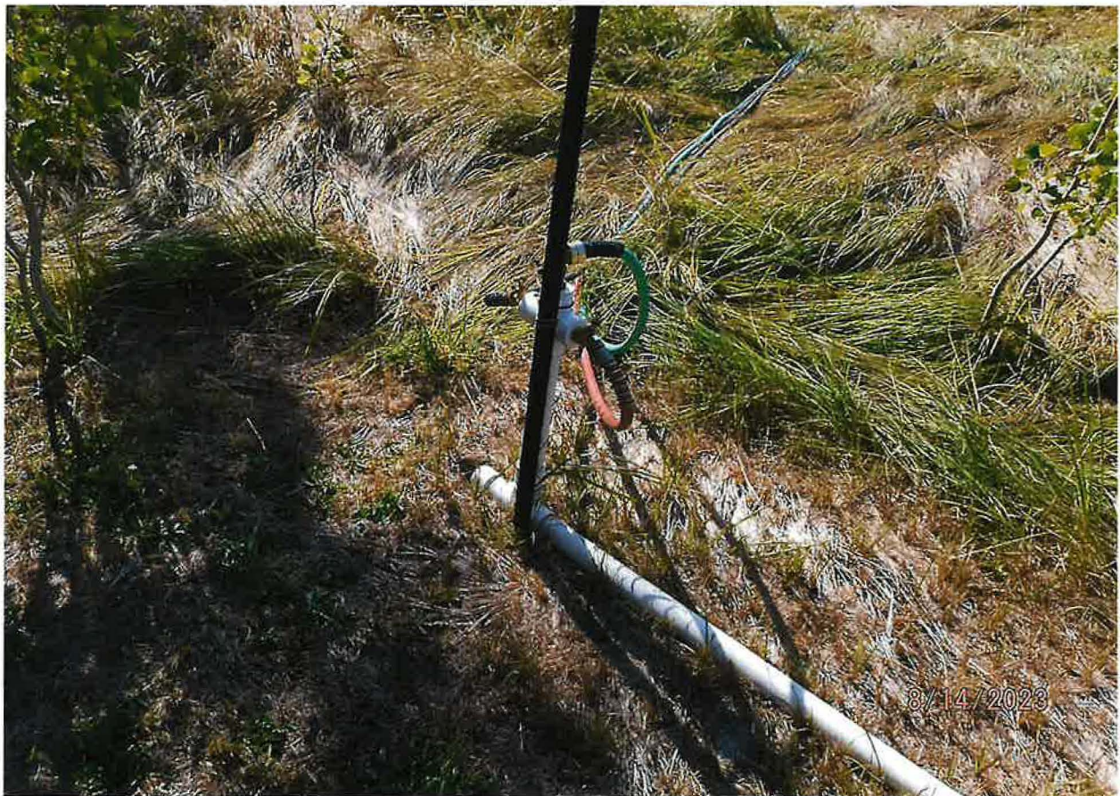
IRRIGATION POU – RISER PIPES TO HOSE AND SPRINKLER ATTACHEMENTS LOCATED AT INTERVAL ALONG IRRIGATION TRUNK LINE(S)
