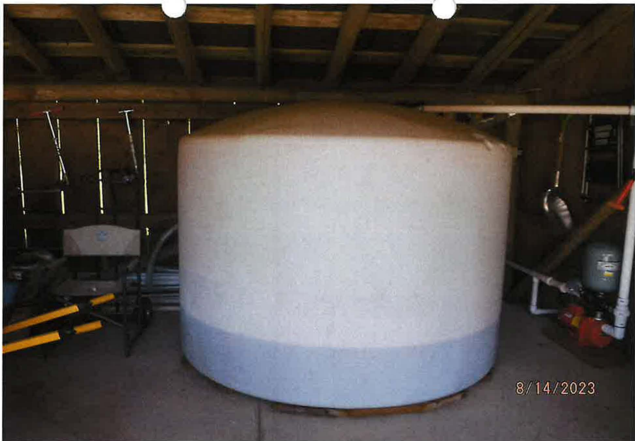
1,500 GAL STORAGE TANK WITH 1 HP RED LION TRANSFER PUMP TO IRRIGATION SYSTEM
