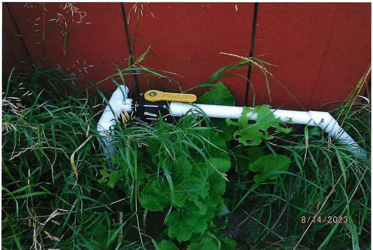
CONVEYANCE SYSTEM FOR IRRIGATION INCORPORATES BURIED PVC PIP AND BALL VALVES TO REGULATE FLOW AT EACH IRRIGATION ZONE
