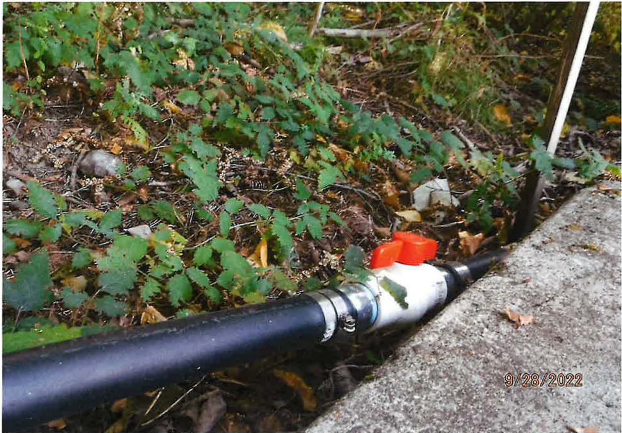
1 ½ INCH POLY PIPE FROM PUMP TO PRESSURE TANK & TO IRRIGATION RISER VALVES
