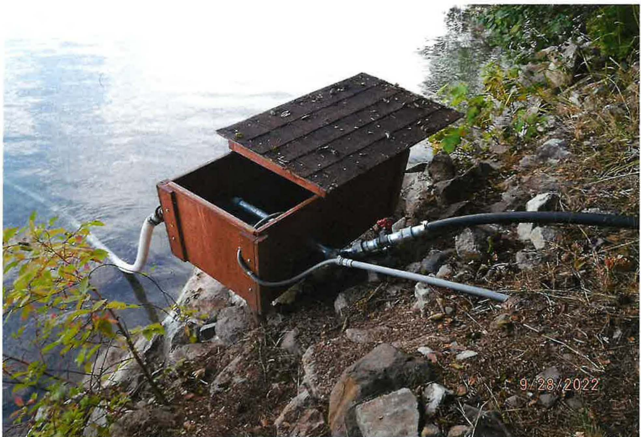
POD – PUMP WITH INTAKE PIPE IN RIVER
