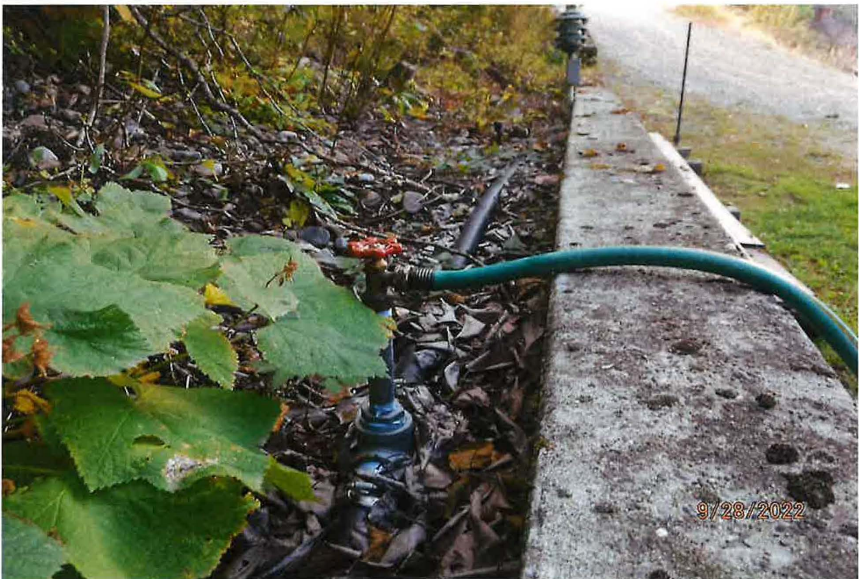
IRRIGATION RISER HOSE BIBE LOCATED AT IRRIGATION AREA ALONG RIVERFRONT
