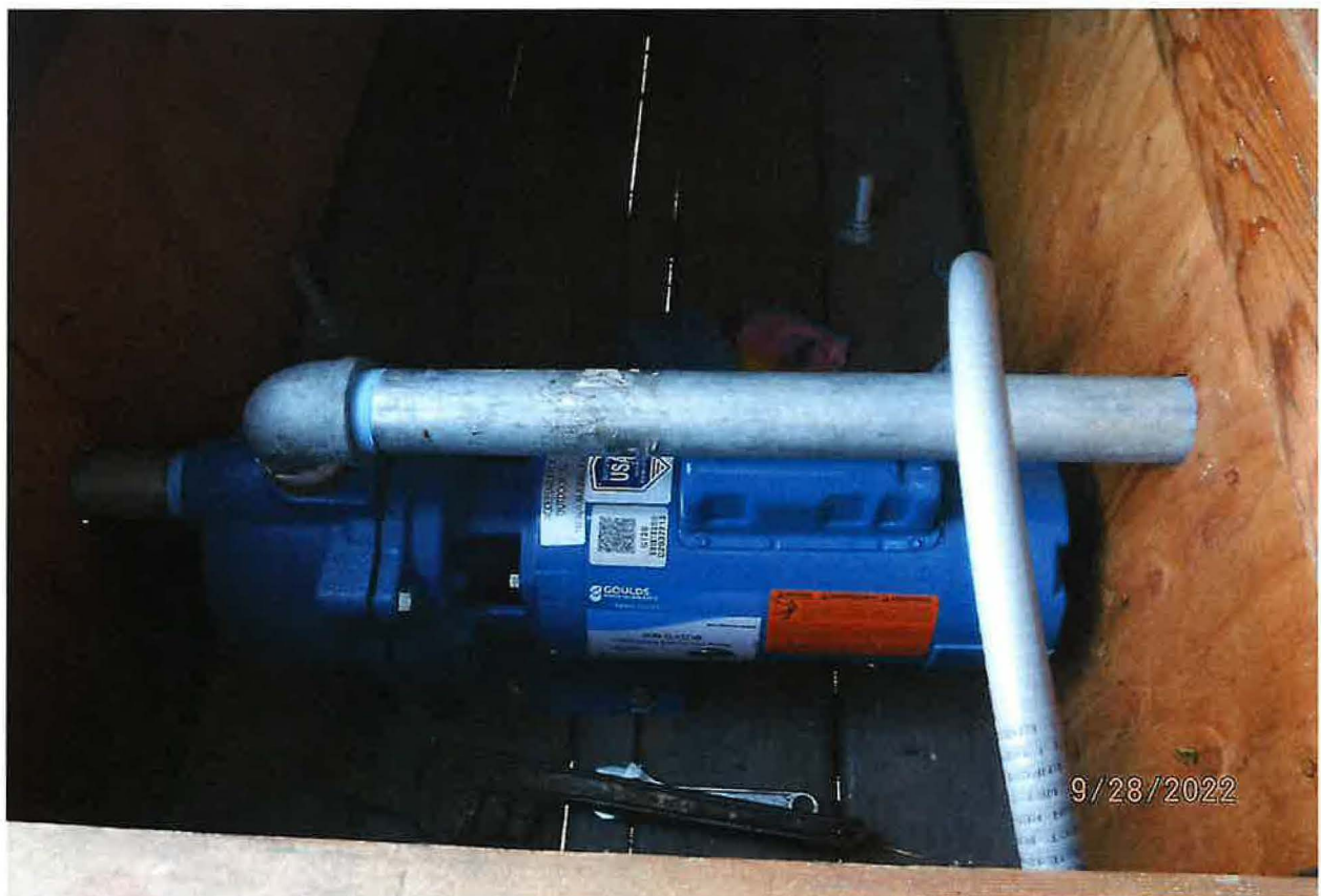
2 HP CENTRIPRO CENTRIFUGAL PUMP INSTALLED IN IRRIGATION SYSTEM
