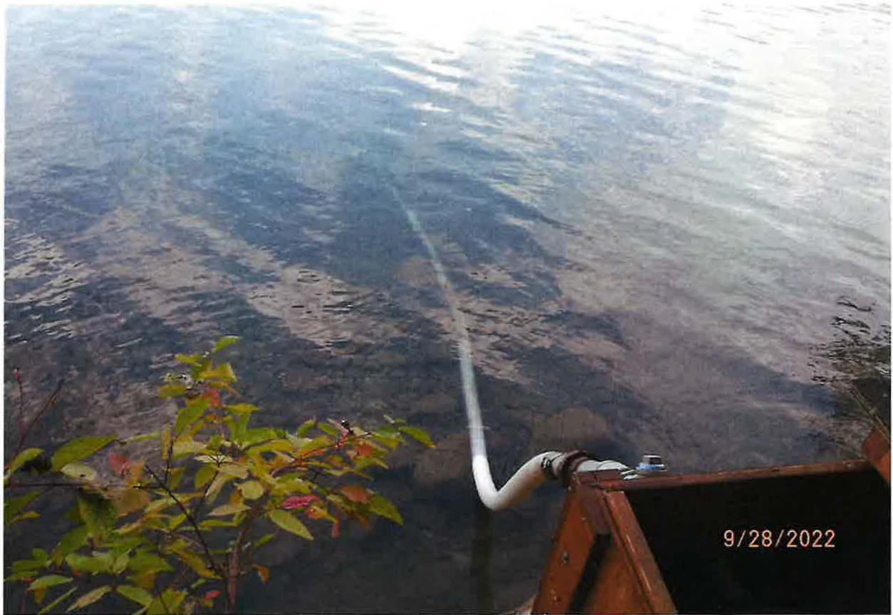
SCREENED INTAKE PIPE WITH FOOT VALVE
