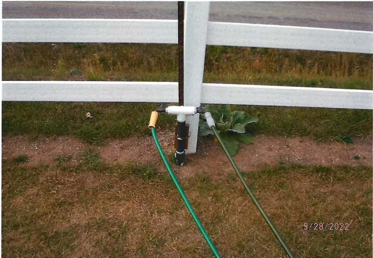
IRRIGATION RISER PIPE WITH HOSE SPLITTER
