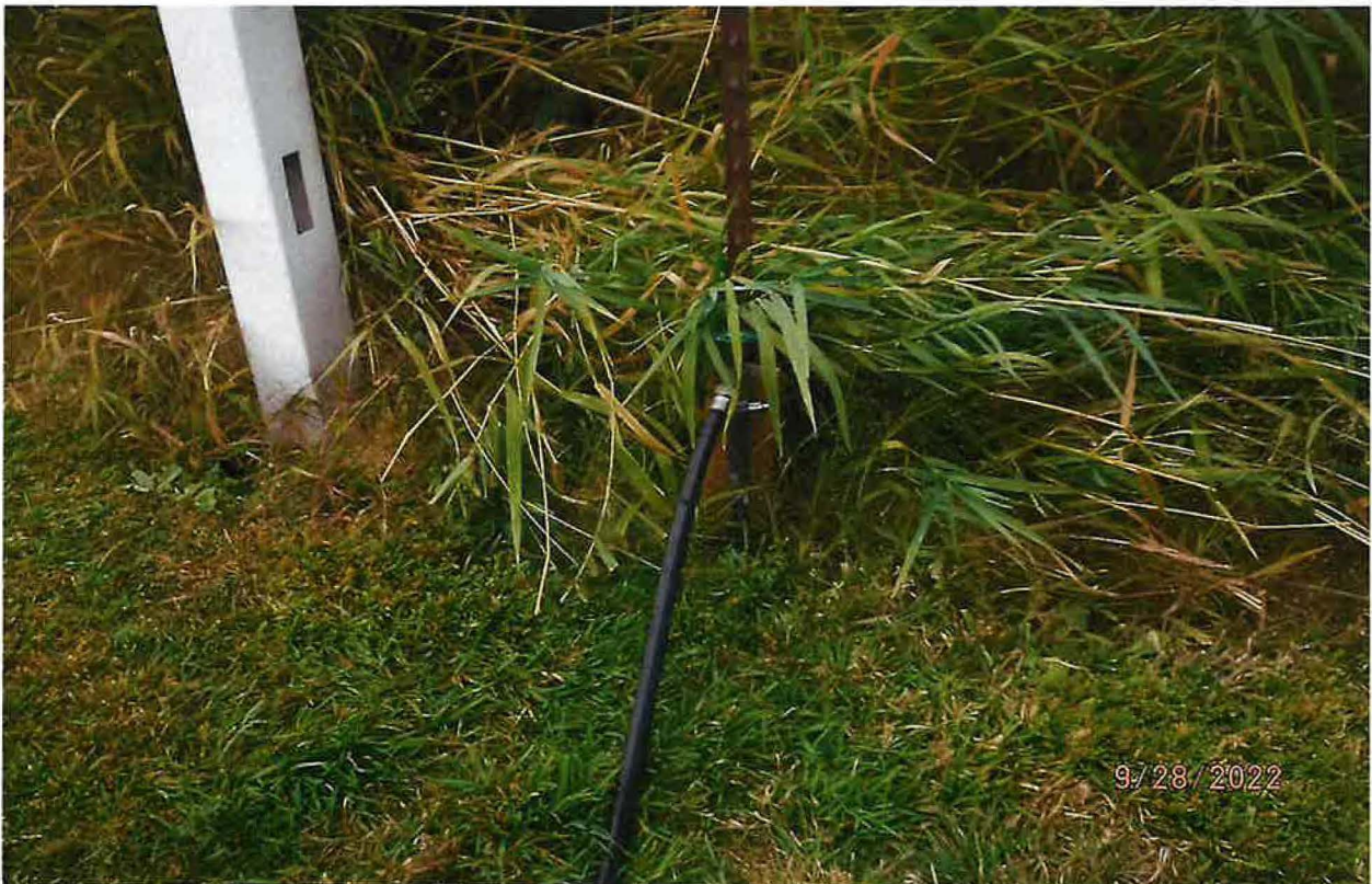
IRRIGATION RISER PIPE WITH HOSE BIB
