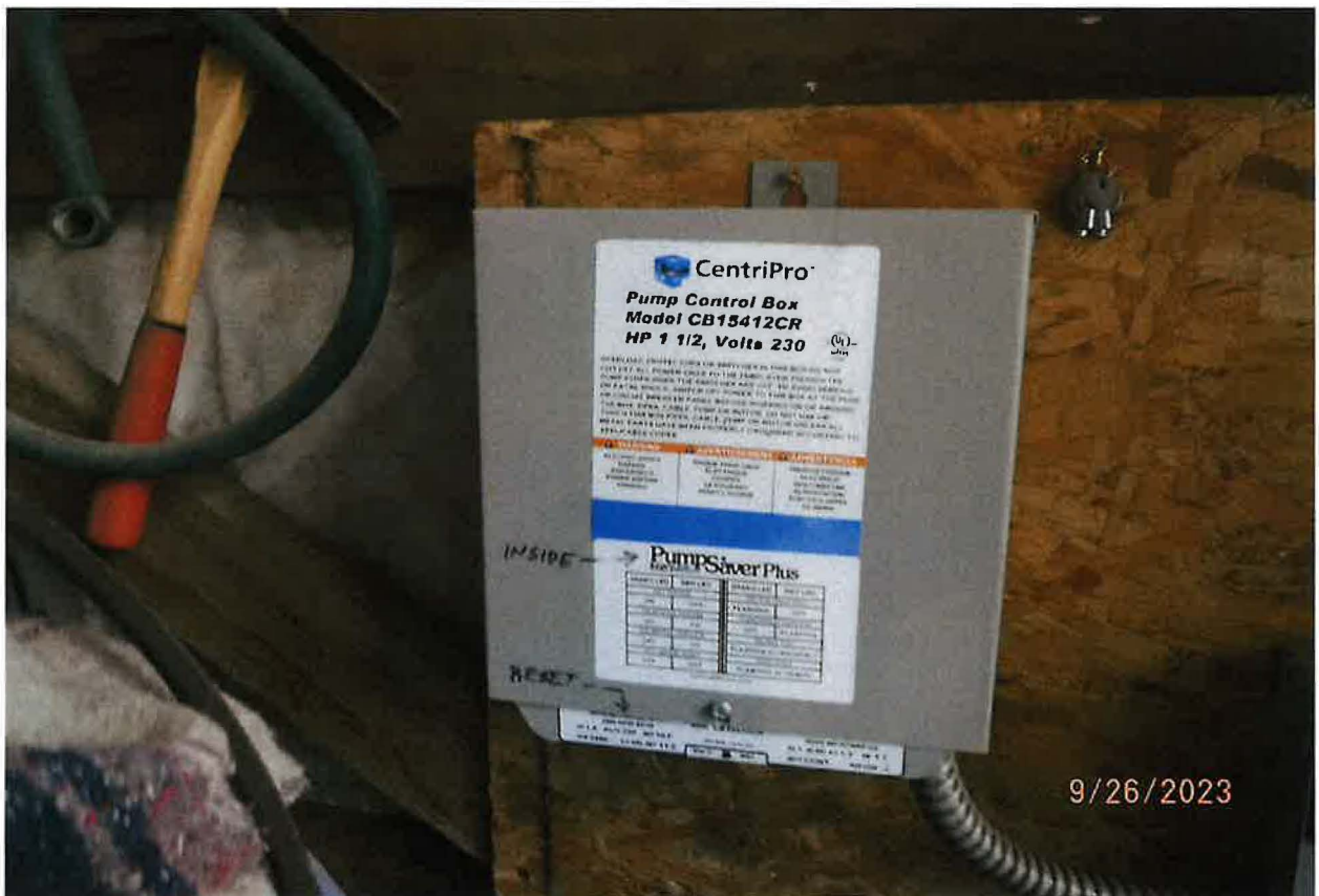
CENTRIPRO 1.5 HP PUMP MOTOR INSTALLED ON SYSTEM
