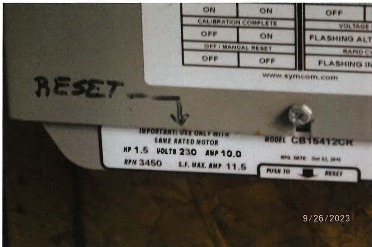
1.5 HP PUMP MOTOR
