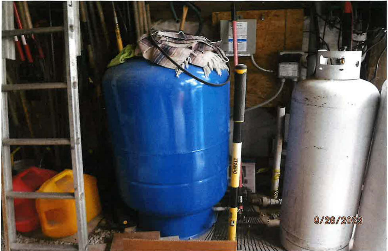
DIVERTING WORKS INCORPORATE A 1.5 HP PUMP AND BURIED PIPELINE TO PRESSURE TANK PRIOR TO MULTI-ZONE IRRIGATION SYSTEM DISTRIBUTION
