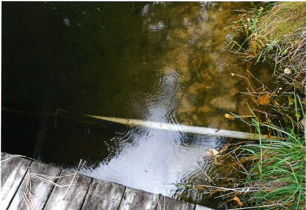
POD – SUBMERSED PUMP IN POND
