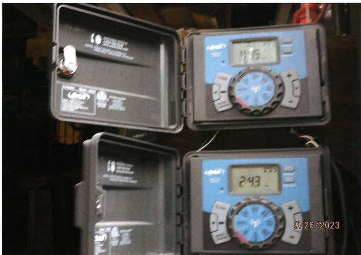
MULTI-ZONE IRRIGATION SYSTEM
