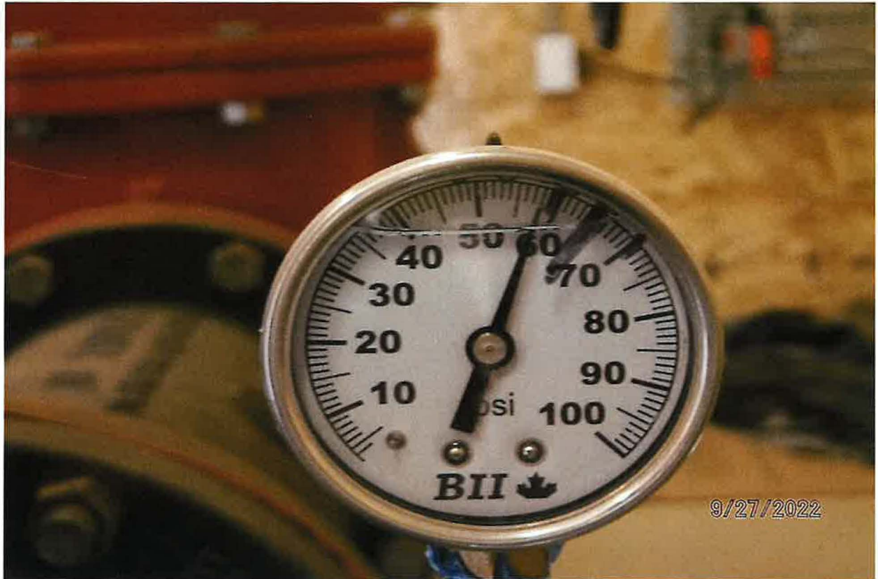
WATER SYSTEM OPERATIONAL PRESSURE 60-70 PSI
