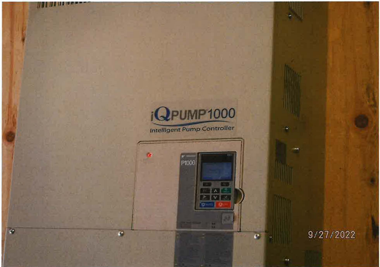
VARIABLE FREQUENCY DRIVE PUMP MOTOR INSTALLED IN SYSTEM
