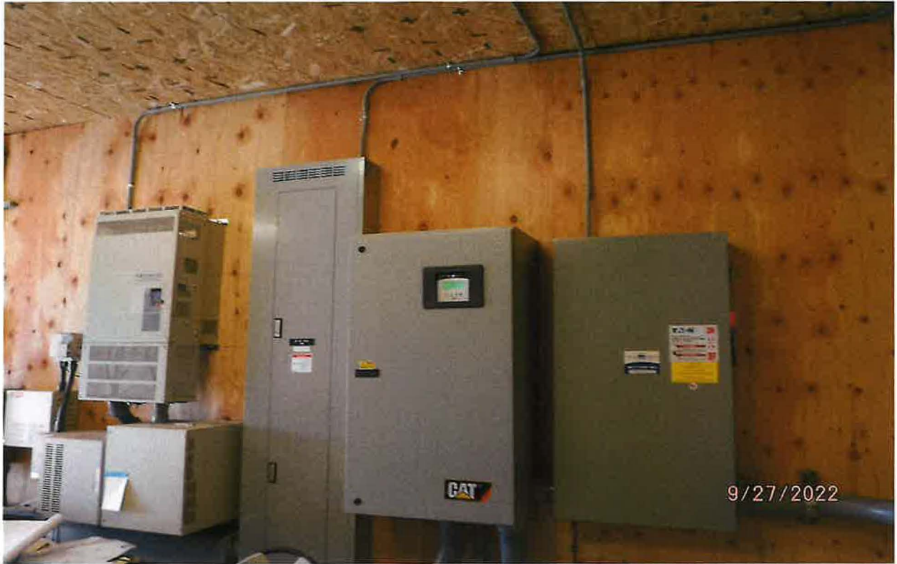
WATER SYSTEM COMPONENT CONTROL PANEL(S)
