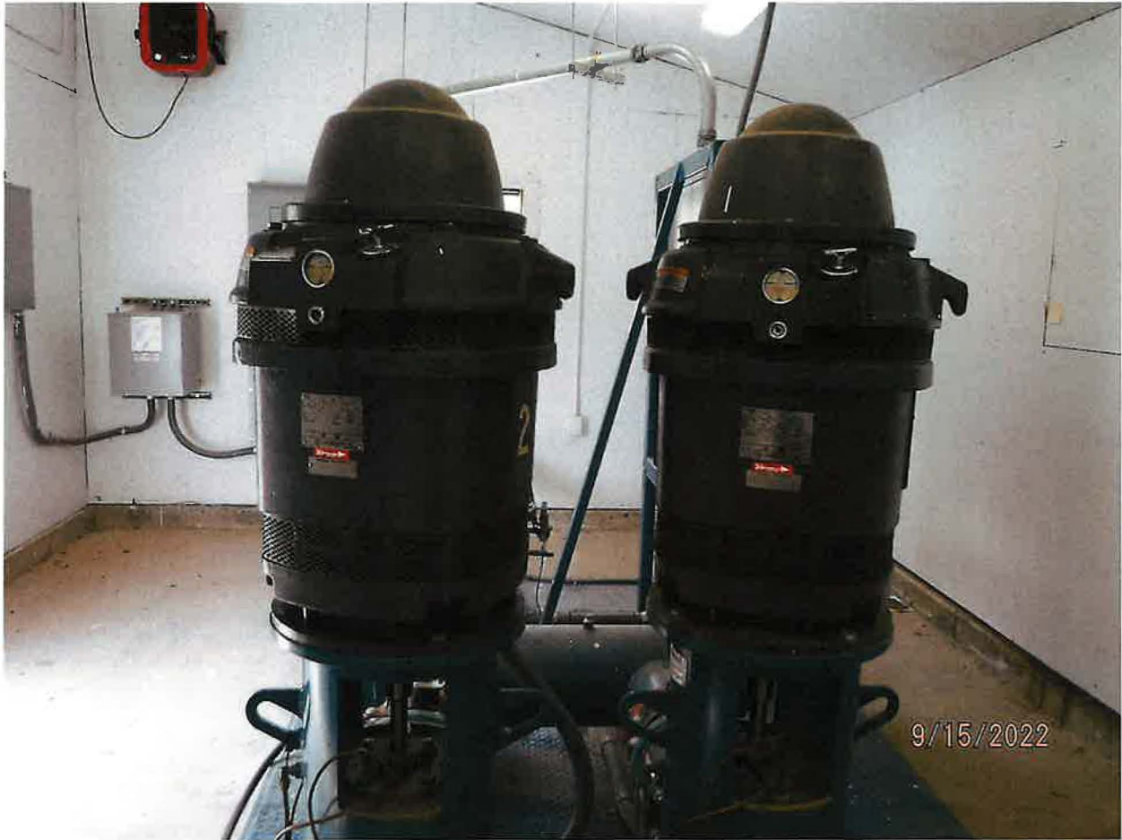
EACH PUMP IS A U.S. MOTORS BRAND PUMP
