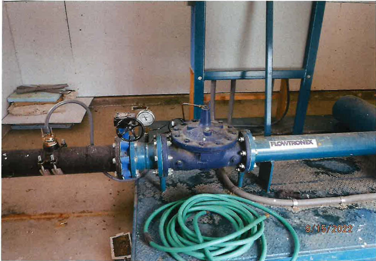
BADGER METER ULTRASONIC FLOWMETER INSTALLED ON SYSTEM
