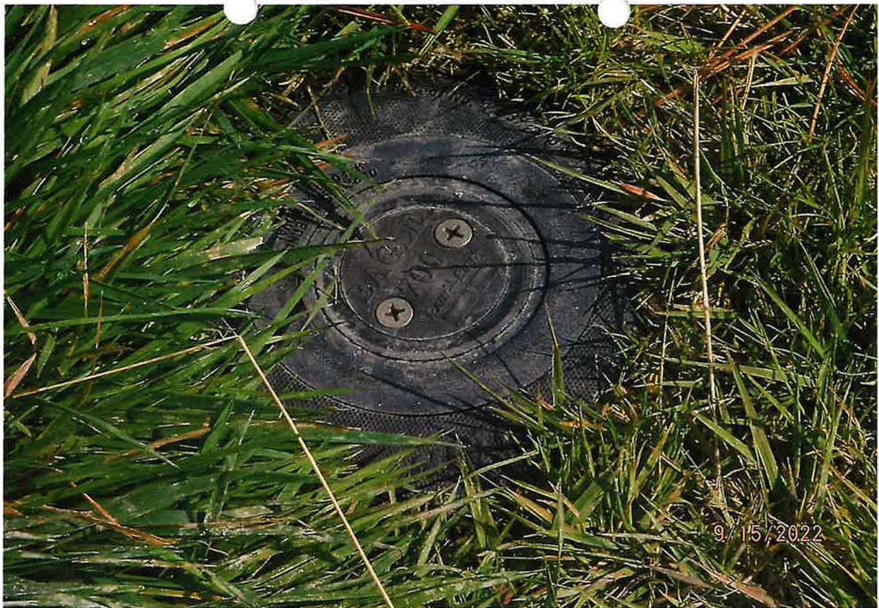
PRESSURIZED IRRIGATION FROM STORAGE USE AT POU
