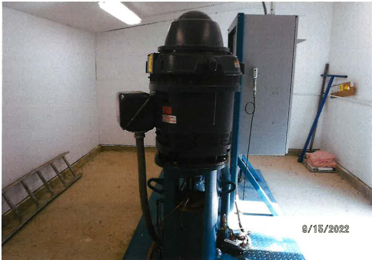
40 HP PUMP USED TO DISTRIBUTE IRRIGATION FROM STORAGE WATER
