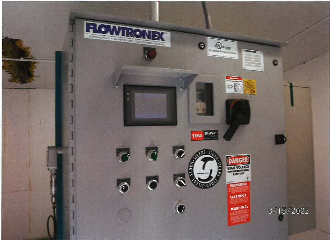
IRRIGATION FROM STORAGE PUMP CONTROL SYSTEM
