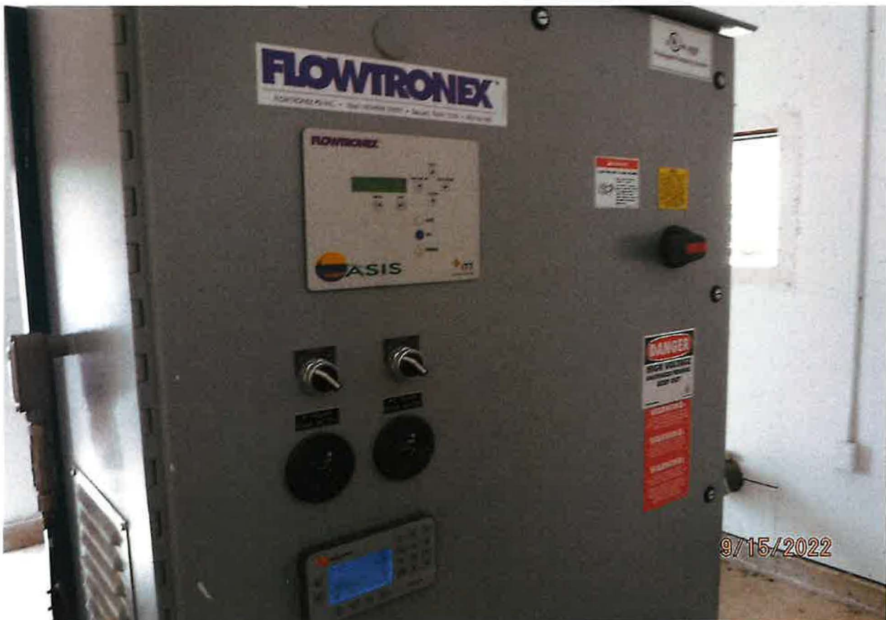
FLOWTRONEX PUMP SYSTEM SCADA CONTROL SYSTEM
