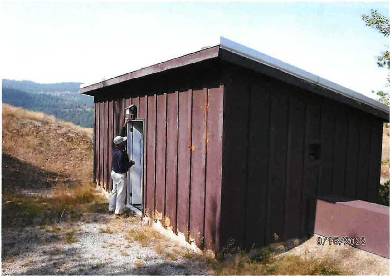
IRRIGATION FROM STORAGE PUMP STATION
