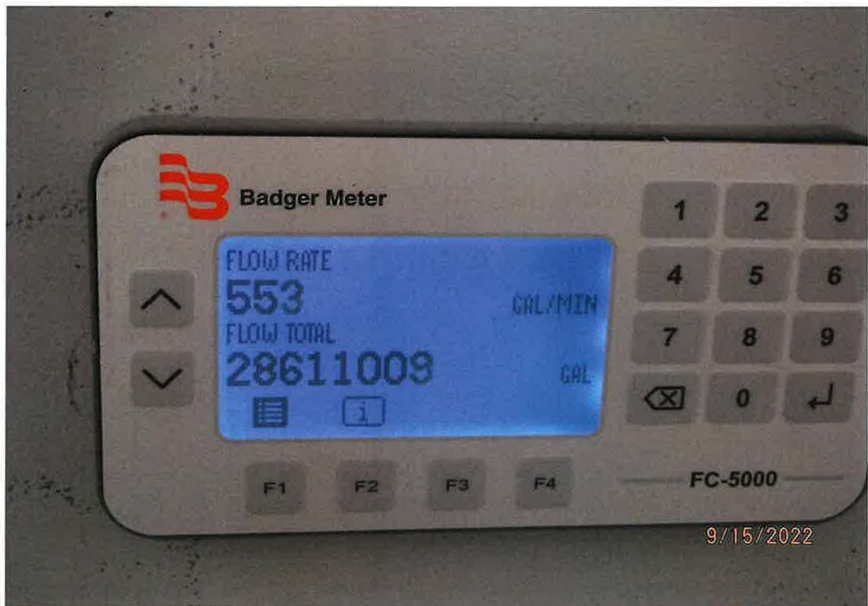
FLOWMETER MEASUREMENT TAKEN FROM EACH PUMP USING BADGER BRAND FLOWMETER
