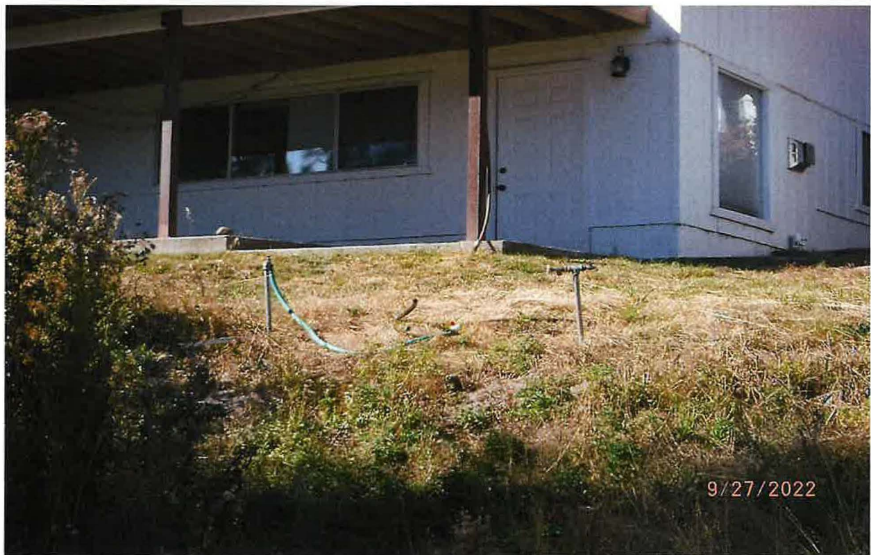
DEDICATED IRRIGATION SYSTEM RISER PIPE(S) WITH HOSE BIB TO HOSE/SPRINKLER USE FOR LTs 7 & 8, BLK 1 (RP070800010070 & RP070800010080) LOCATED AT 7378 W SANDERS RD
