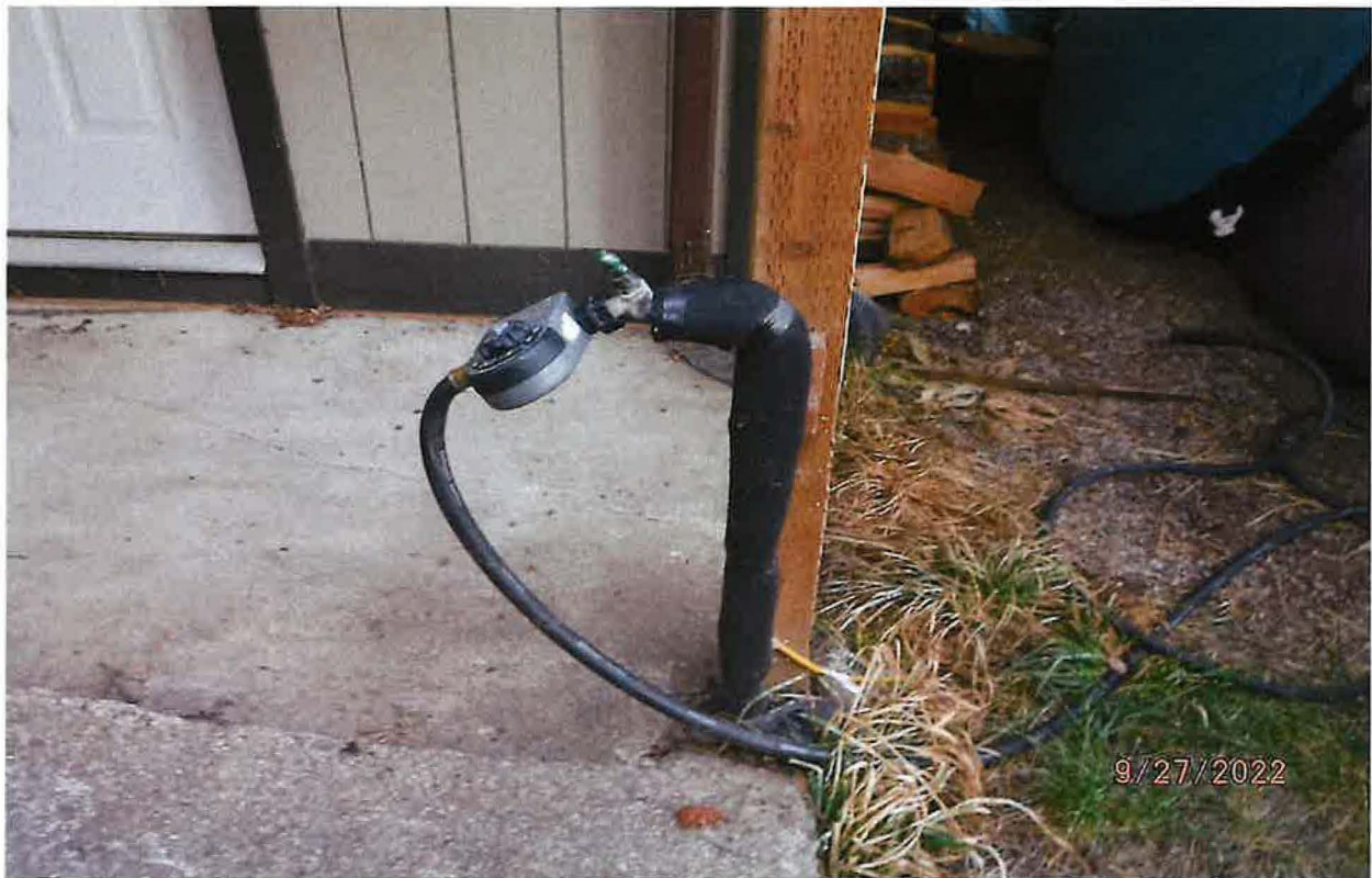
DEDICATED IRRIGATION SYSTEM RISER PIPE WITH HOSE BIB TO HOSE/SPRINKLER USE FOR LT 2, BLK 1 (RP070800010020) LOCATED AT 7262 W SANDERS RD
