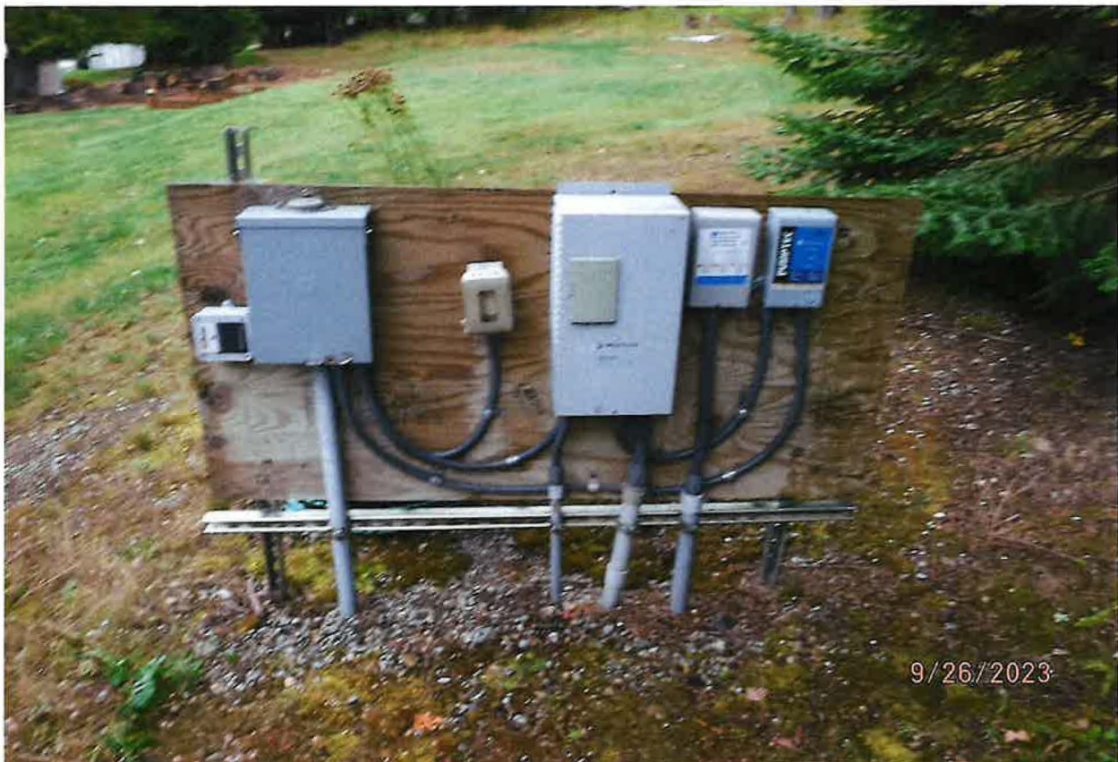
DIVERTING WORKS CONTROL PANEL TREE
