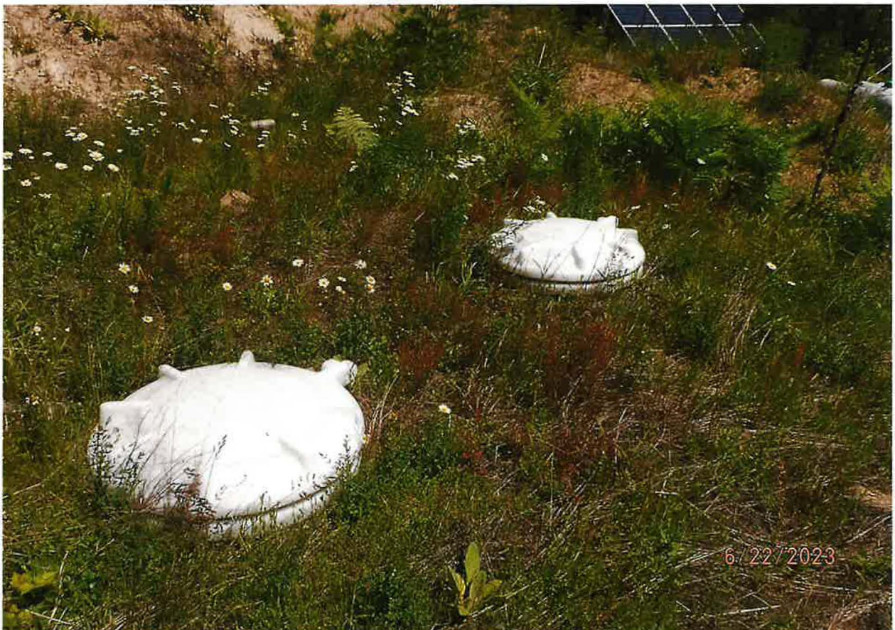
2EA STORAGE RESERVOIRS DEVELOPED IN DOMESTIC SYSTEM
