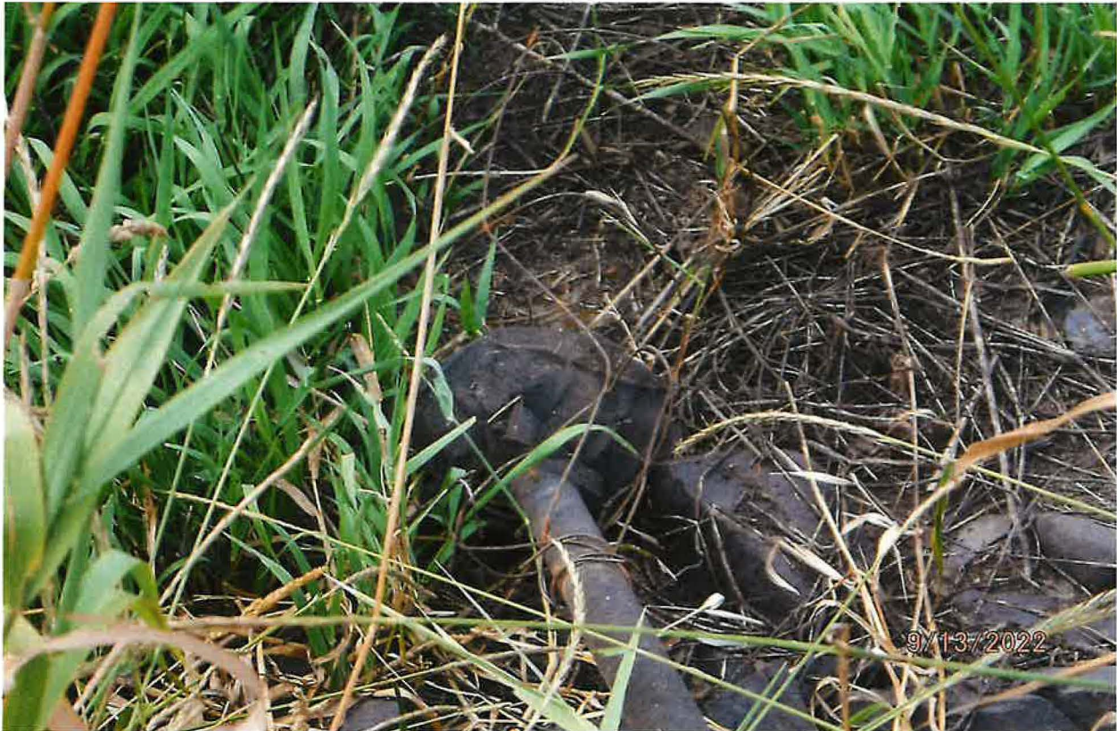
INTAKE PIPE WITH MESH SCREENING – CREEK HAD DRIED UP FOR THIS YEAR BY MID SEPTEMBER
