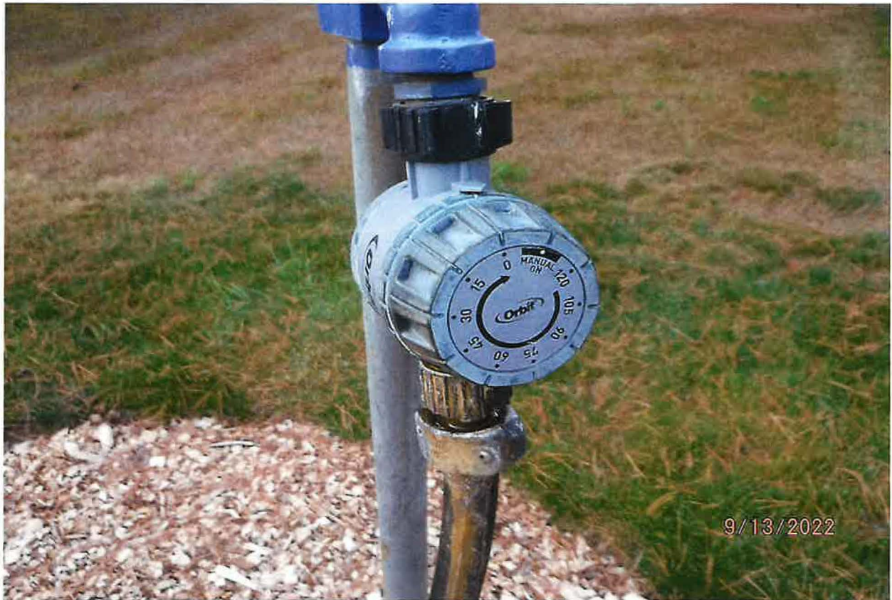
HOSE AND SPRINKLER ON TIMERS FOR IRRIGATION
