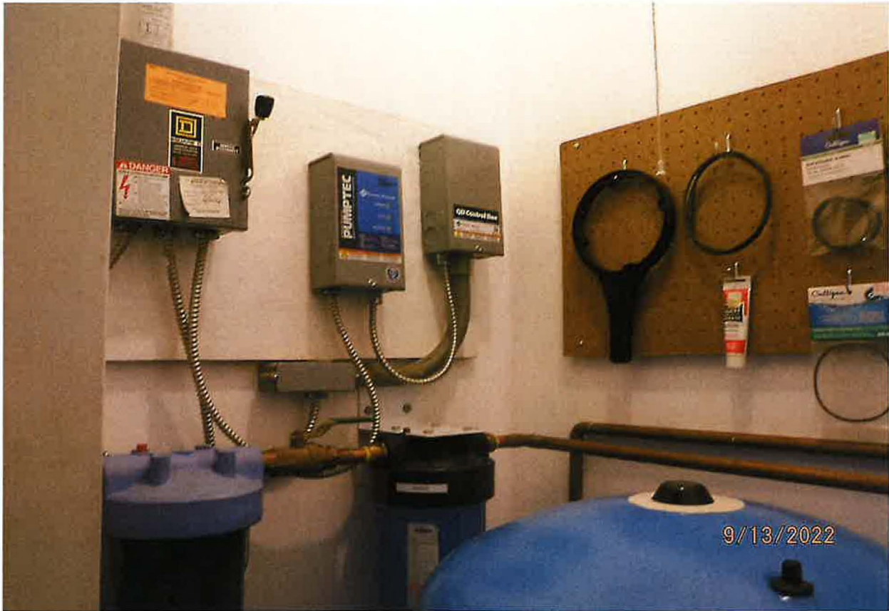
WATER SYSTEM INFRASTRUCTURE
