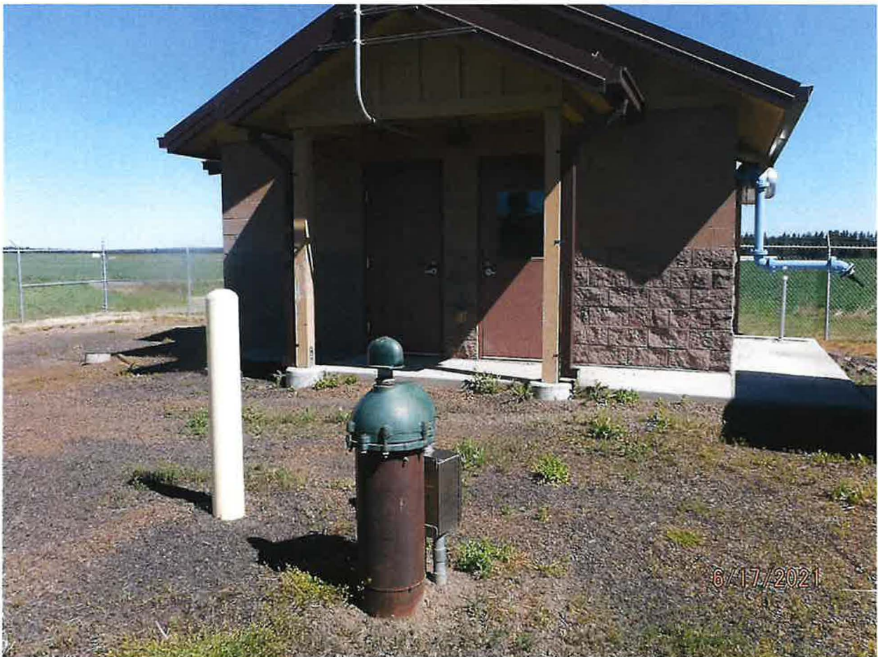
POD – WELL No.13 WITH 15 HP 10-STAGE PUMP/MOTOR INSTALLED
