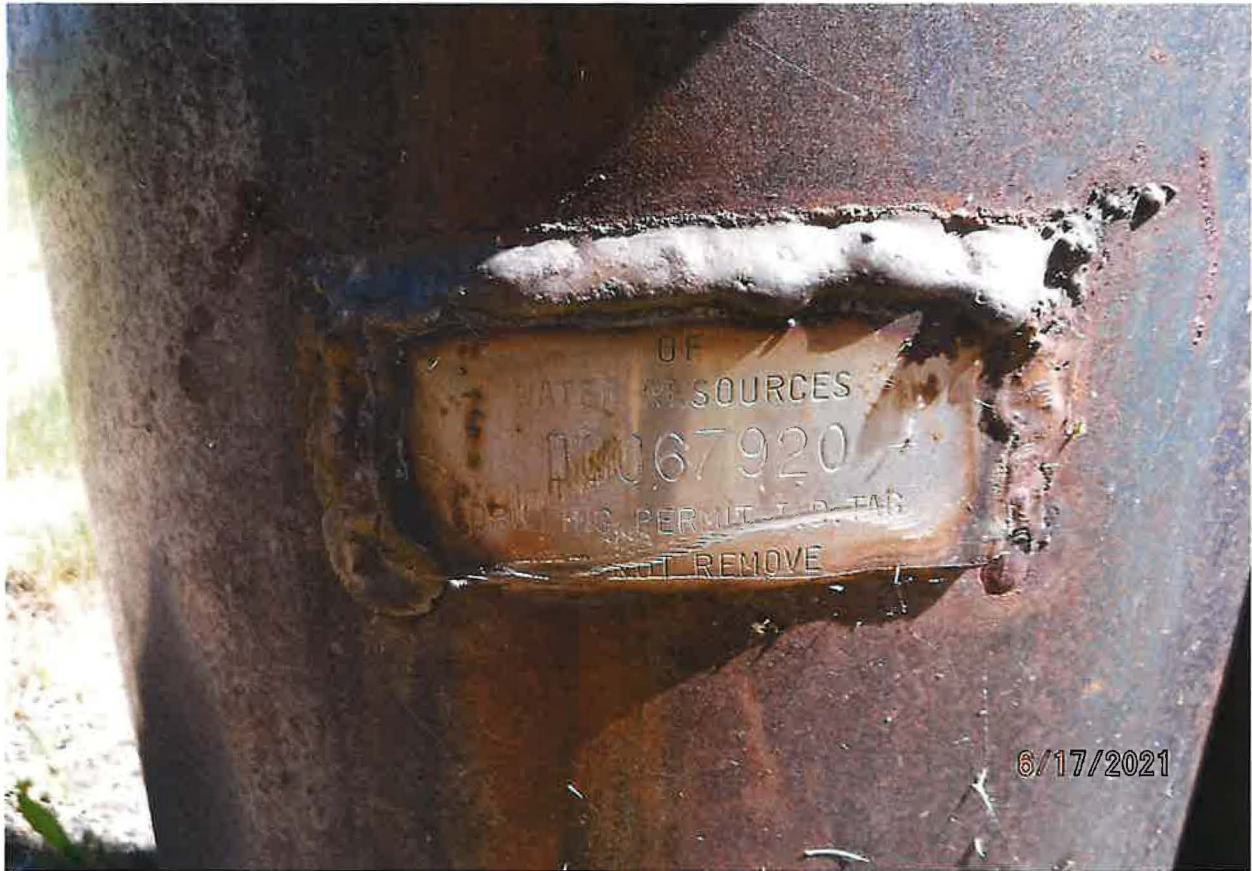
POD – WELL No.15 D-TAG DOO67920 WITH 15 HP 12 STAGE PUMP/MOTOR INSTALLED
