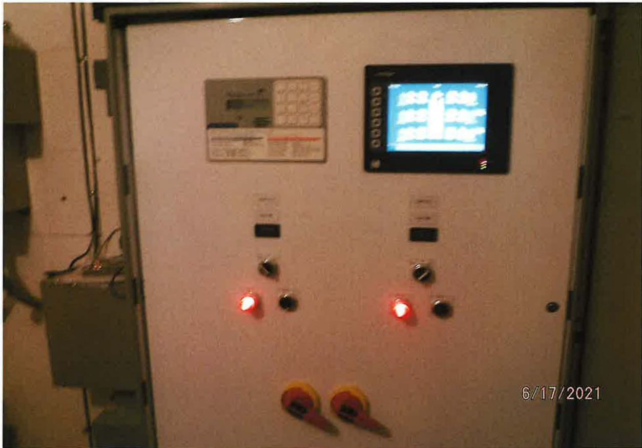
PUMP STATION WELL No.6 & No.7 CONTROL PANEL
