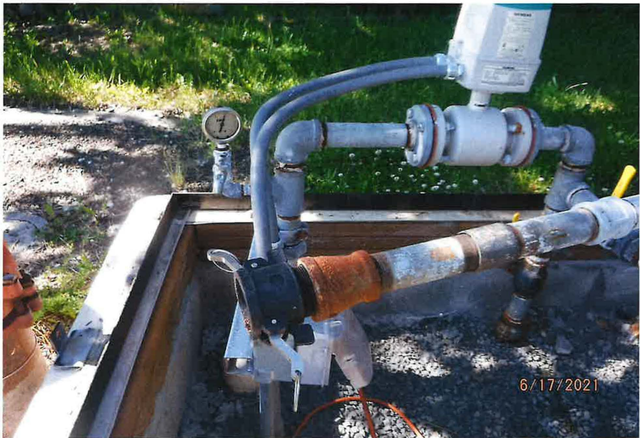
WELL No.4 DIVERTING WORKS WITH SIEMENS FLOWMETER INSTALLED
