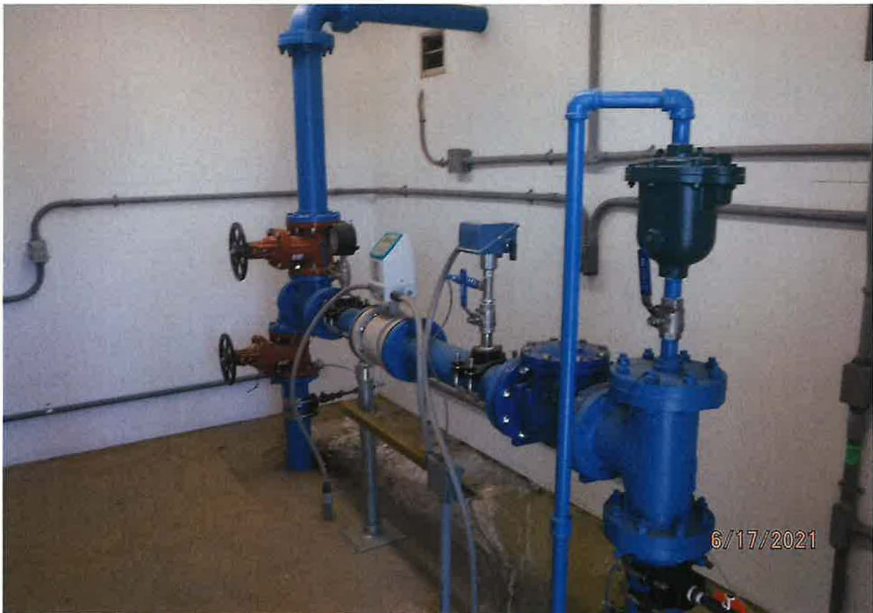
WELL No.13 PUMP STATION WITH DIVERTING WORKS
