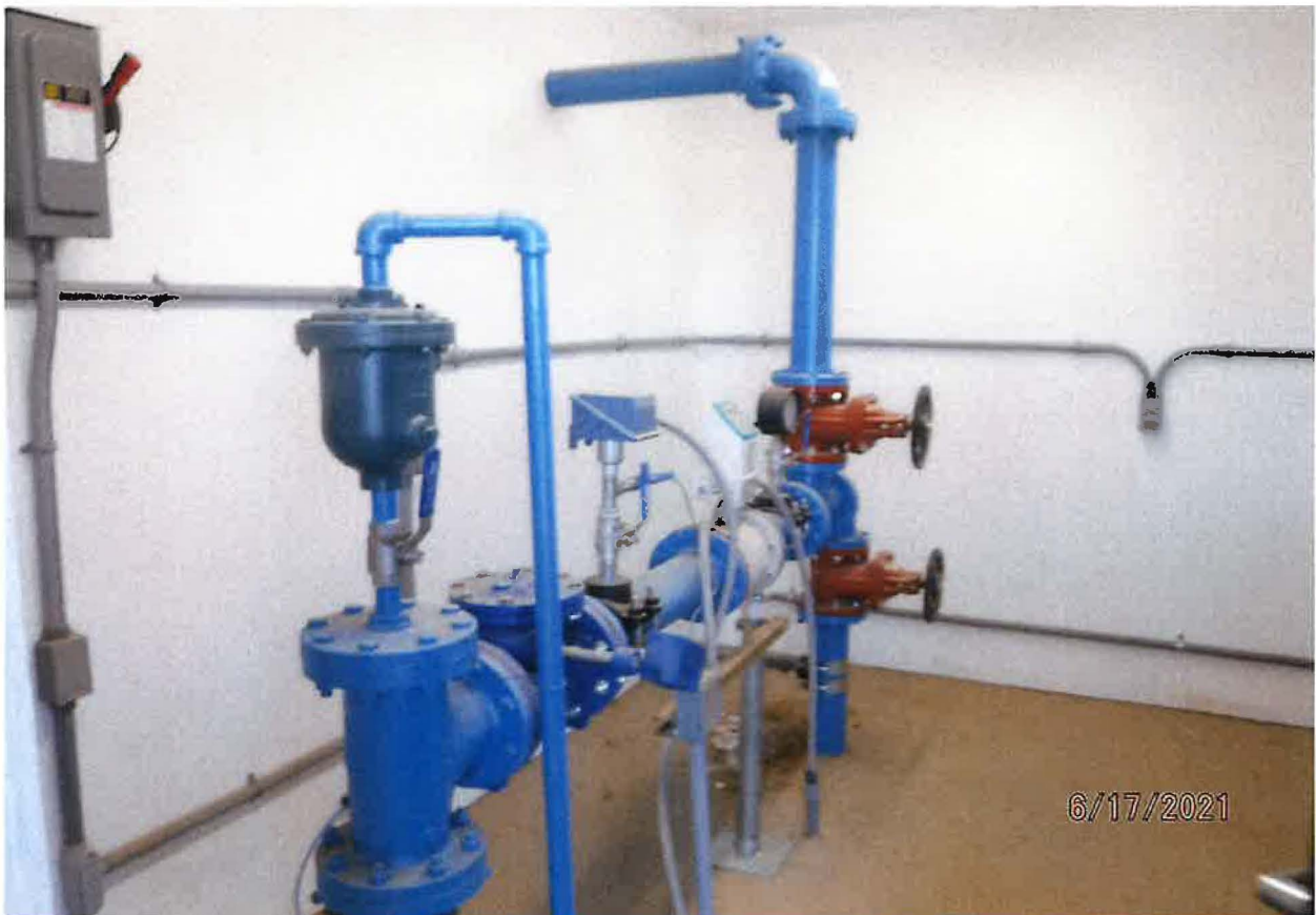
WELL No.15 PUMP STATION AND DIVERTING WORKS
