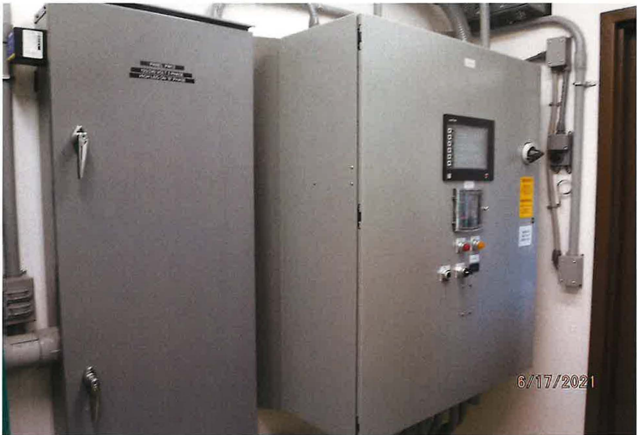
WELL No.13 CONTROL PANEL AND SCADA SYSTEM CONTROL PANEL
