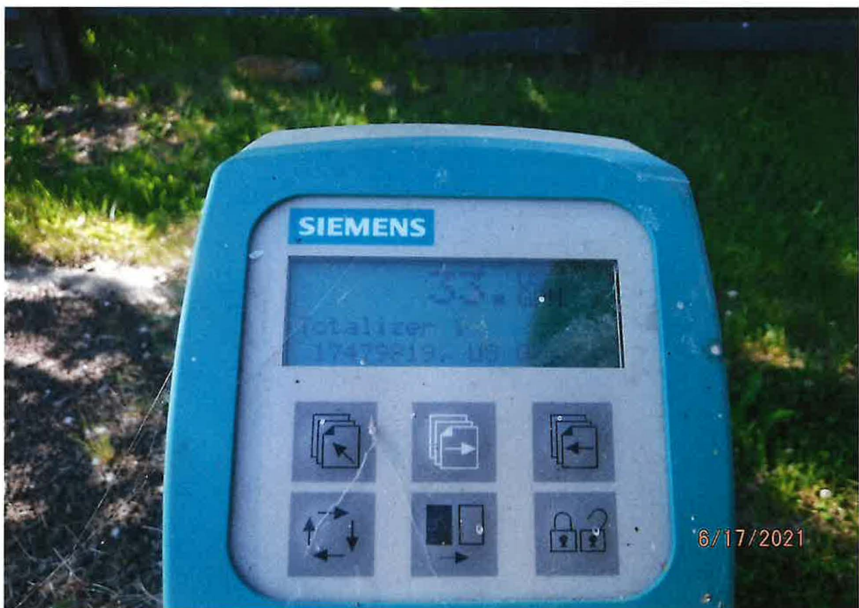
WELL No.4 - SITRANS F M MAG 5100 W FLOWMETER, S/N 7ME658 02621U463
