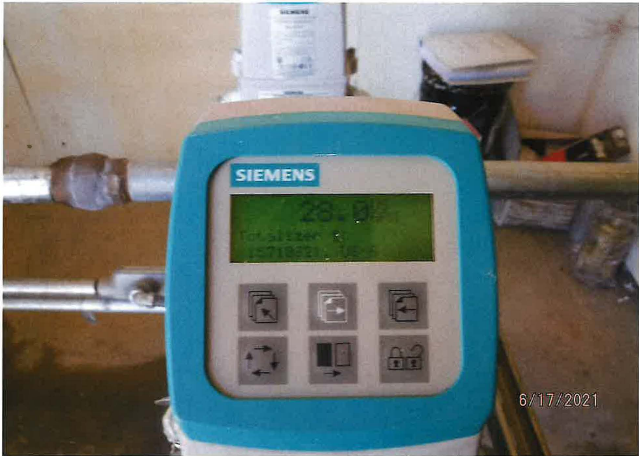
WELL No.4 - SITRANS F M MAG 5100 W FLOWMETER, S/N 7ME658 415001U293
