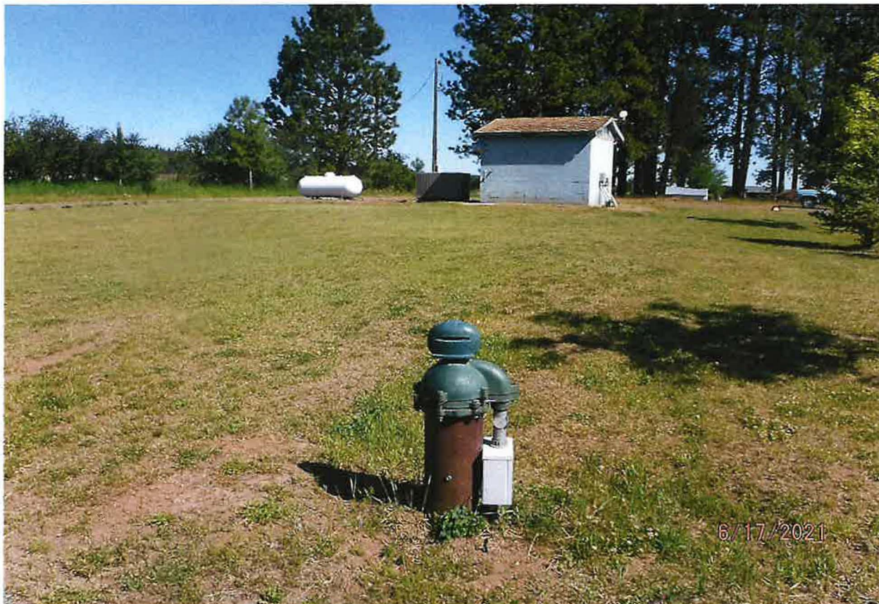
POD – WELL No.6, WITH DEQ TAG E0008546; UNKOWN PUMP HP INSTALLED IN WELL
