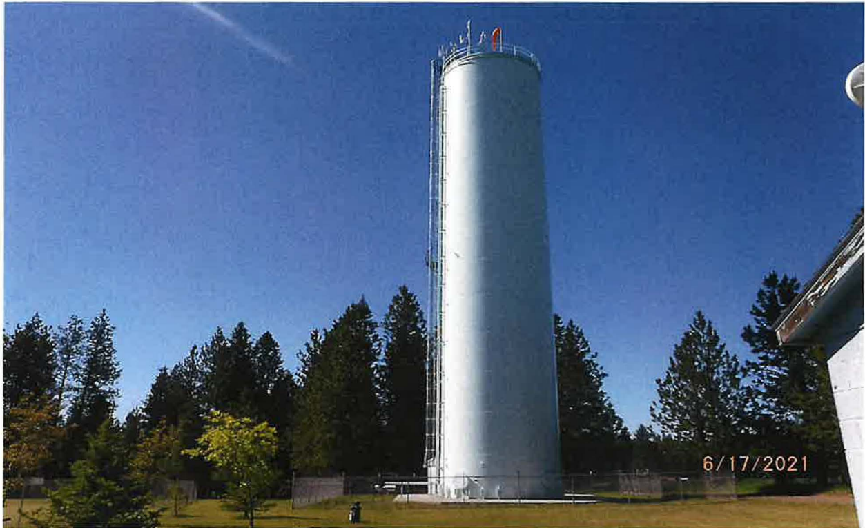
400,000-GAL STORAGE TANK, CO-LOCATED WITH WELL No.6 & No.7 WITH PUMP HOUSE
