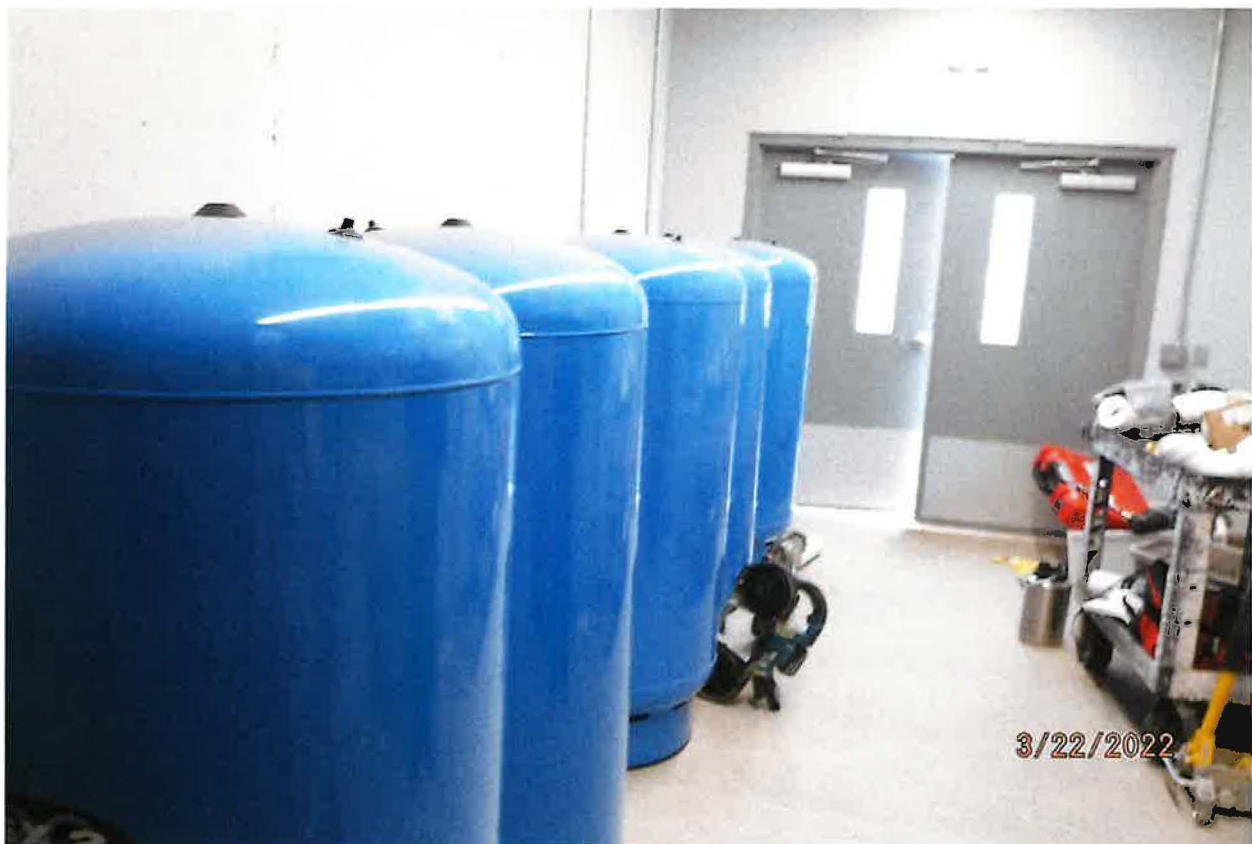
5EA PRESSURE TANKS INSTALLED IN SYSTEM
