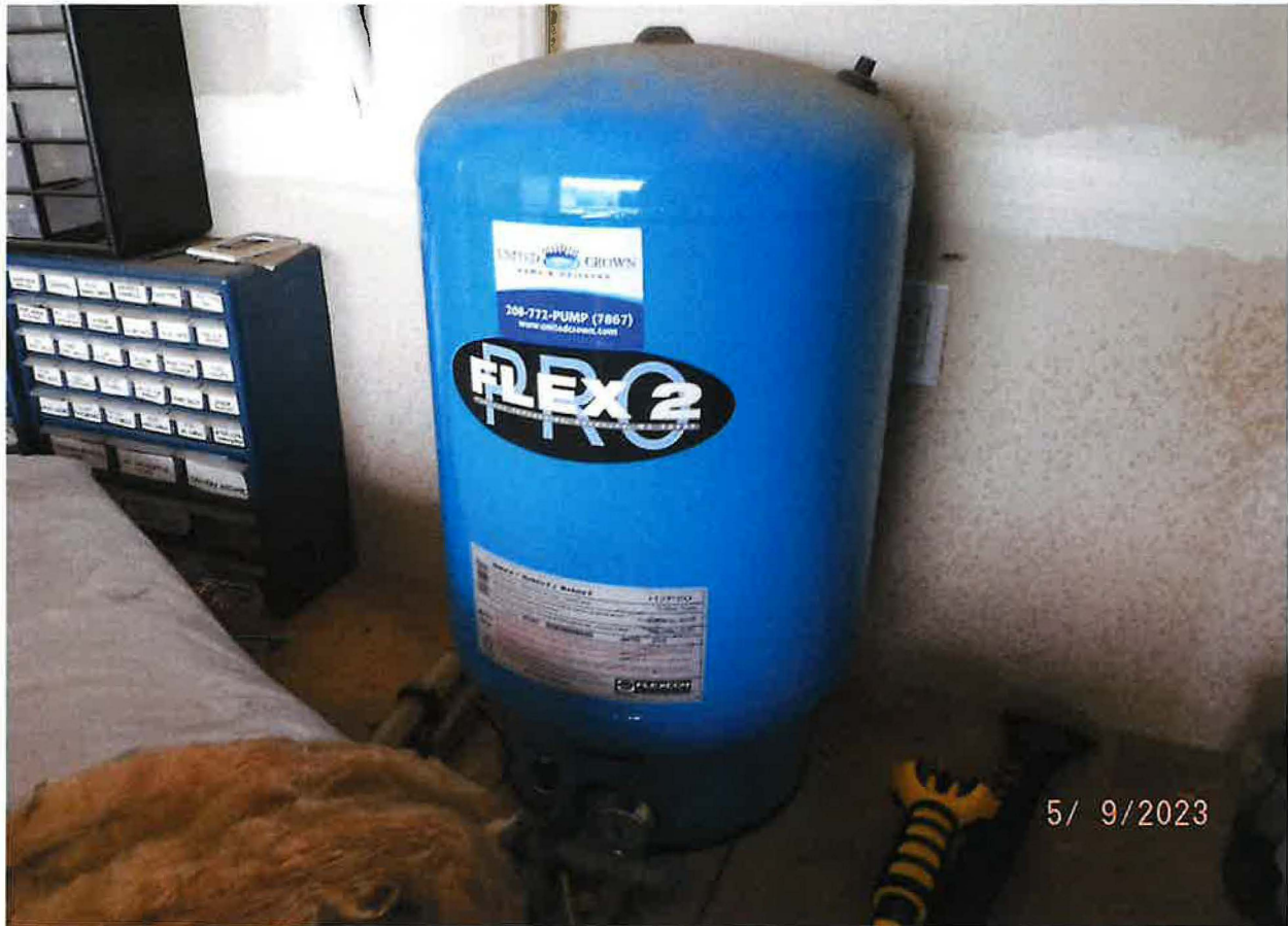
WATER SYSTEM PUMPS DIRECT TO PRESSURE TANK PRIOR TO DISTRIBUTION TO BENEFICIAL USES
