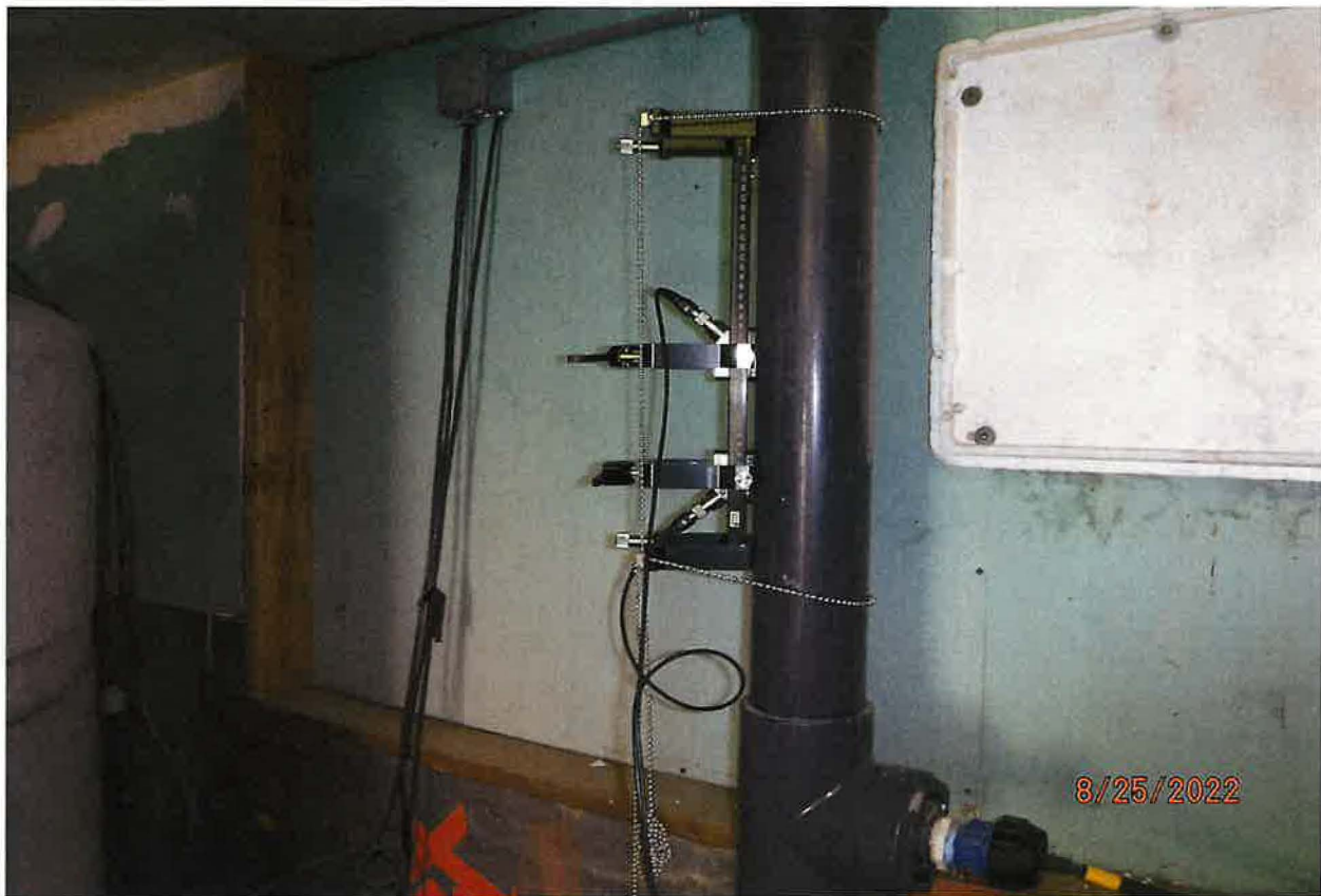
FLOW METER MEASUREMENT
