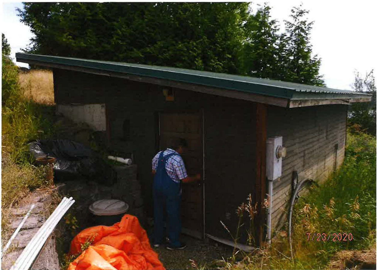
PUMP HOUSE ELEVATED ON BENCH ABOVE POD
