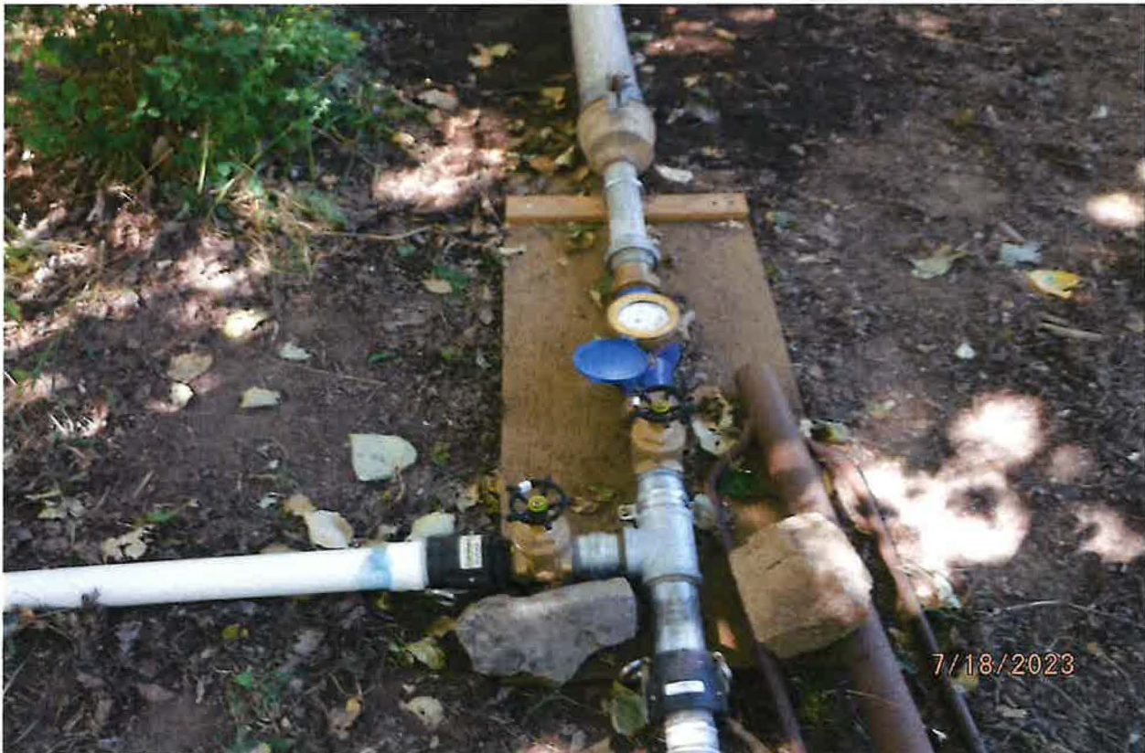
DIVERTING WORKS INCLUDE 2" PUMP DISCHARGE TO 5" IRRIGATION MAIN TRUNK TO 3" HAND LINE
