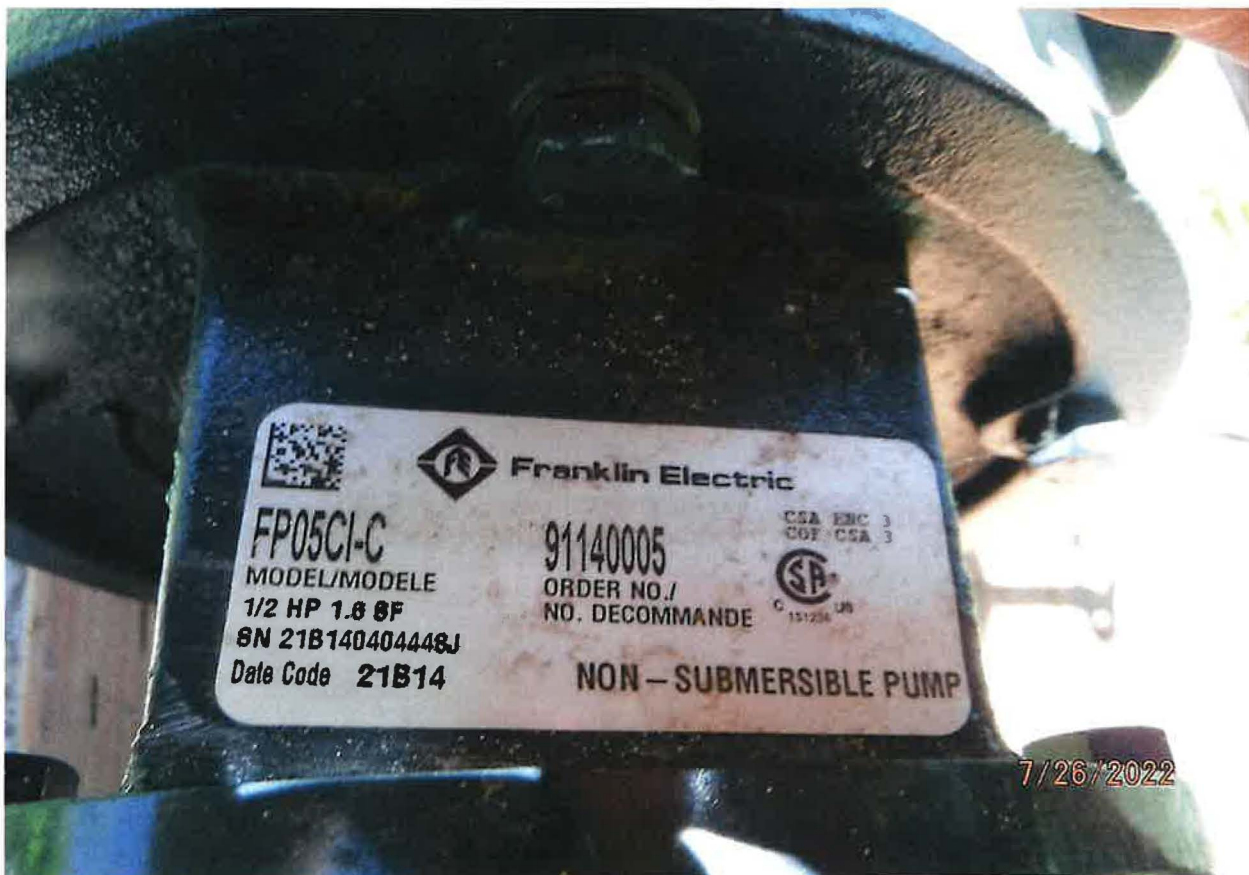
FRANKLIN ELECTRIC ½ HP PUMP MOTOR PAIRED WITH U.S. MOTORS JET PUMP AT POD
