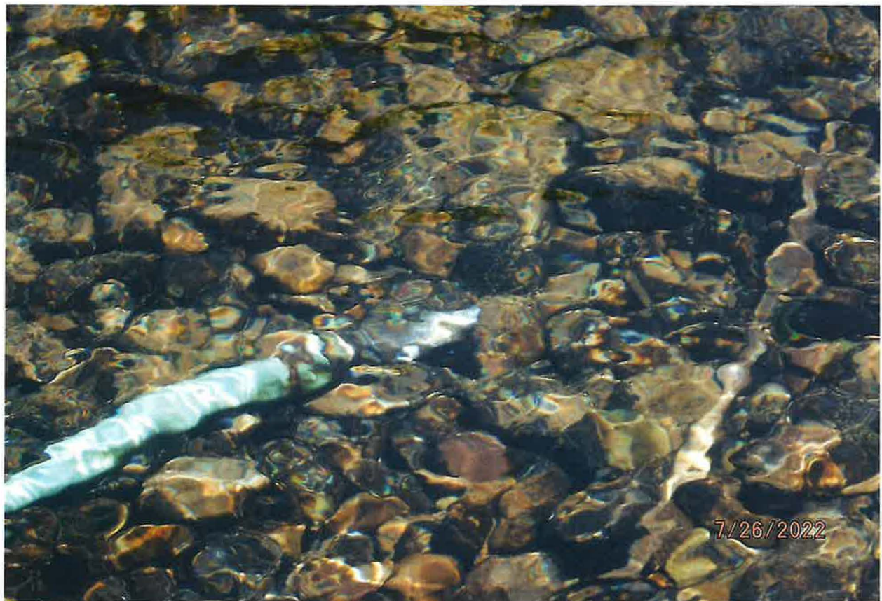
BOTH POD PIPES HAVE A SCREEN INSTALLED ON THE INTAKE IN RIVER
