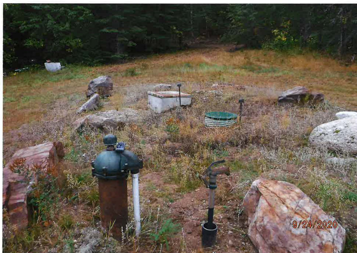
3,000 GAL STORAGE TANK LOCATED IN NE¼NW¼
