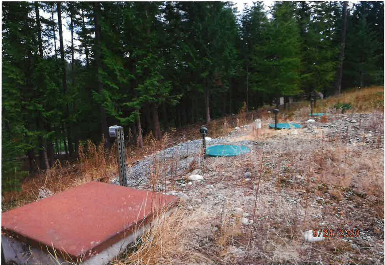
9,000 GALLON STORAGE RESERVOIR – CO-MINGLES WATER FROM 4EA WELLS
