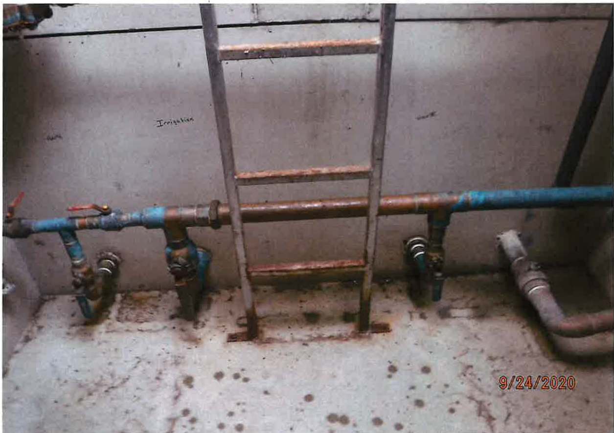
VAULTED 9,000 GALLON STORAGE RESERVOIR WATER WORKS
