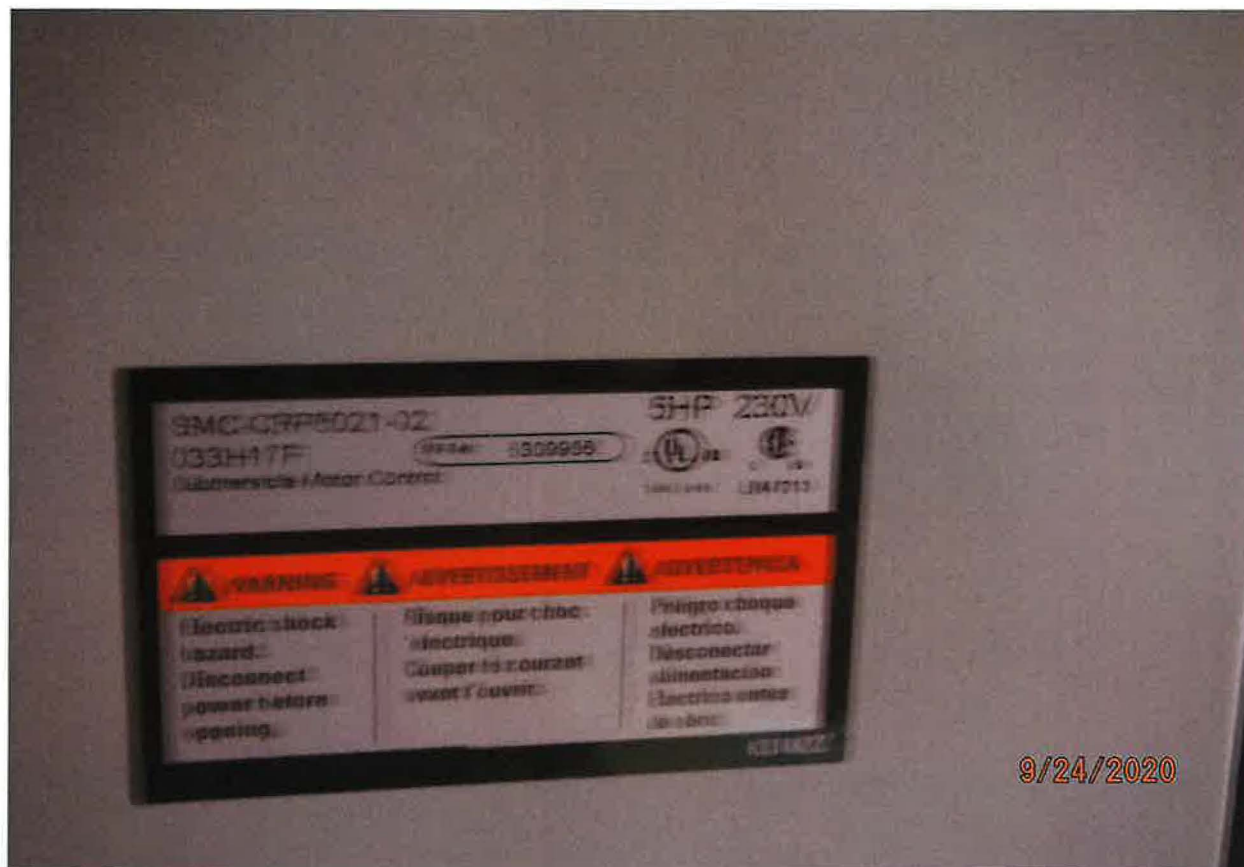
5 HP PUMP IN WELL WITHOUT TAG
