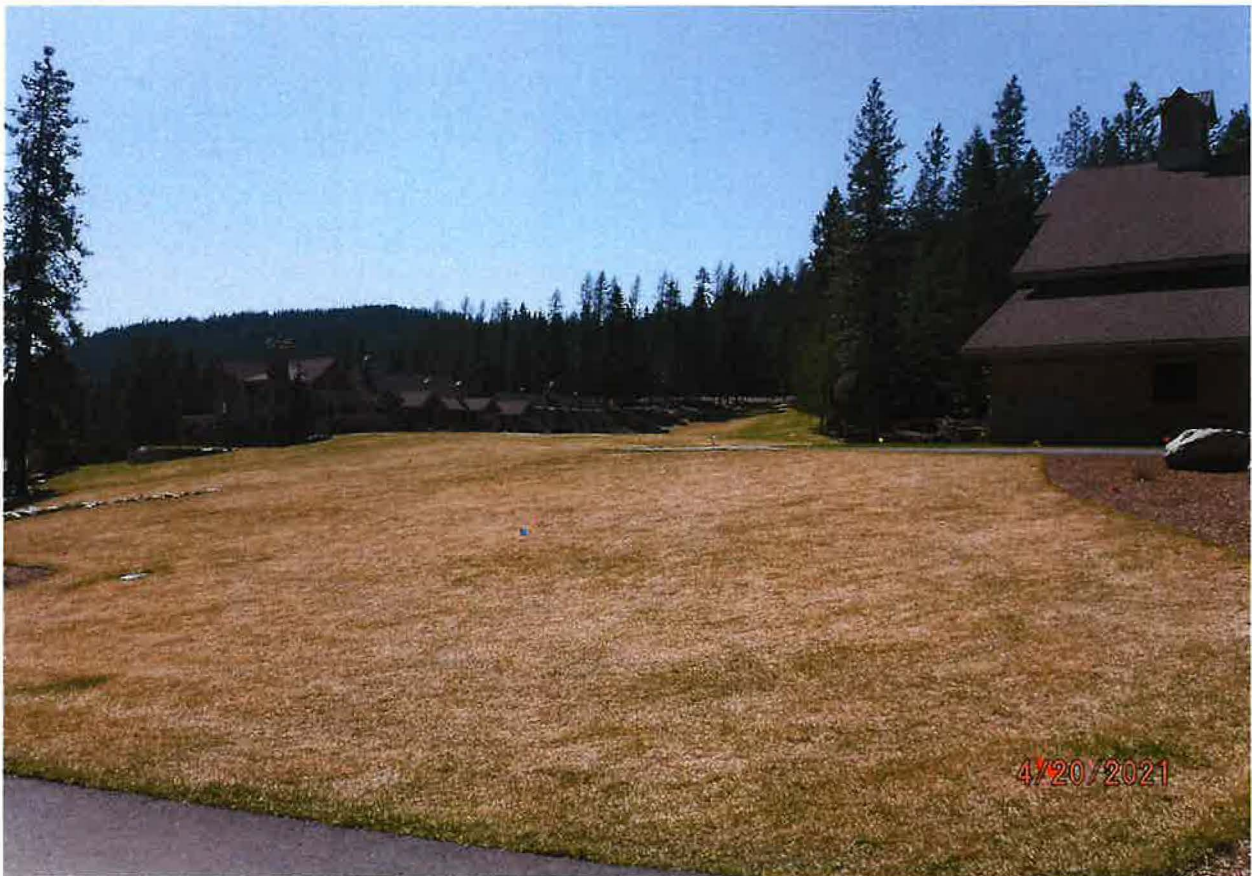
IRRIGATION POU – PRESSURIZED SPRINKLER HEADS FLAGGED
