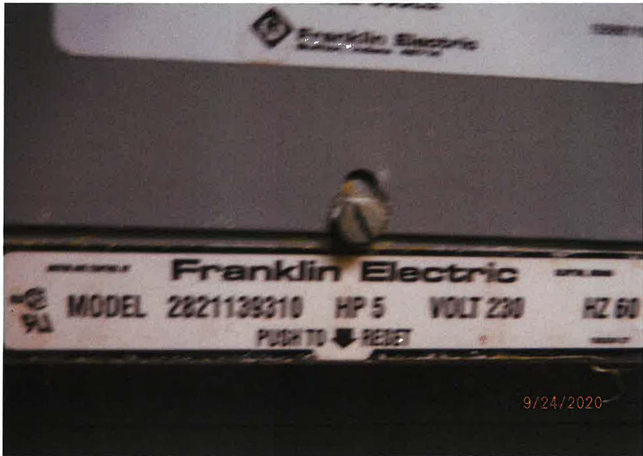
5 HP PUMP IN WELL D0054541
