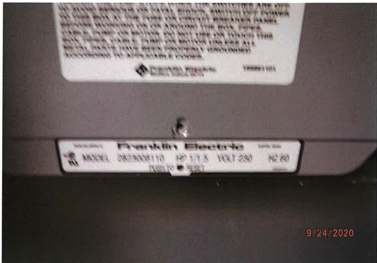
1.5 HP PUMP IN WELL 96-91-N-69
