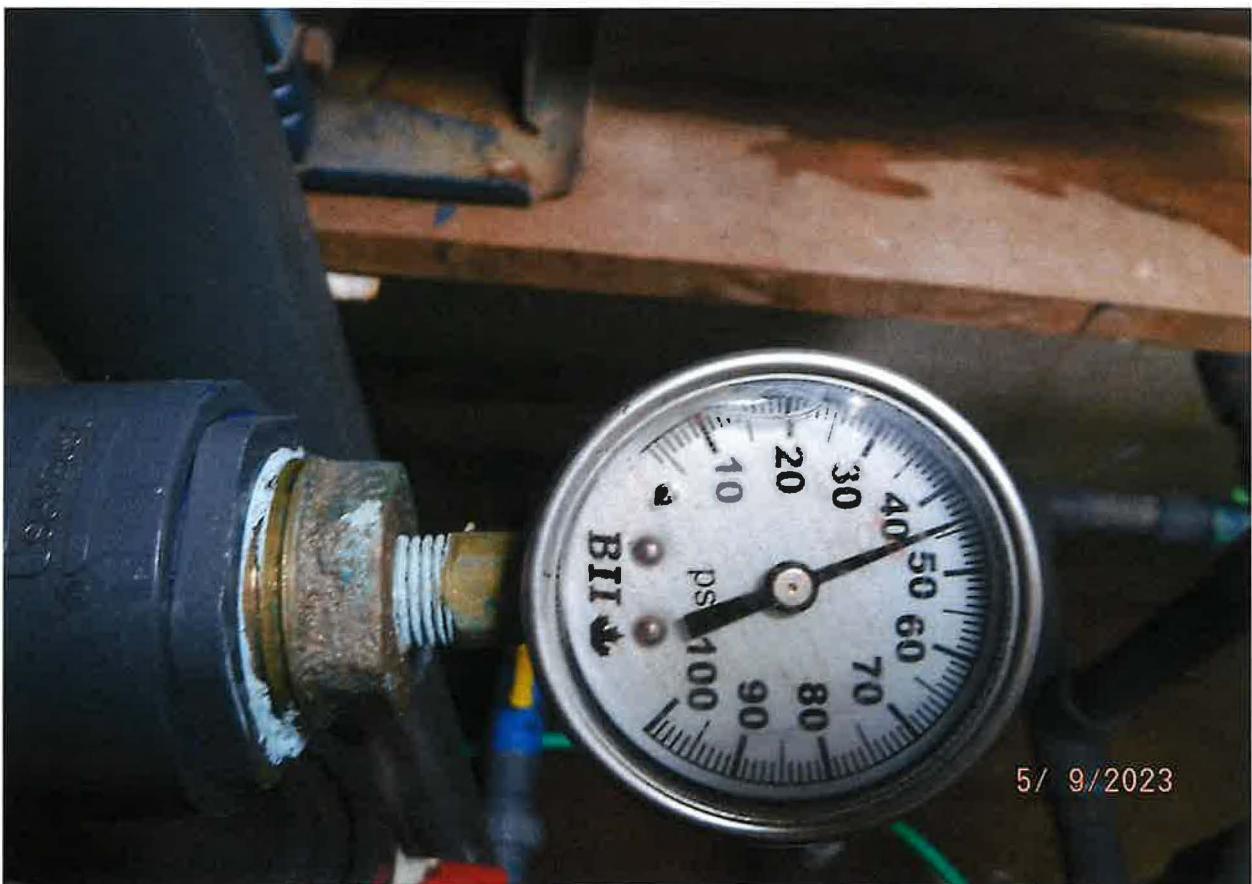
45 PSI WATER SYSTEM OPERATING PRESSURE
