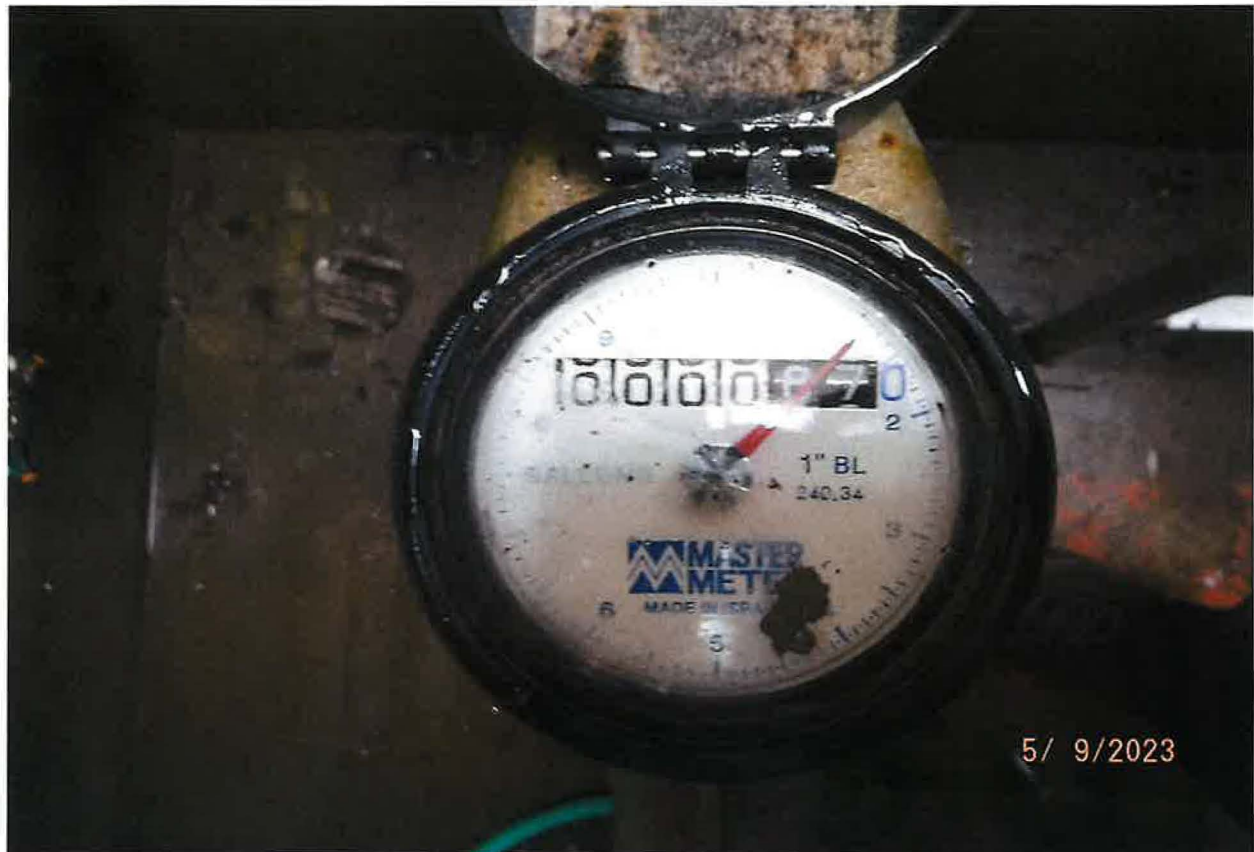
EXAMPLE – 1 OF 4 FLOWMETERS INSTALLED IN SYSTEM – MASTER METER
