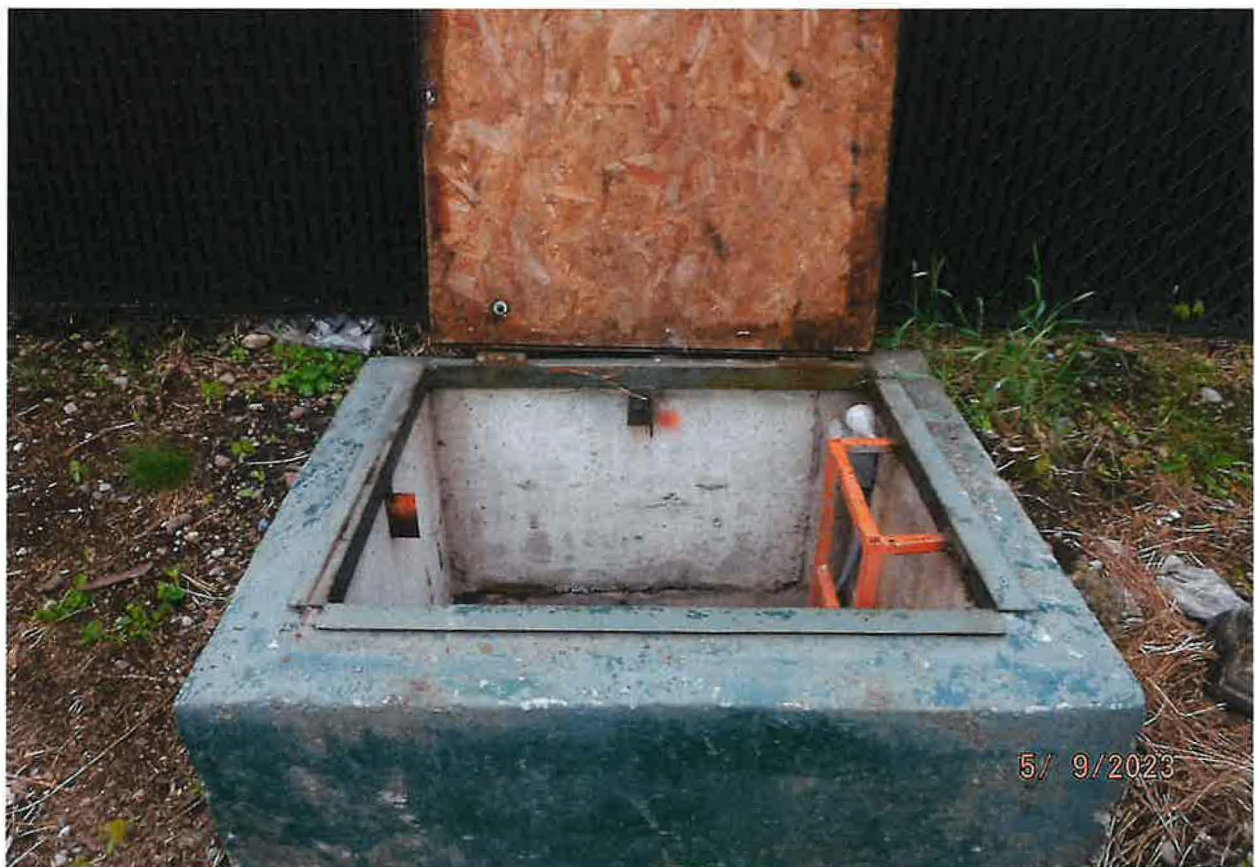
WATER SYSTEM DIVERTING WORKS LOCATED IN VAULT CO-LOCATED WITH WELL
