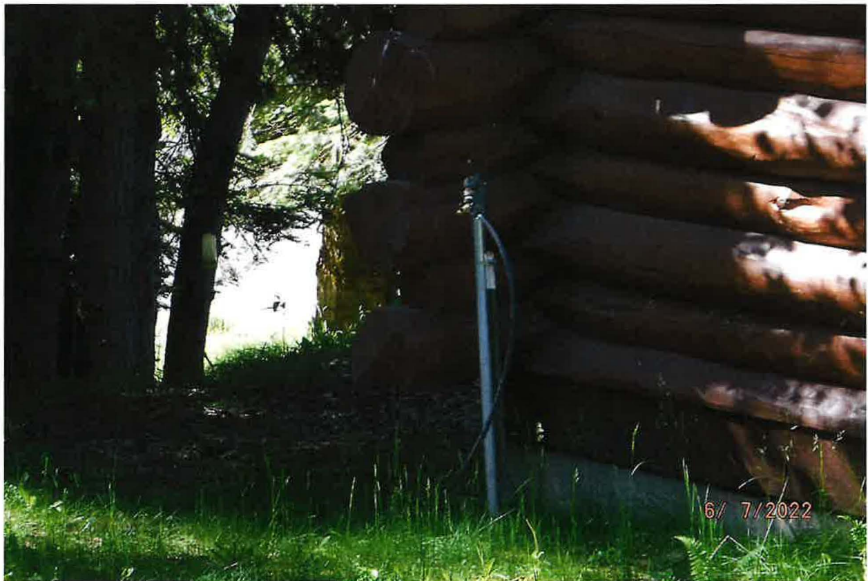
IRRIGATION POU – HOSE AND SPRINKLERS FROM FROST-FREE HYDRANT
