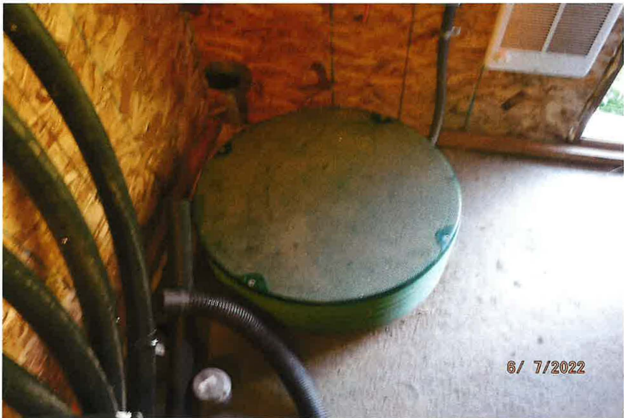
VAULTED 1,500 GAL CISTERN – LID LOCATED WITHIN PUMP HOUSE
