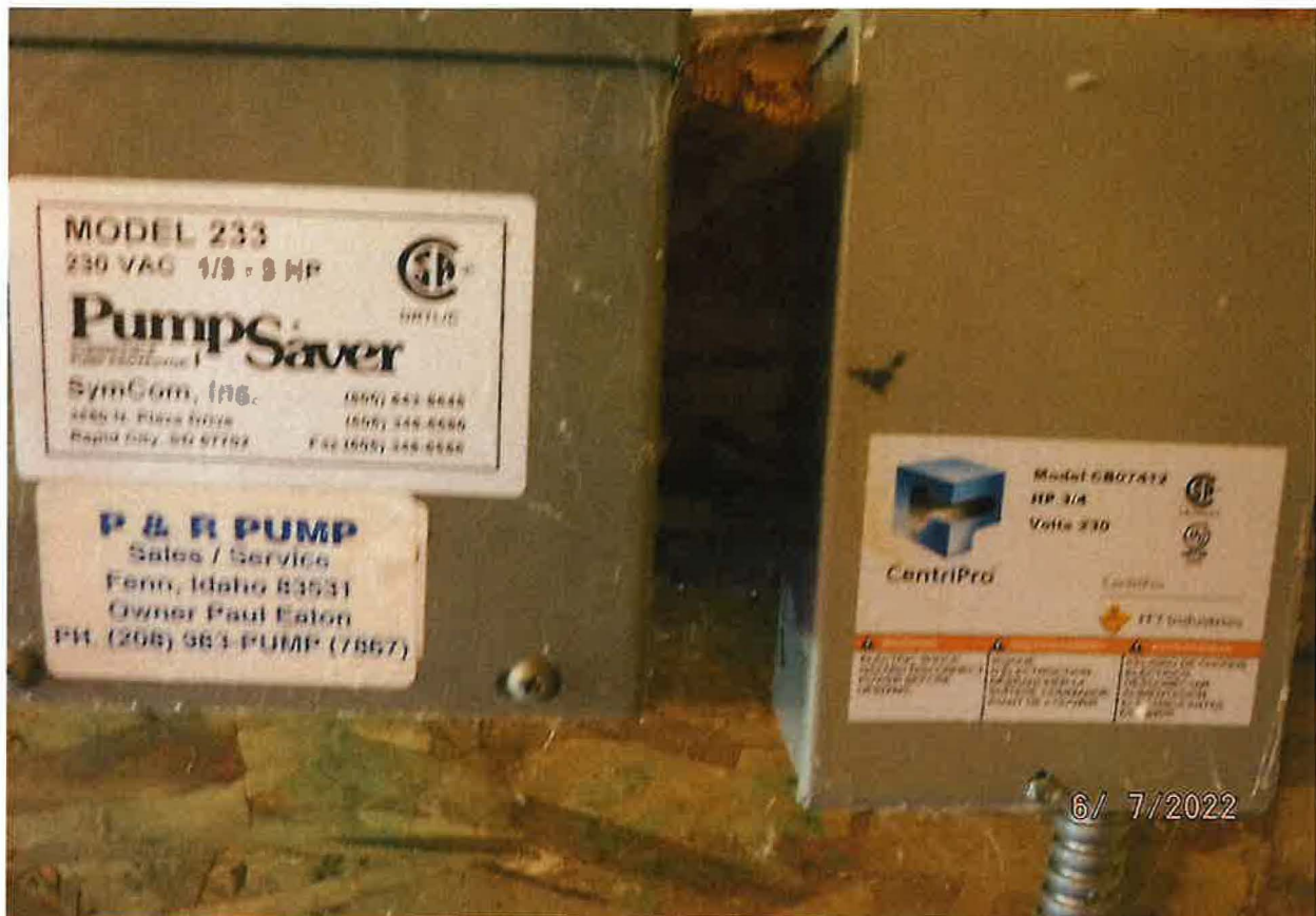
TWO EACH TRANSFER PUMP CONTROL PANELS
