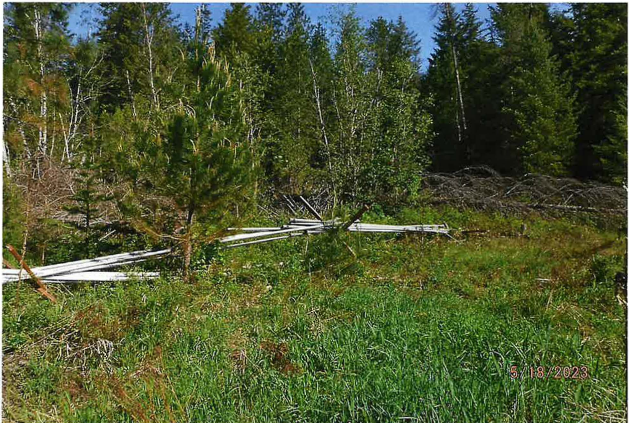
IRRIGATION FROM STORAGE – SPRINKLER HAND LINE USED FOR IRRIGATION SYSTEM
