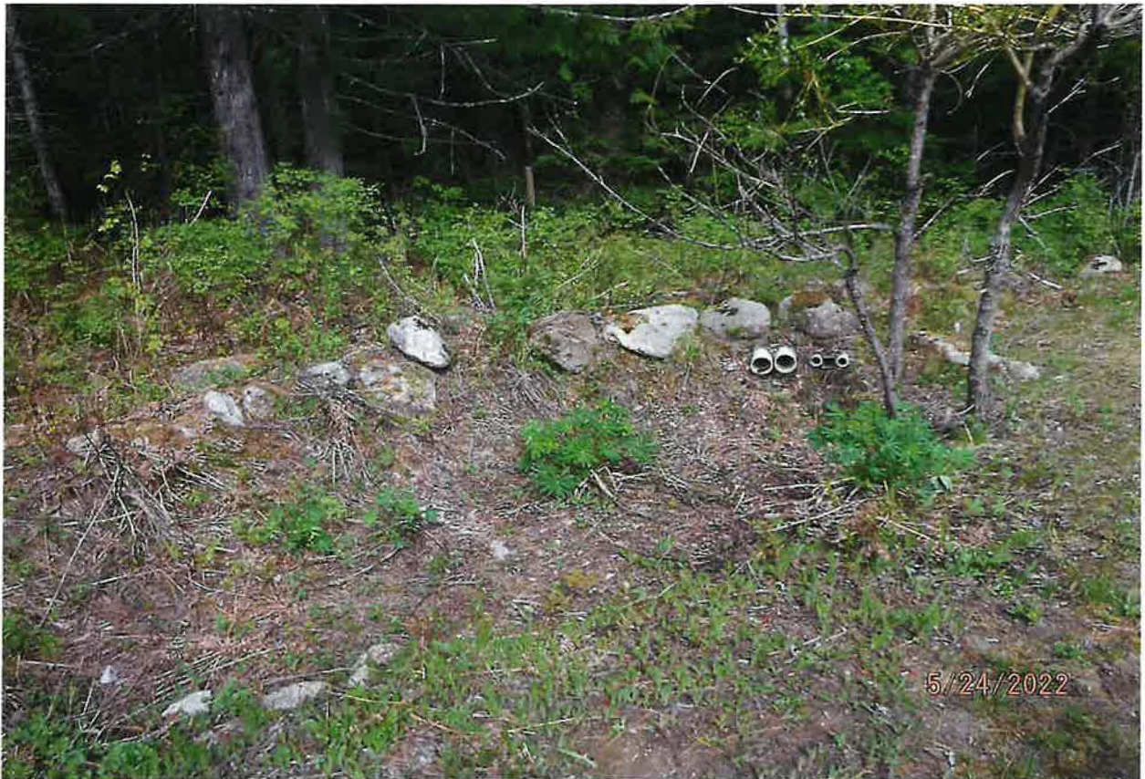
SMALL OVERFLOW BASIN WITH PIPES THAT ROUTE OVERFLOW DOWNSLOPE BACK TO CREEK
