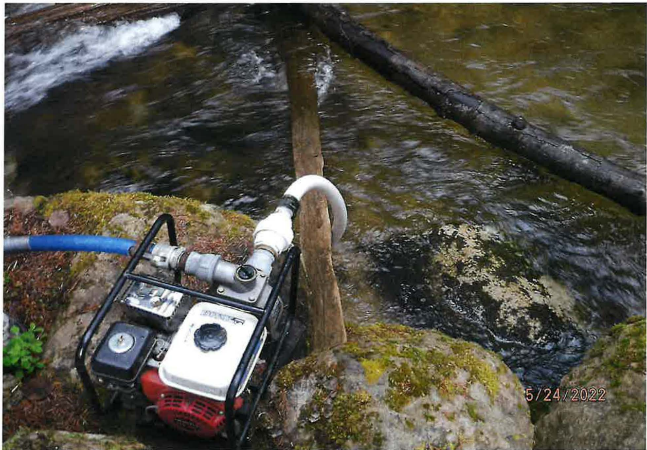
POD – WATER TRANSFER PUMP WITH INTAKE PIPE IN CREEK
