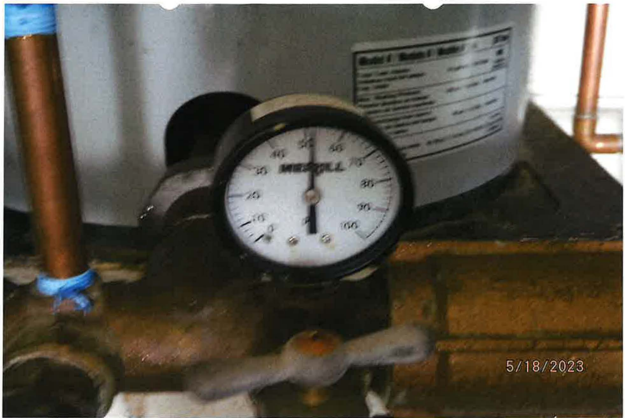
50 PSI WATER SYSTEM OPERATING PRESSURE
