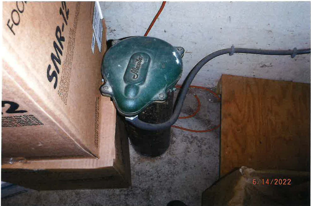
POD – GW WELL (PRE 1987 CONSTRUCTION DATE) – LOCATED WITHIN THE MOOSE KNUCKLE RESTAURANT COMMERCIAL BUILDING, IN THE OFFICE ROOM
