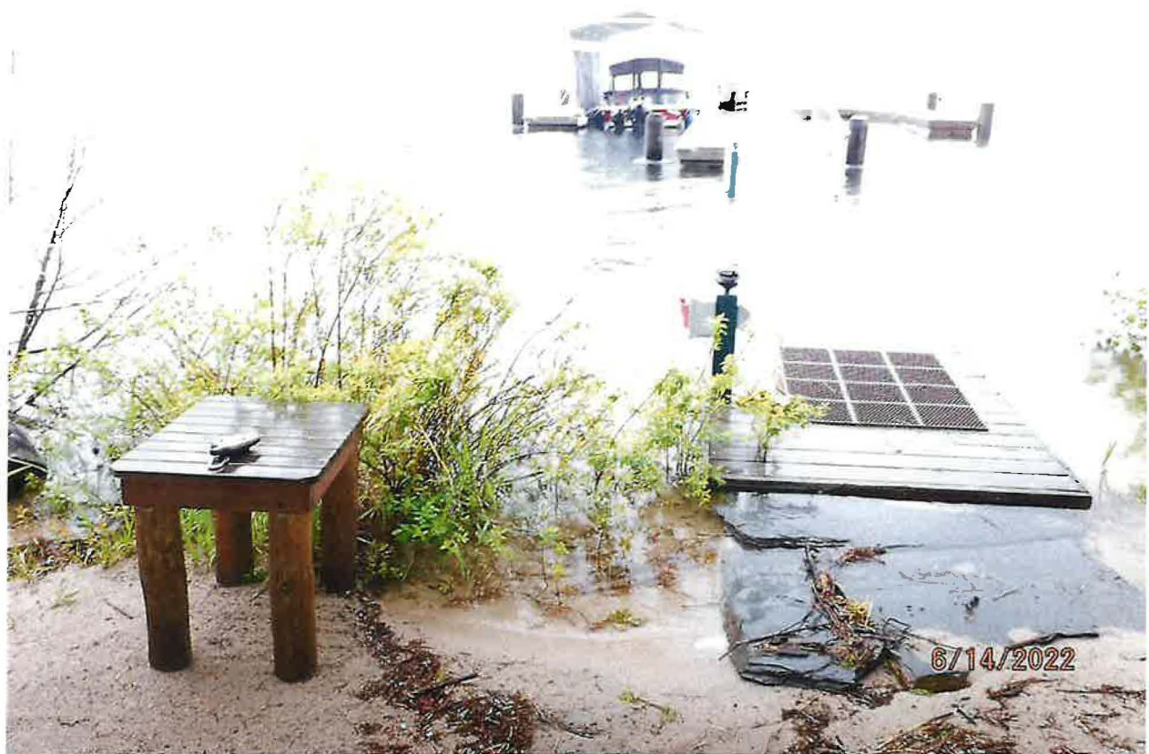
POD – BURIED POLY INTAKE PIPE WITH PUMP AND SCREEN IN LAKE
