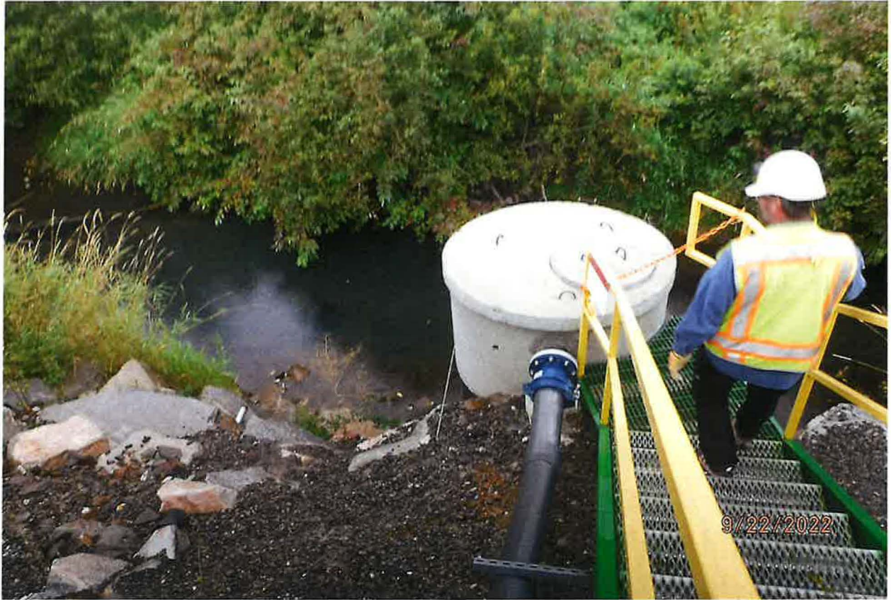
POD – PUMP ENCASED IN CONCRETE RINGS AT DEPTH 7 FT BELOW CREEK BED LEVEL
