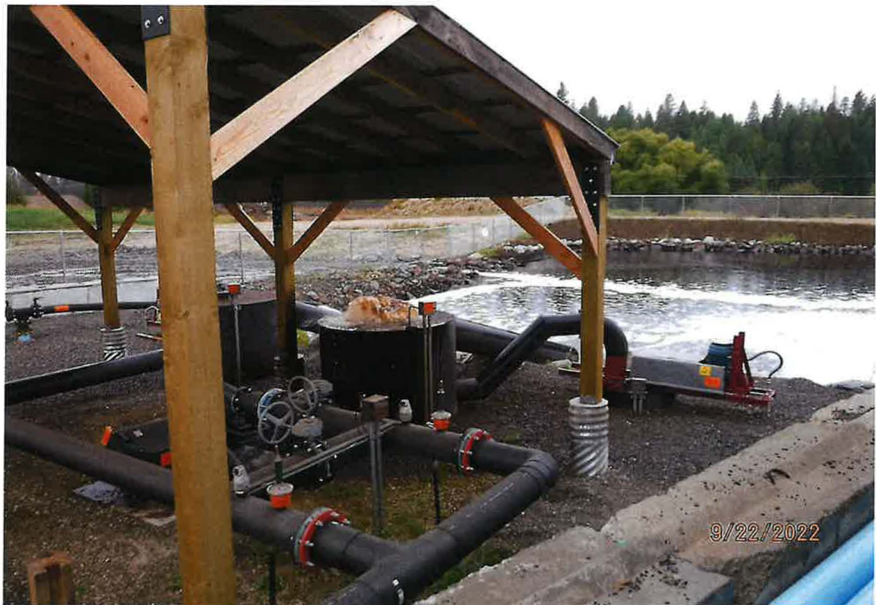
2 PUMP SYSTEMS A RECIRCULATION POND
