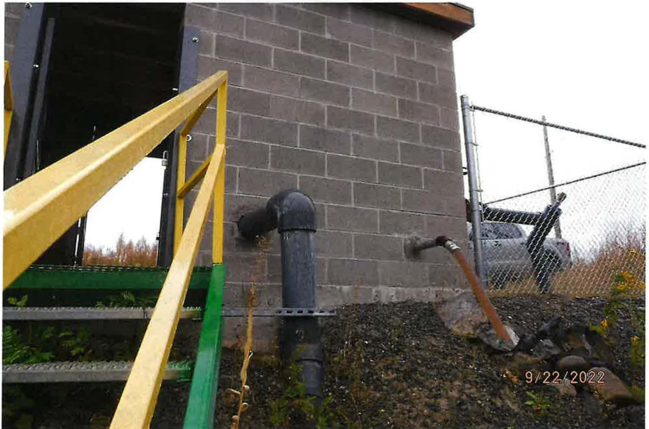
INTAKE PIPE TO PUMP STATION
