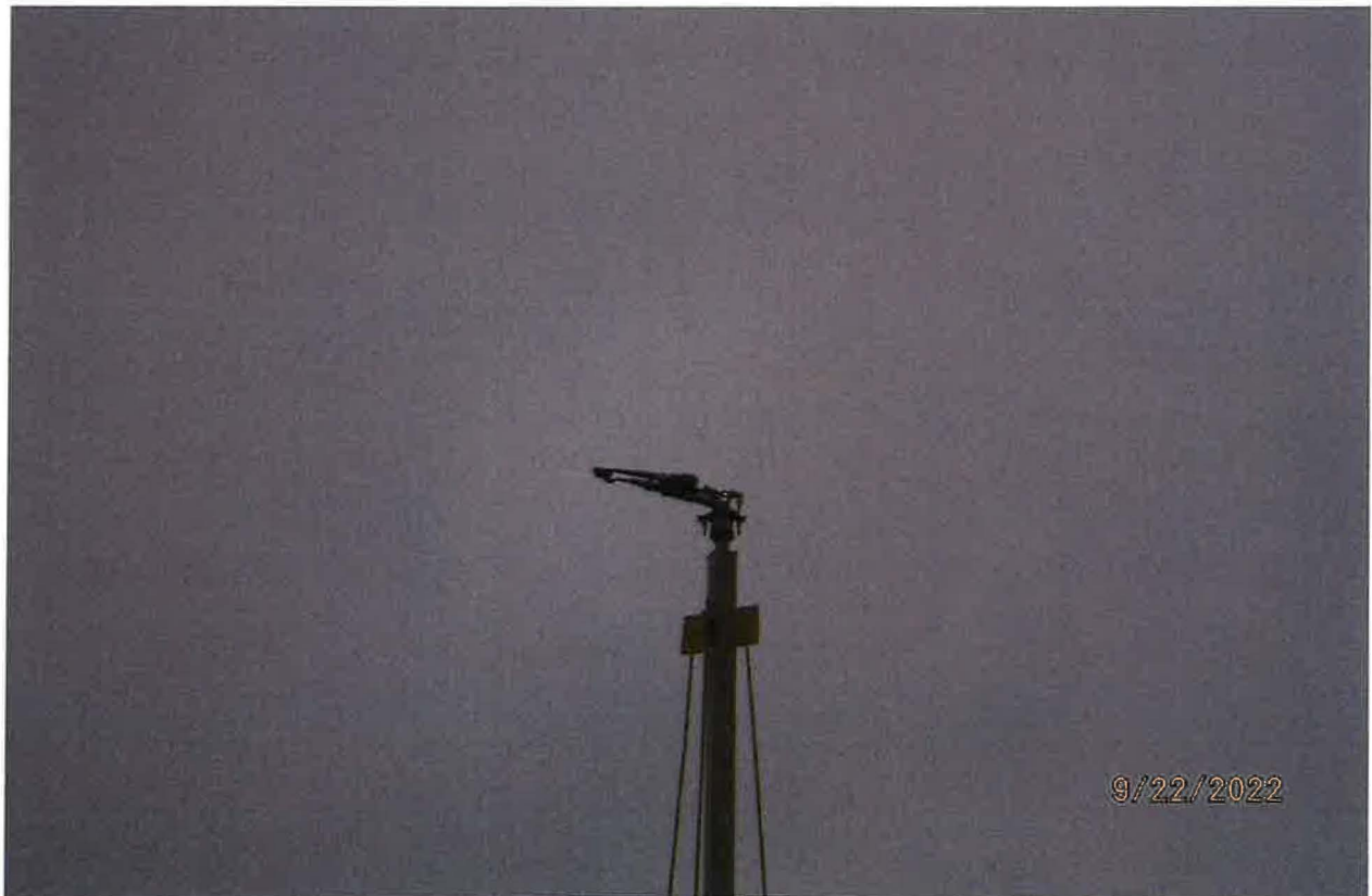
INDUSTRIAL & FP POU – UP TO 13 BIG GUN SPRINKLERS OPERATE OFF RECIRCULATION SYSTEM – 80 PSI 100 GPM PER NOZZLE PROVIDE 150 FT RADIUS FOR LOGWATERING
