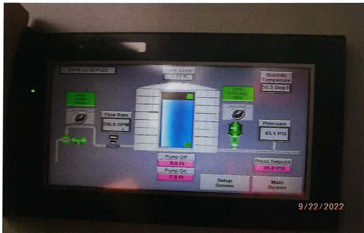
396.5 GPM WAS THE LOWEST FLOW RATE OBSERVED AT TIME OF EXAM
