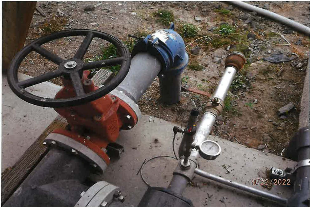
MAIN SERVICE LINE FROM STORAGE TANK TO USES & FIRE PROTECTION HOSE FILL POINT
