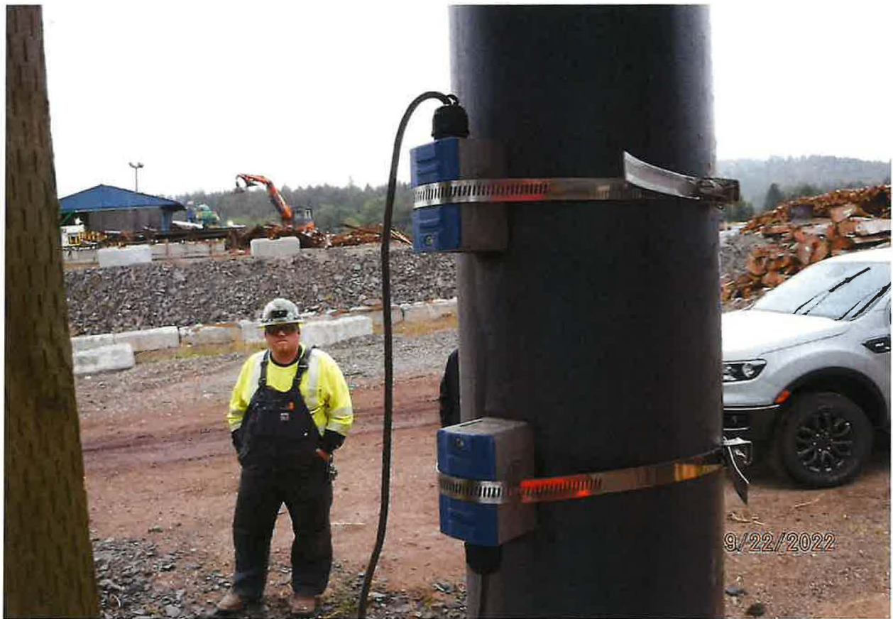
FLOWMETER INSTALLED ON MAIN SERVICE PIPE PRIOR TO REACHING STORAGE TANK
