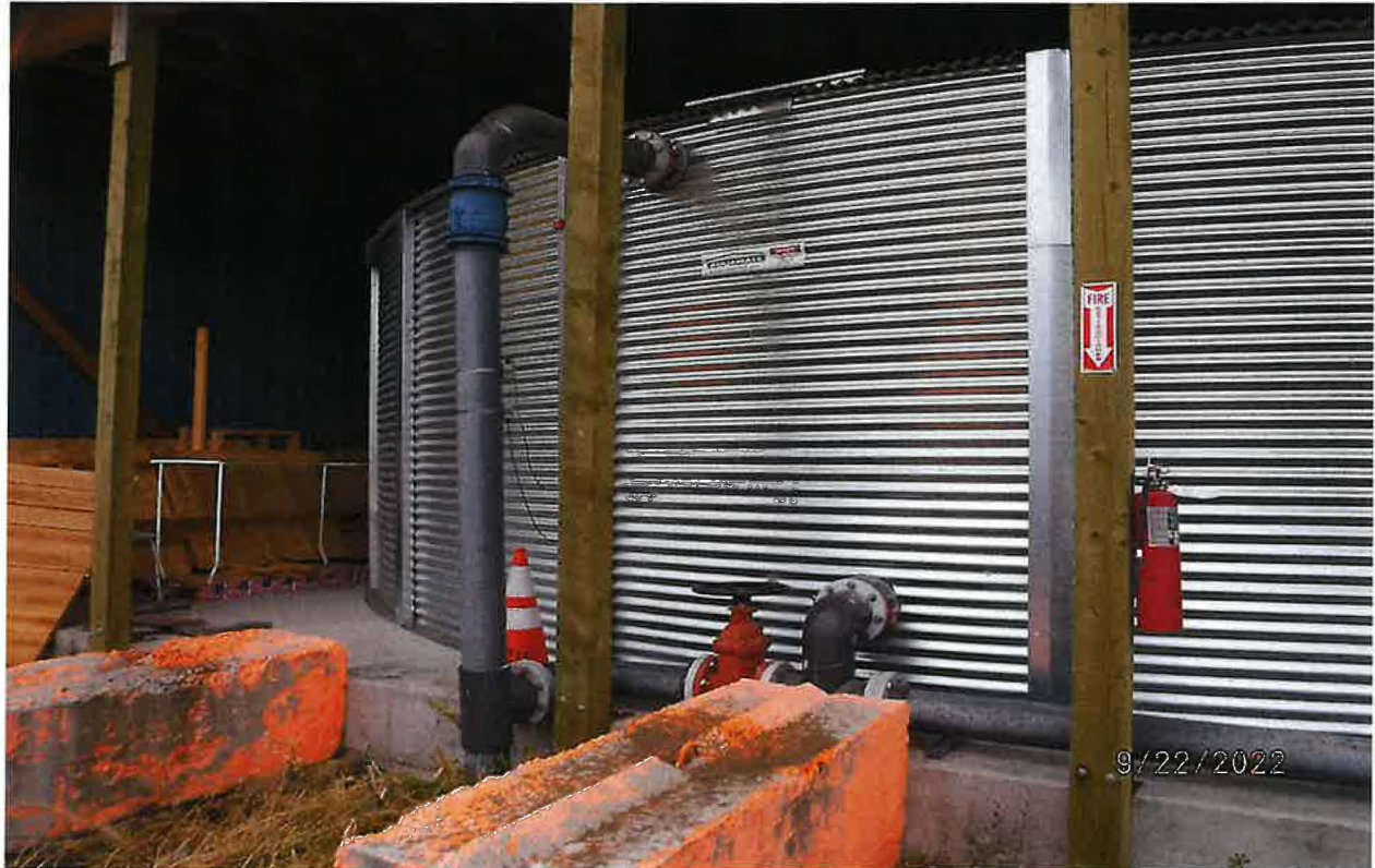
100,000 GALLON STORAGE TANK – INFLOW VERTICAL LINE TO STORAGE & OUTFLOW TANK TO USE(S) PIPELINE
