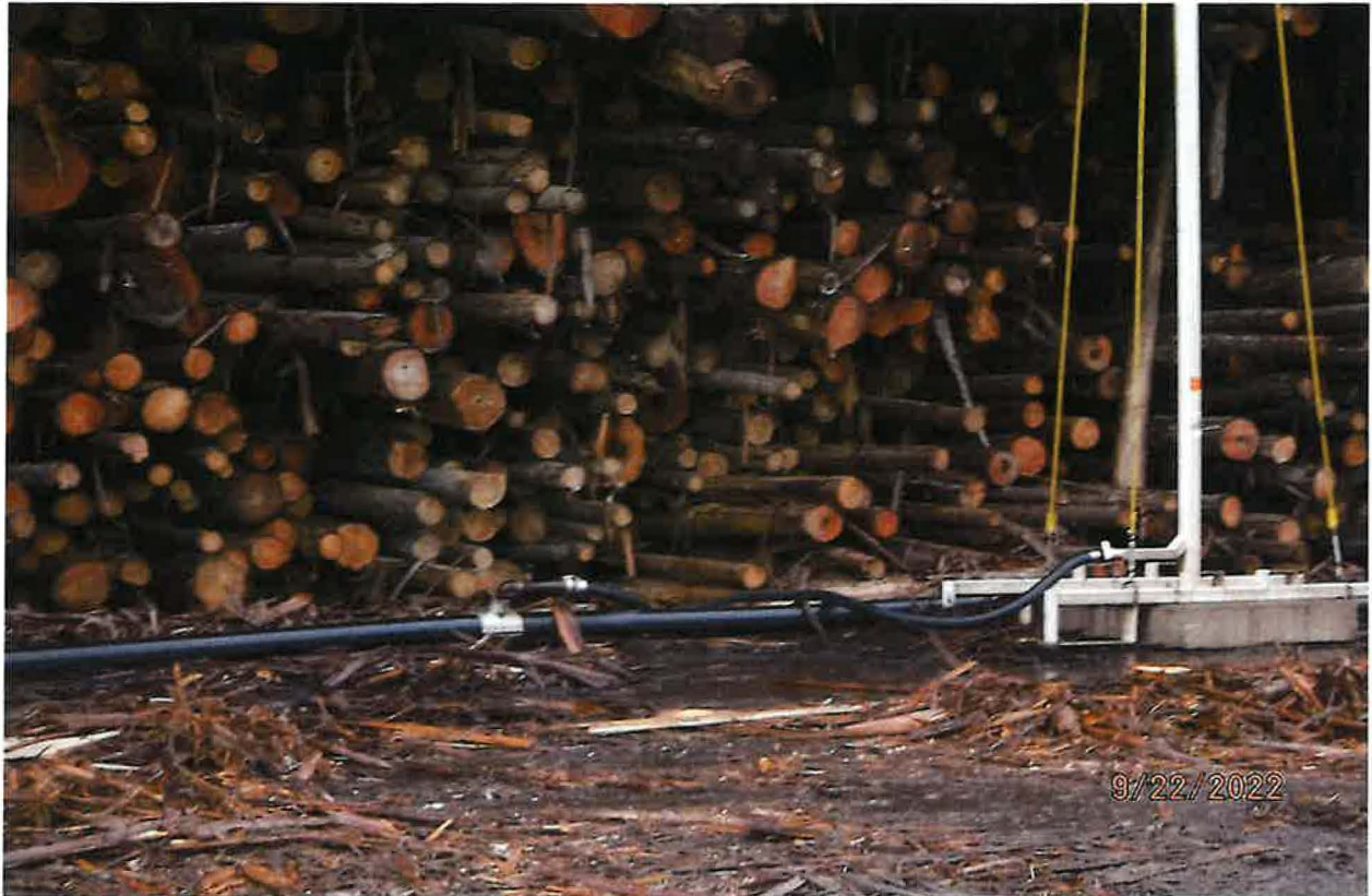
MULTIPLE LATERAL WATER LINES TO SPRINKLER RISERS FROM RECIRCULATION POND SYSTEM
