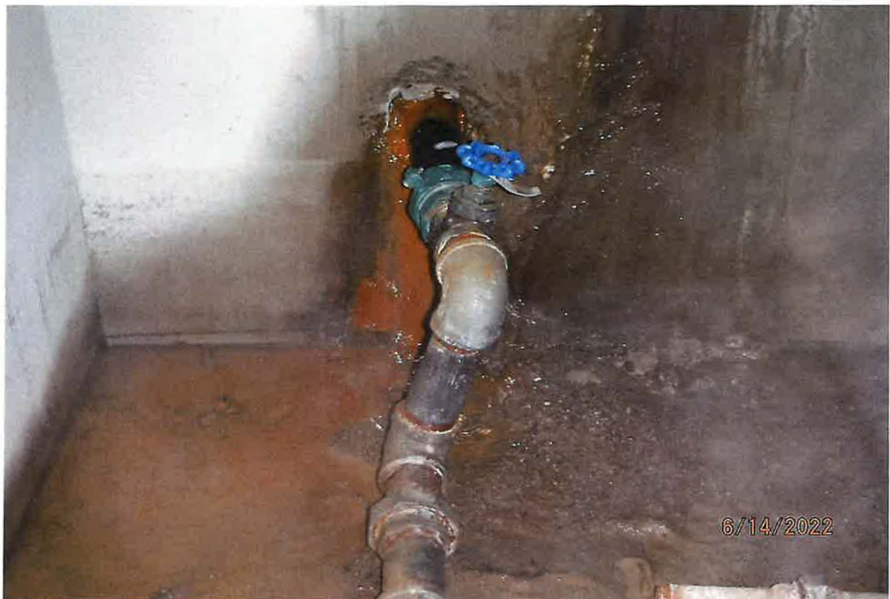
MAIN SERVICE PIPE FROM WELL TO VAULTED PUMP STATION
