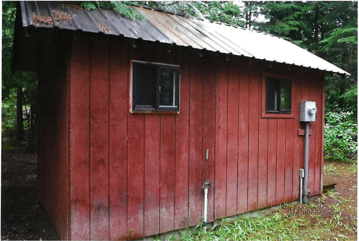
PUMP HOUSE CO-LOCATED WITH WELL
