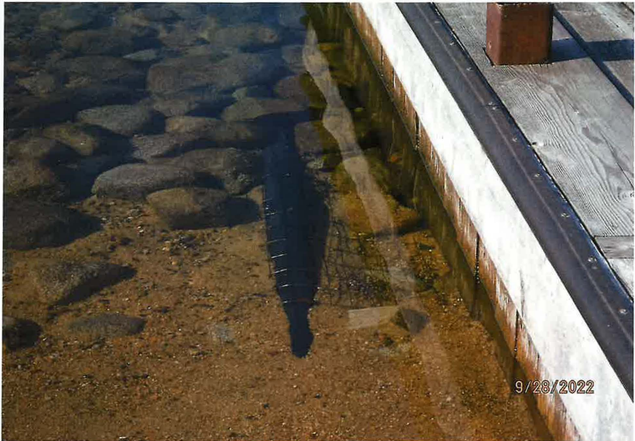
INTAKE PIPE ROUTES ALONG DOCK INTO LAKE
