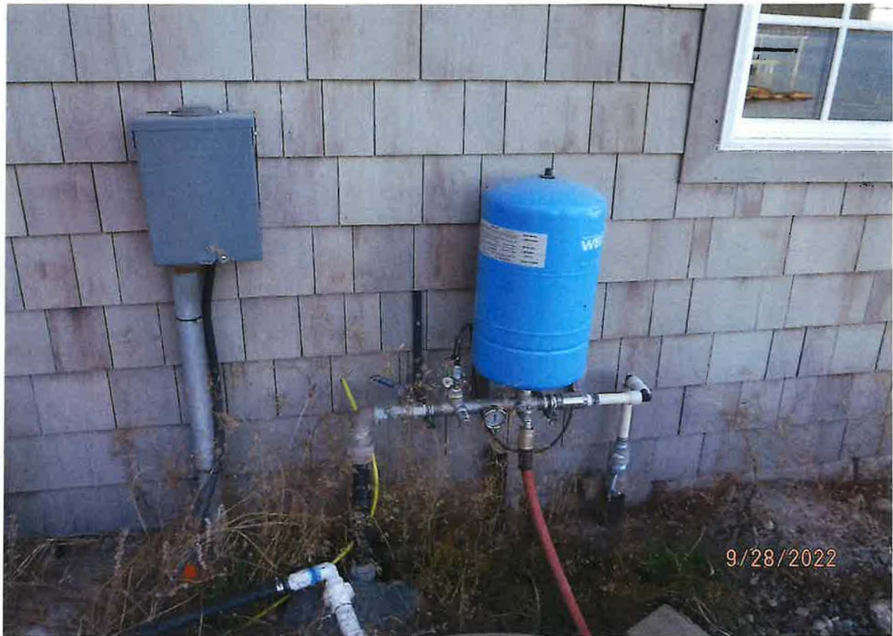
FROM INTAKE PIPE TO SMALL PRESSURE POT BEFORE DISTRIBUTION TO WATER USES
