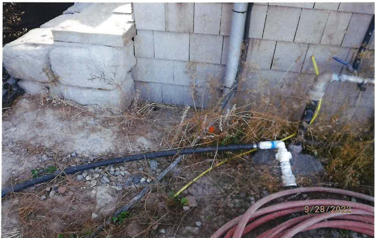
MAIN SERVICE LINE TO HOME
