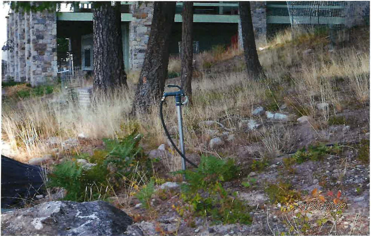
IRRIGATION POU – FROST FREE HYDRANT TO HOSE & SPRINKLER
