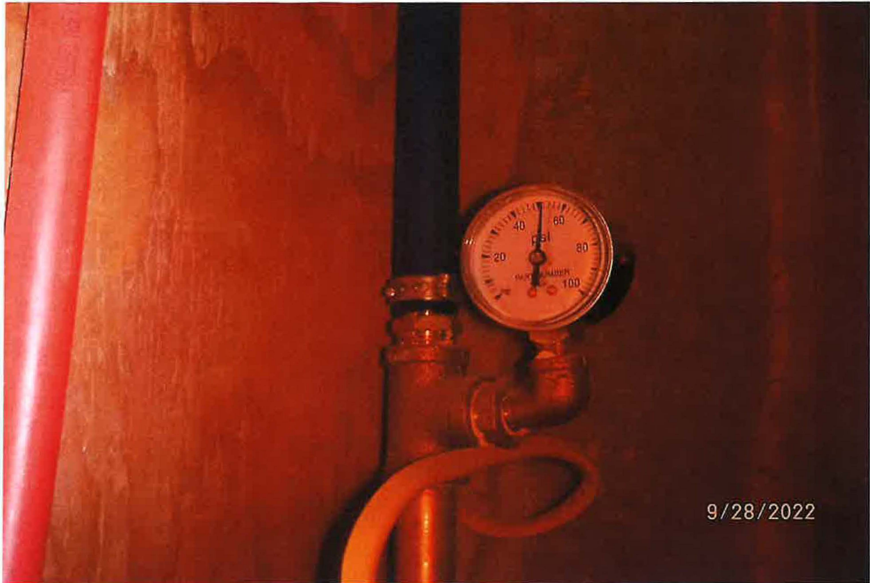
50 PSI WATER SYSTEM OPERATING PRESSURE
