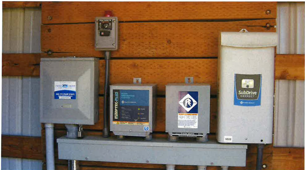
PUMP HOUSE OVERVIEW
