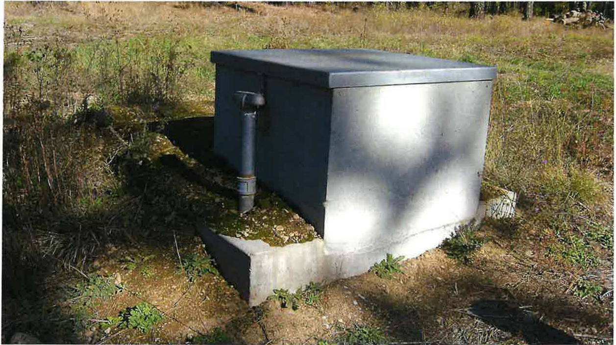
CONCRETE VAULT CONTAINING PRESSURE TANK AND ON/OFF VALVES FOR WATER TO EACH HOME
