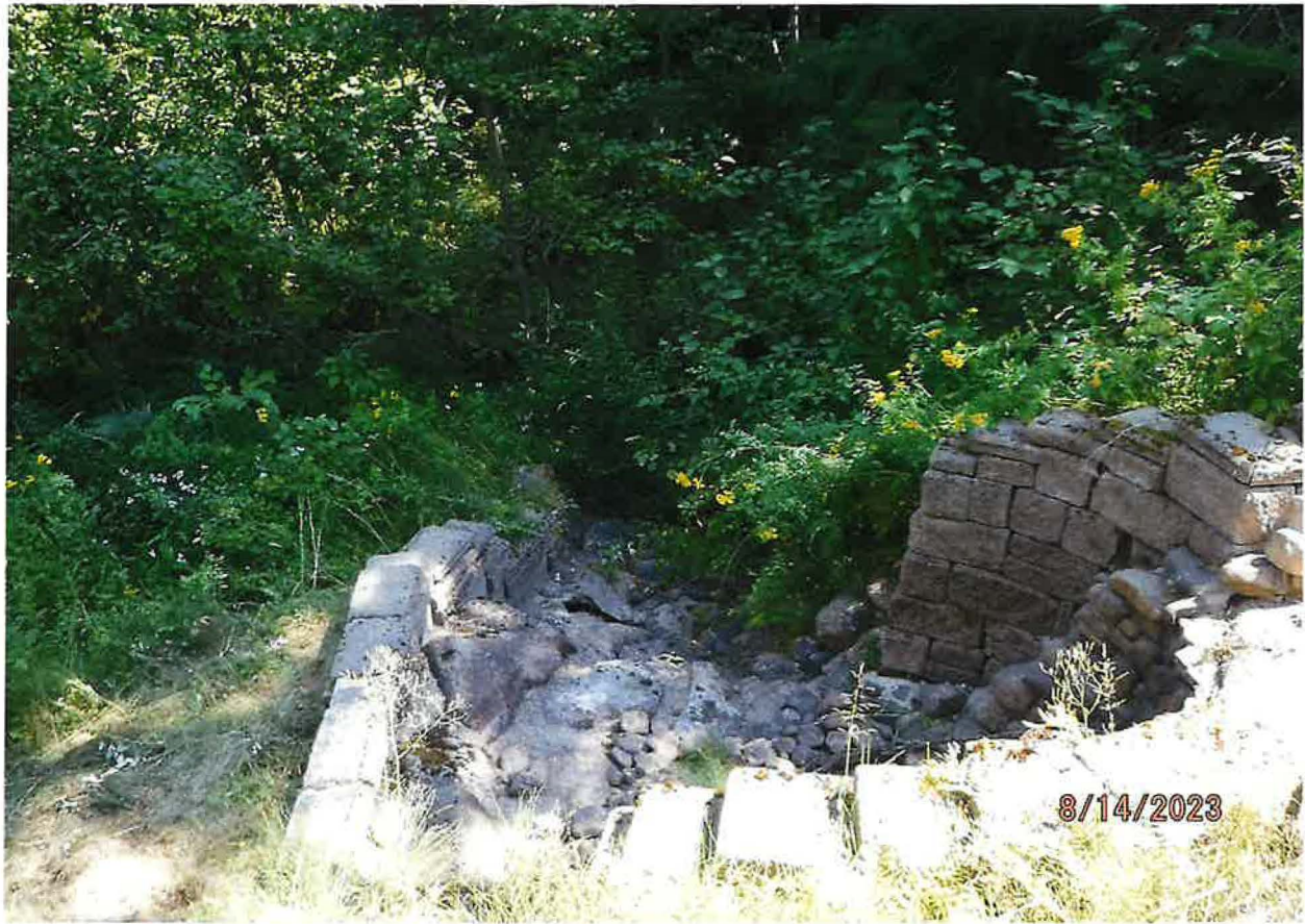
PRIMARY OVERFLOW DISCHARGES DOWNSTREAM USING NATURAL CHANNEL ADAPTED TO CREATE A SMALL WATER FEATURE
