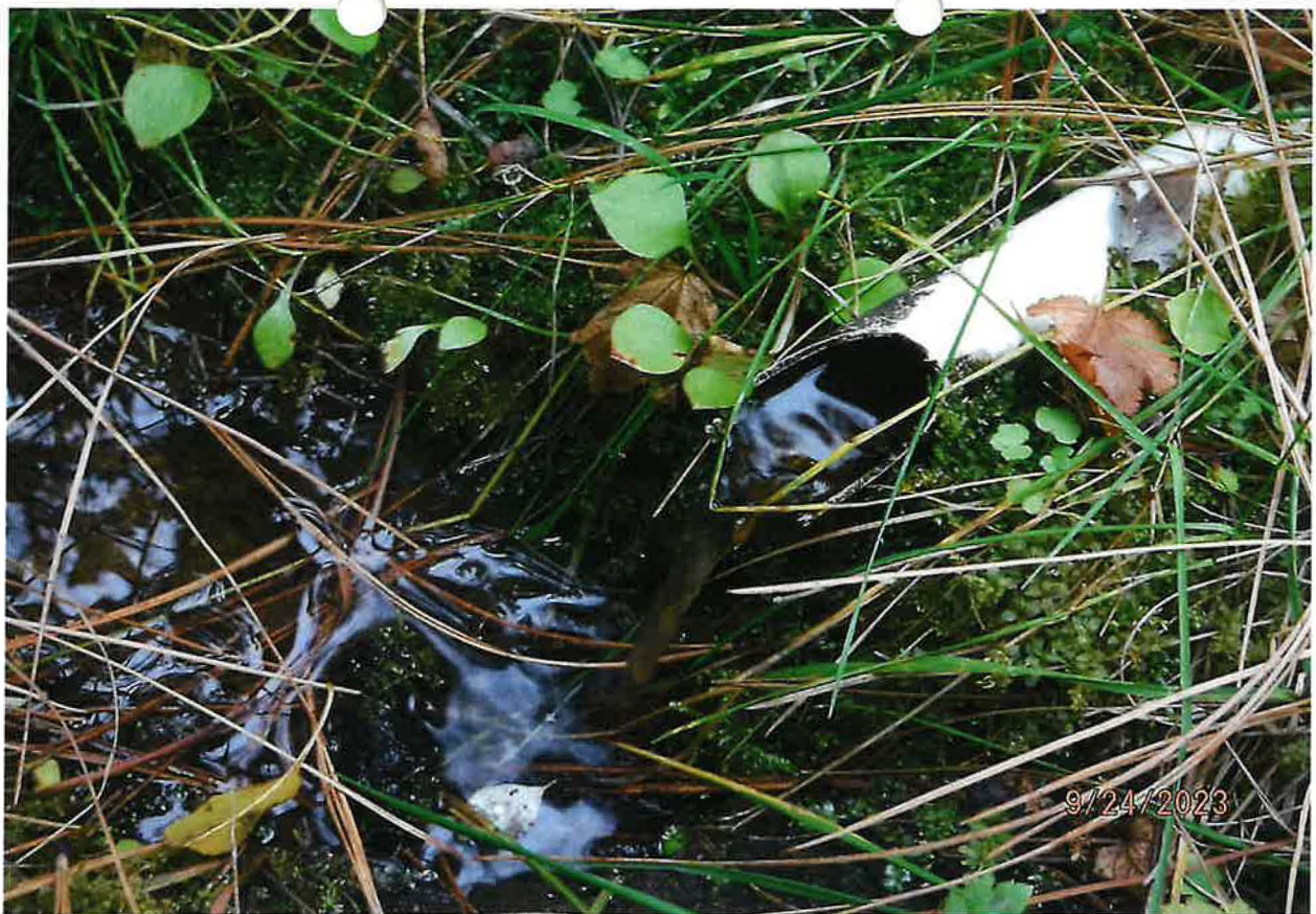
OVERFLOW DISCHARGE FROM STORAGE RESERVOIR
