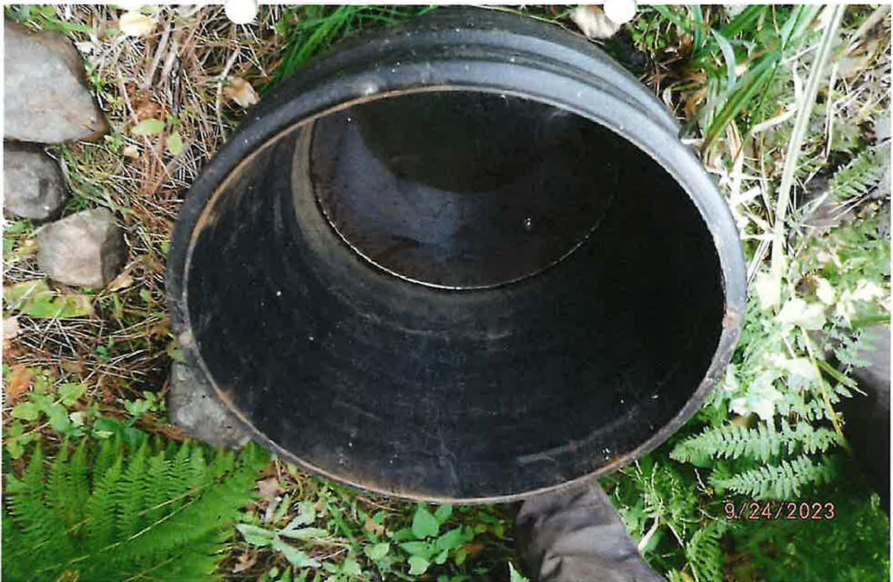
POD – SPRING SOURCE FILLS TO APPROXIMATELY GROUND LEVEL AND HAS 1" PIPE GRAVITY FLOWING TO A 550-GAL STORAGE RESERVOIR PRIOR TO DISTRIBUTION FOR BENEFICIAL USE
