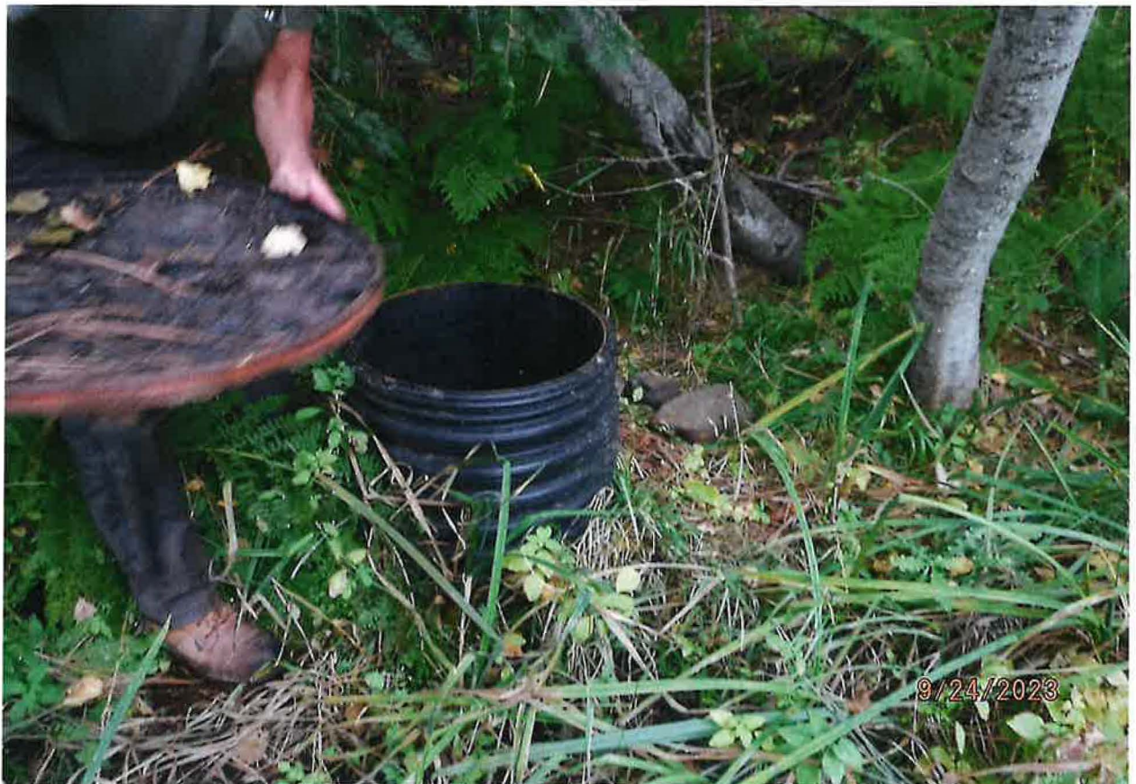
POD – SPRING SOURCE WITH VERTICAL CORRUGATED PIPE VERTICALLY INSTALLED SERVING AS A SPRING BOX
