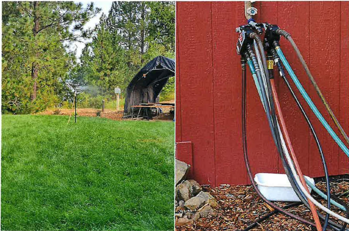
POU - IRRIGATION SPRINKLER SYSTEM RUNNING
