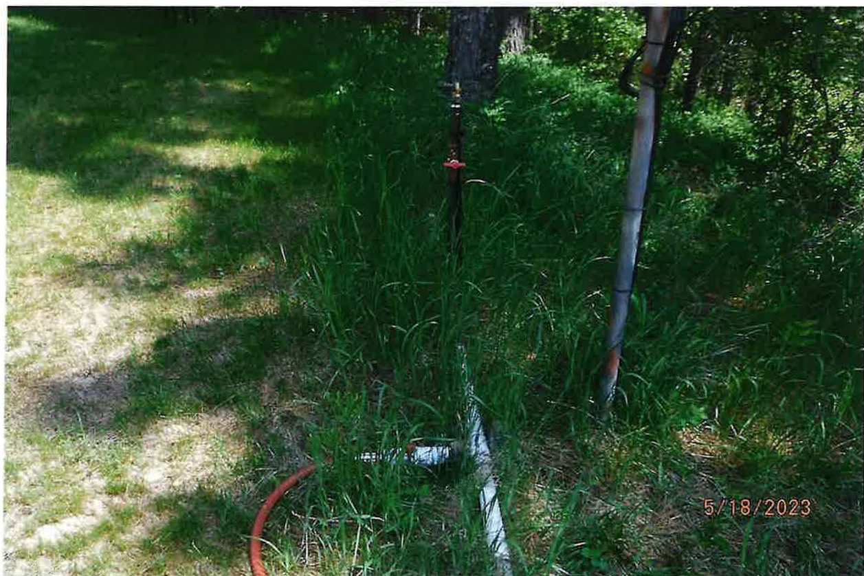
IRRIGATION RISER PIPE WITH IMPACT SPRINKLER
