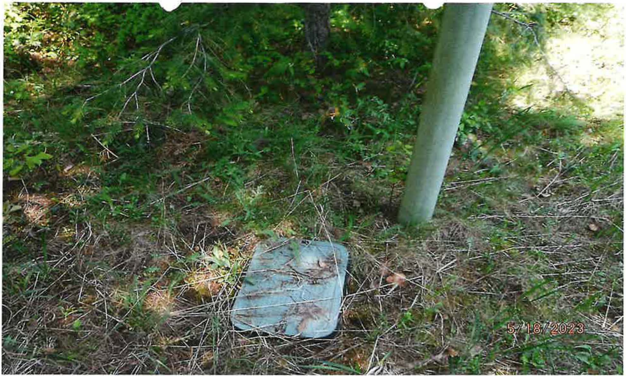
IRRIGATION POU – CONVEYANCE SYSTEM INCORPORATES PVC MAIN TRUNK LINES WITH HOSE BIBS AT INTERVALS THROUGHOUT THE ENTIRE POU, HOSE TO TRIPOD IMPACT SPRINKLERS WITH 5/32 ND NOZZLES.
