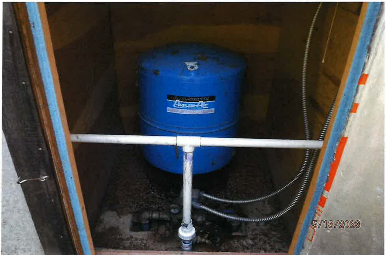
SMALL PUMP HOUSE WITH PRESSURE TANK
