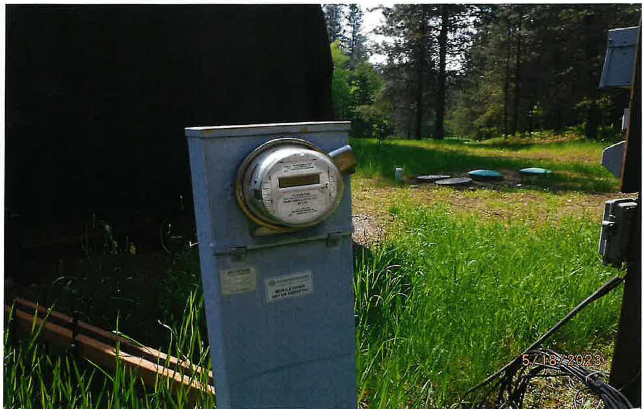
DEDICATED POWER METER FOR RV SITE
