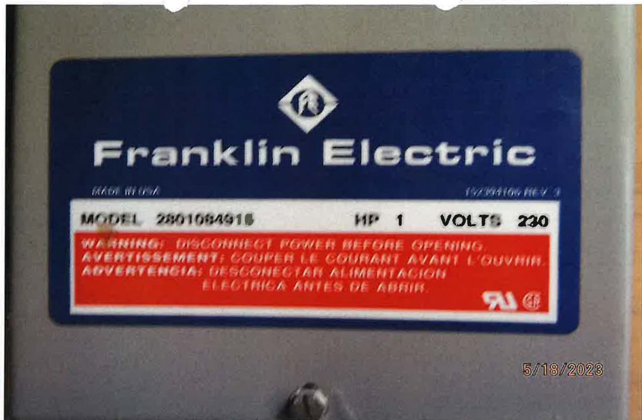
1 HP FRANKLIN ELECTRIC PUMP MOTOR INSTALLED IN WELL
