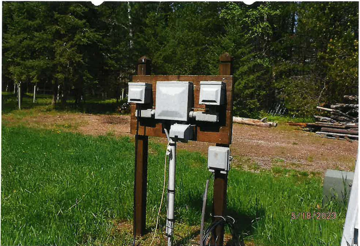
DOMESTIC ELECTRIC CONTROL PANEL BOARD
