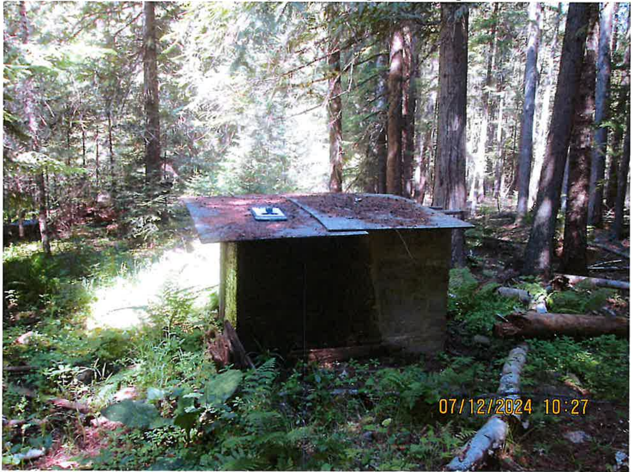
Photo 2: concrete cistern holding water before gravity feeding to residence.
