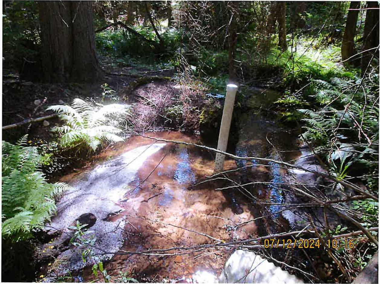
Photo 1: showing wide spot in Alder Creek with perforated intake pipe and aluminum culvert allowing water to flow past POD.
