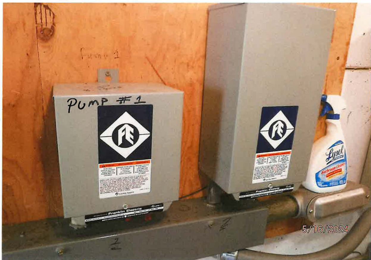
TWO PUMPS INSTALLED DOWN HOLE IN 10" CASED WELL (No.1 & No.2)
