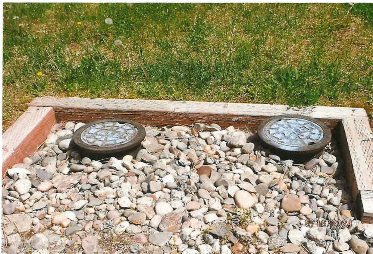
WATER MAIN ROUTES ACROSS ROAD FROM PUMP STATION TO A TEE IN THE SYSTEM. MANUAL SHUTOFF VALVES INSTALLED IN SYSTEM FOR EACH FORK IN THE MAIN LINE
