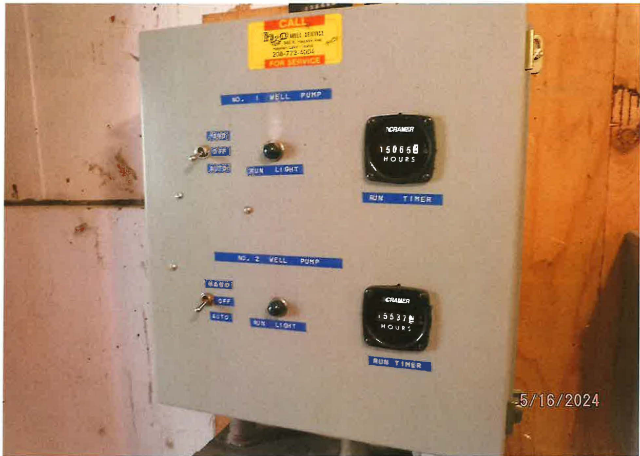
DIVERTING WORKS – PUMP CONTROL PANEL
