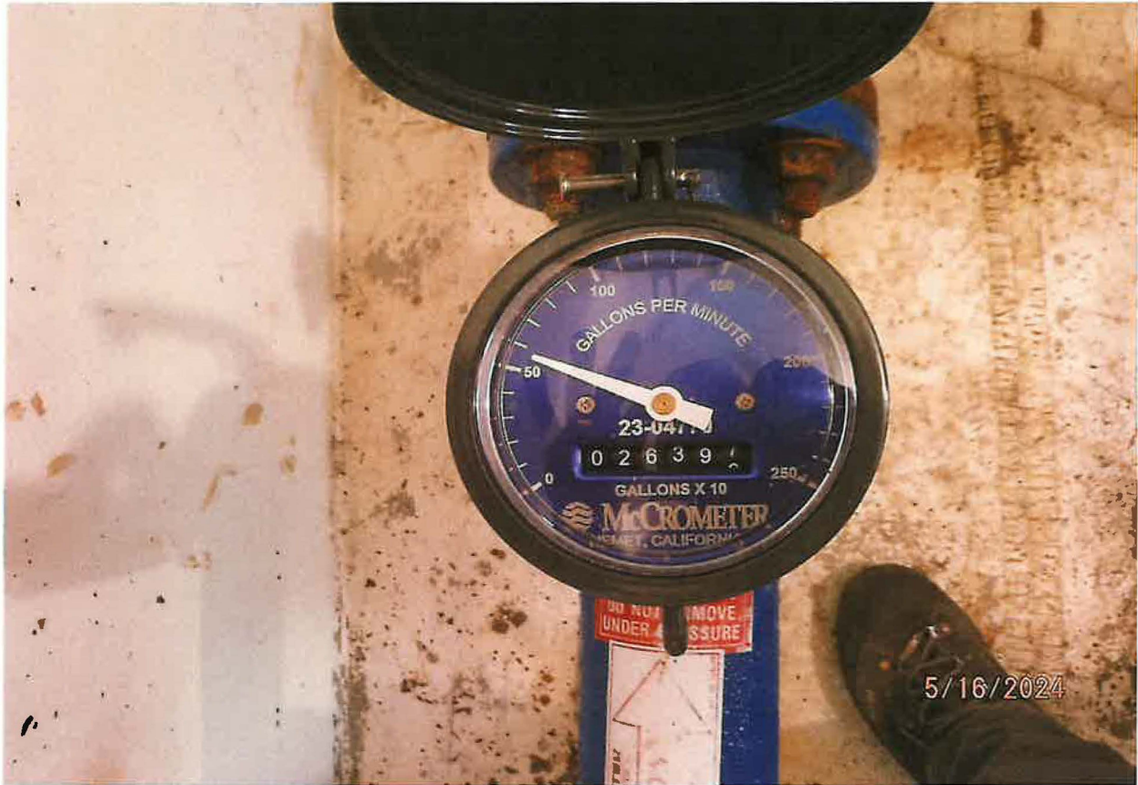
DIVERTING WORKS – McCROMETER FLANGED VELOCITY STYLE FLOWMETER INSTALLED ON SYSTEM
