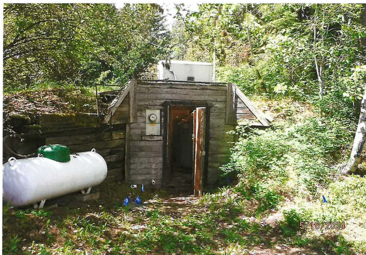
PUMP STATION – LOCATED IN FRONT OF WELL (WELL IN GRASS AREA BEYOND VAULTED PUMP STATION)
