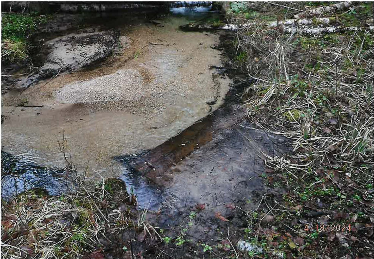
POD – UNNAMED STREAM DIVERSION USING SCREENED WOODEN COLLECTION BOX WITH 2" POLY PIPE GRAVITY FLOWING TO STORAGE POND (DIVERSION TO STORAGE BENEFICIAL USE).
