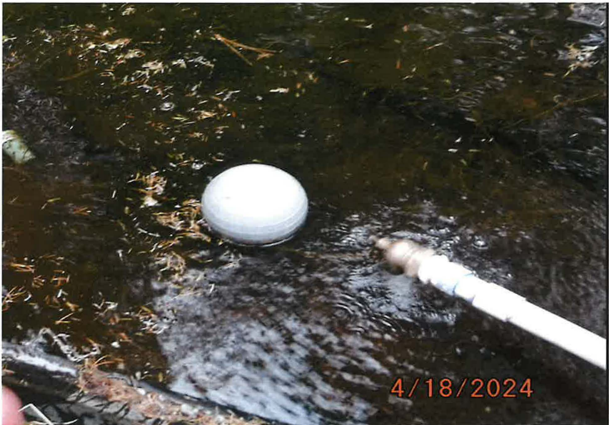
DIVERSION TO STORAGE – PIPELINE IN-FLOWS TO POND WITH FLOAT VALVE ATTACHMENT WHICH CLOSSES WHEN POND REACH FULL POOL LEVELS.
