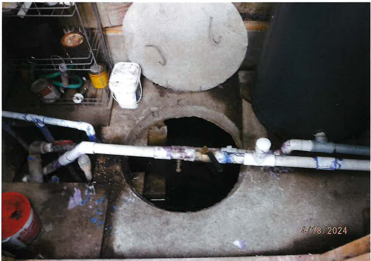
WET WELL IN PUMP STATION WITH PRESSURE TANK USED FOR DISTRIBUTION TO IRRIGATION SYSTEM
