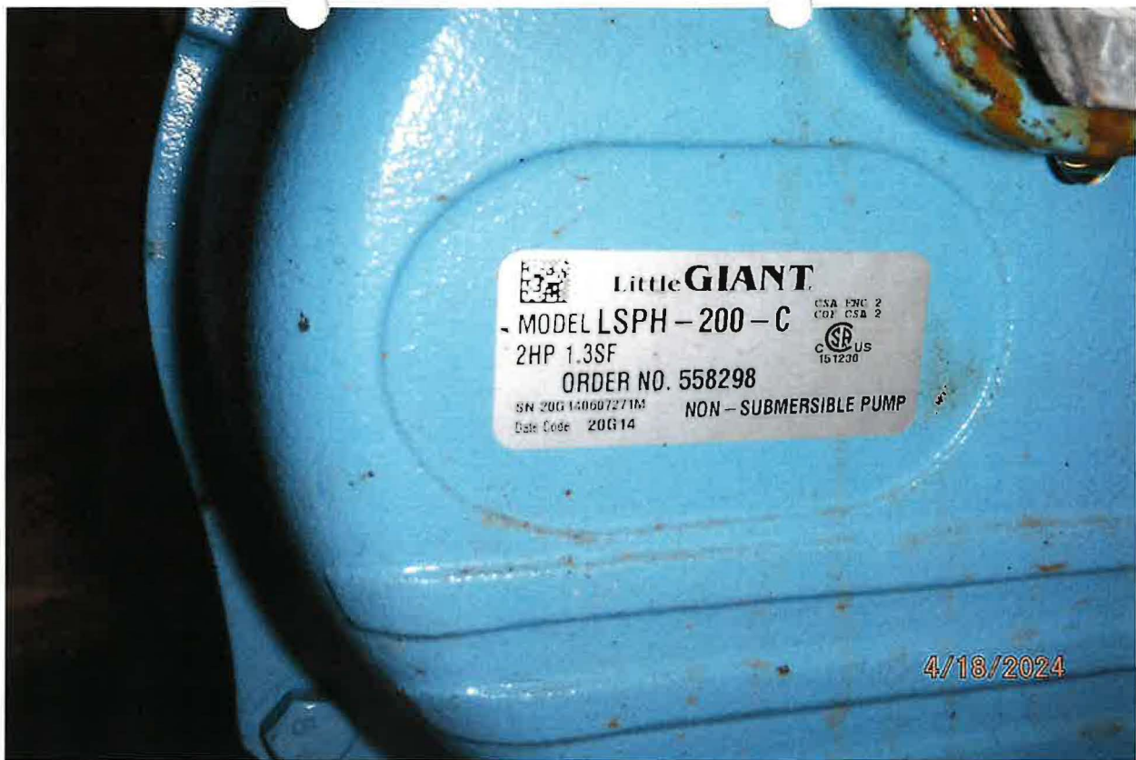
IRRIGATION FROM STORAGE – LITTLE GIANT NON-SUBMERSIBLE PUMP
