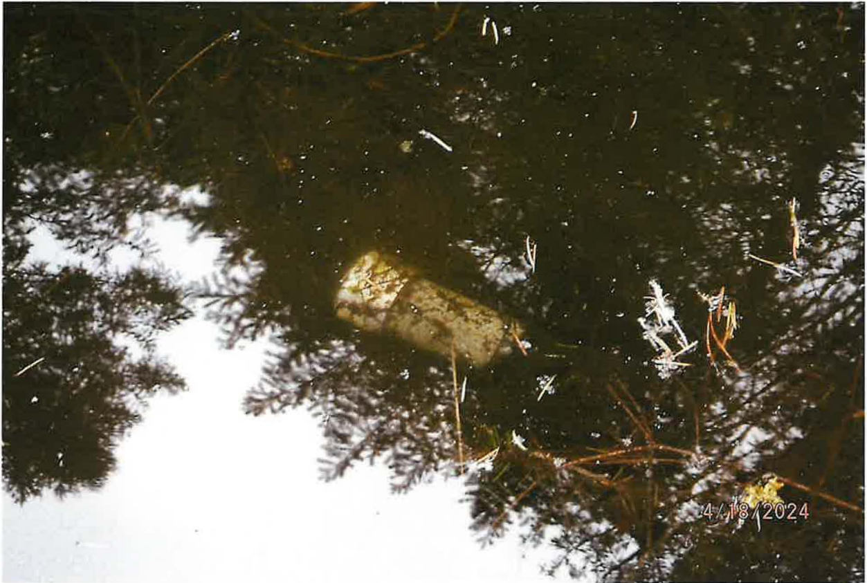
IRRIGATION FROM STORAGE 2-INCH POLY PIPE TO PUMP STATION
