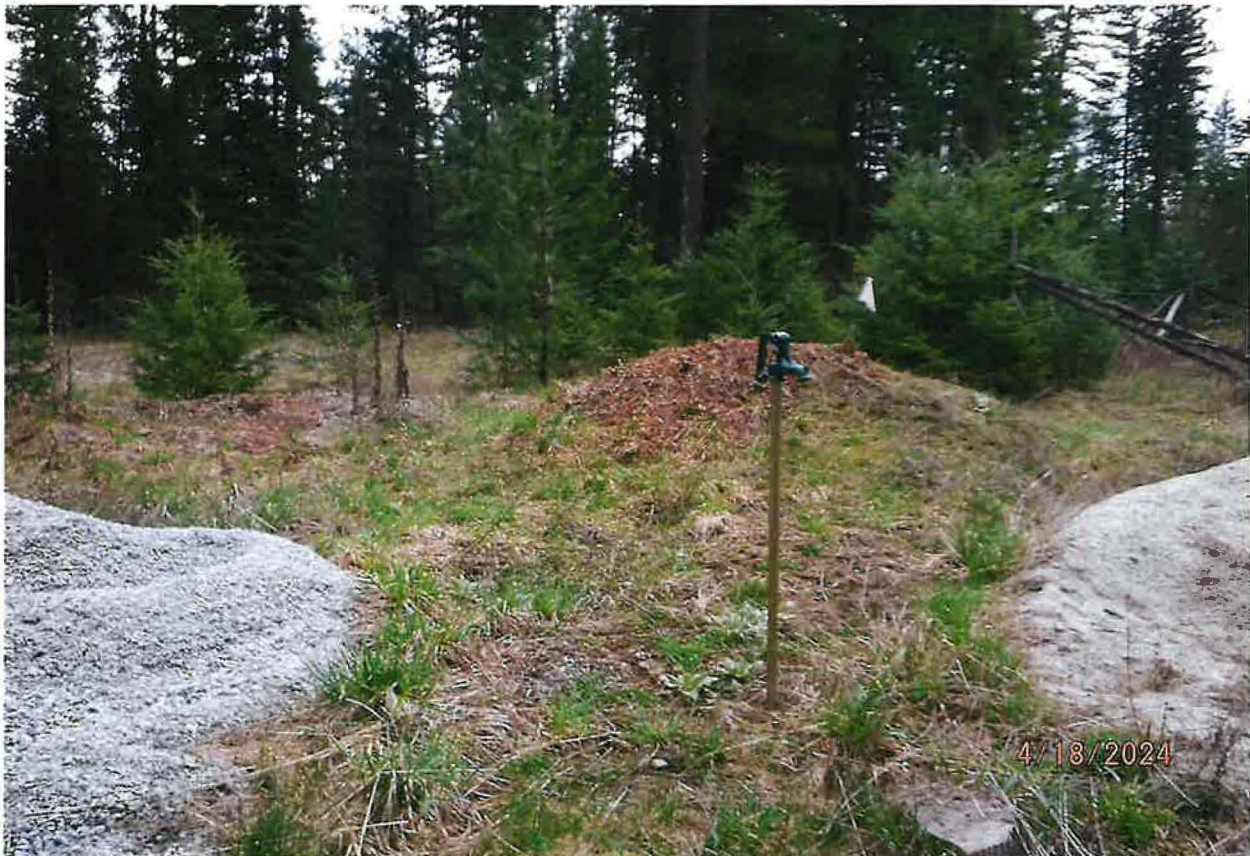
IRRIGATION FROM STORAGE – MUTIPLE FOST FREE HYDRANTS USED BY HOSE AND SPRINKLERS TO WATER TREES AND GARDEN AREA
