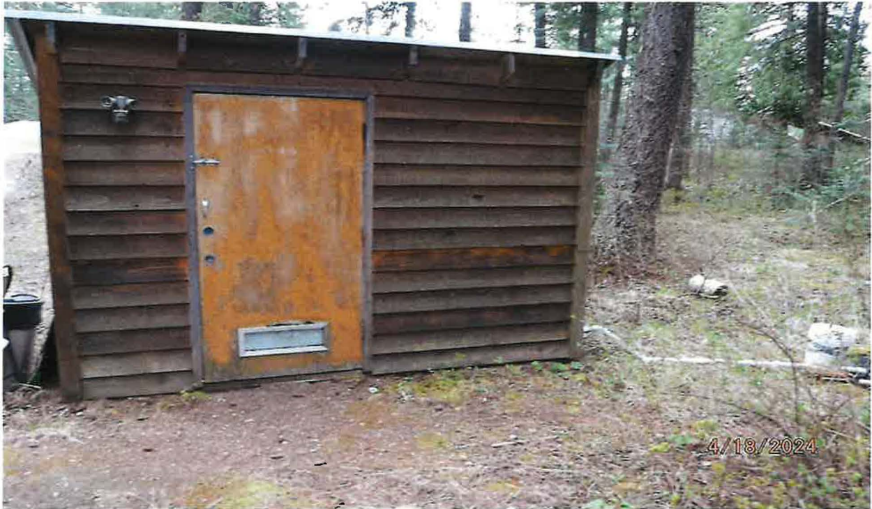
SMALL PUMP STATION WITH WET WELL INSTALLED, FILLED FROM POND PRIOR TO TRANSFER PUMP DISTRIBUTING TO MULTIPLE FROST-FREE HYDRANTS AND IRRIGATION FROM STORAGE BY ZONE PRESSURIZED WATERING
