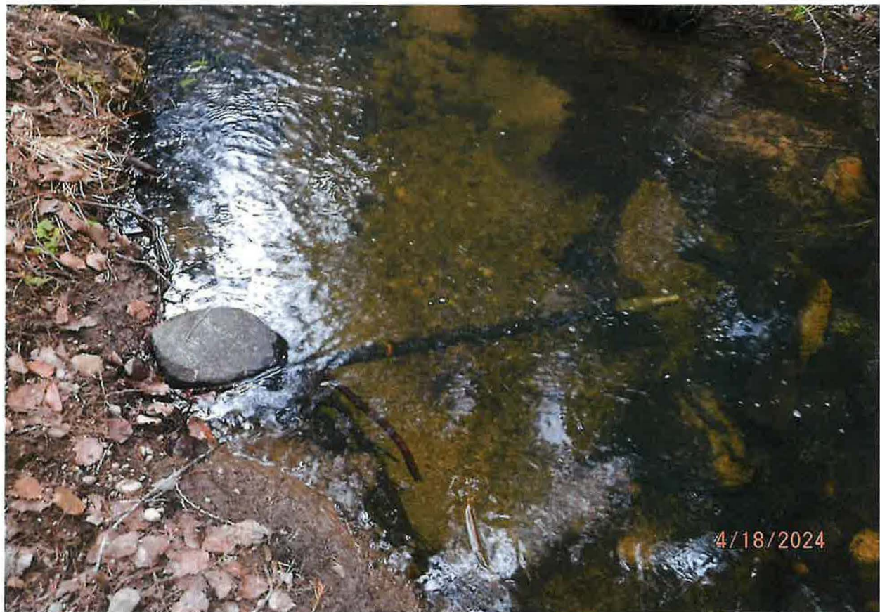
POD - 1 1/4" POLY PIPE INTAKE WITH 1/4" FISH SCREEN INSTALLED IN UNNAMED STREAM
