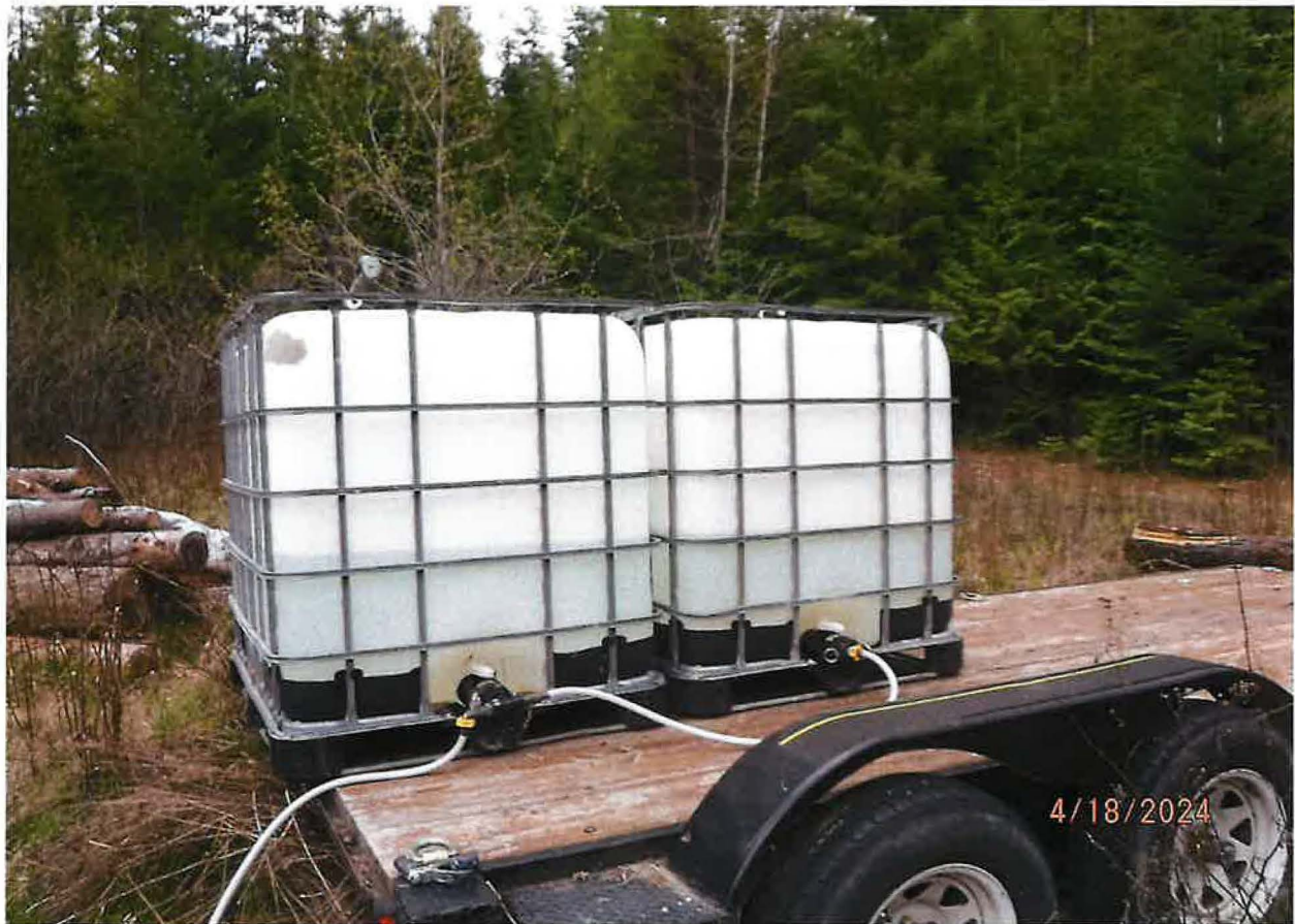
FIRE PROTECTION POU – STREAM WATER USED TO FILL 2 TRAILER MOUNTED 275-GAL TANKS USED FOR DOMESTIC & PREPARED FOR FIRE PROTECTION USES.
