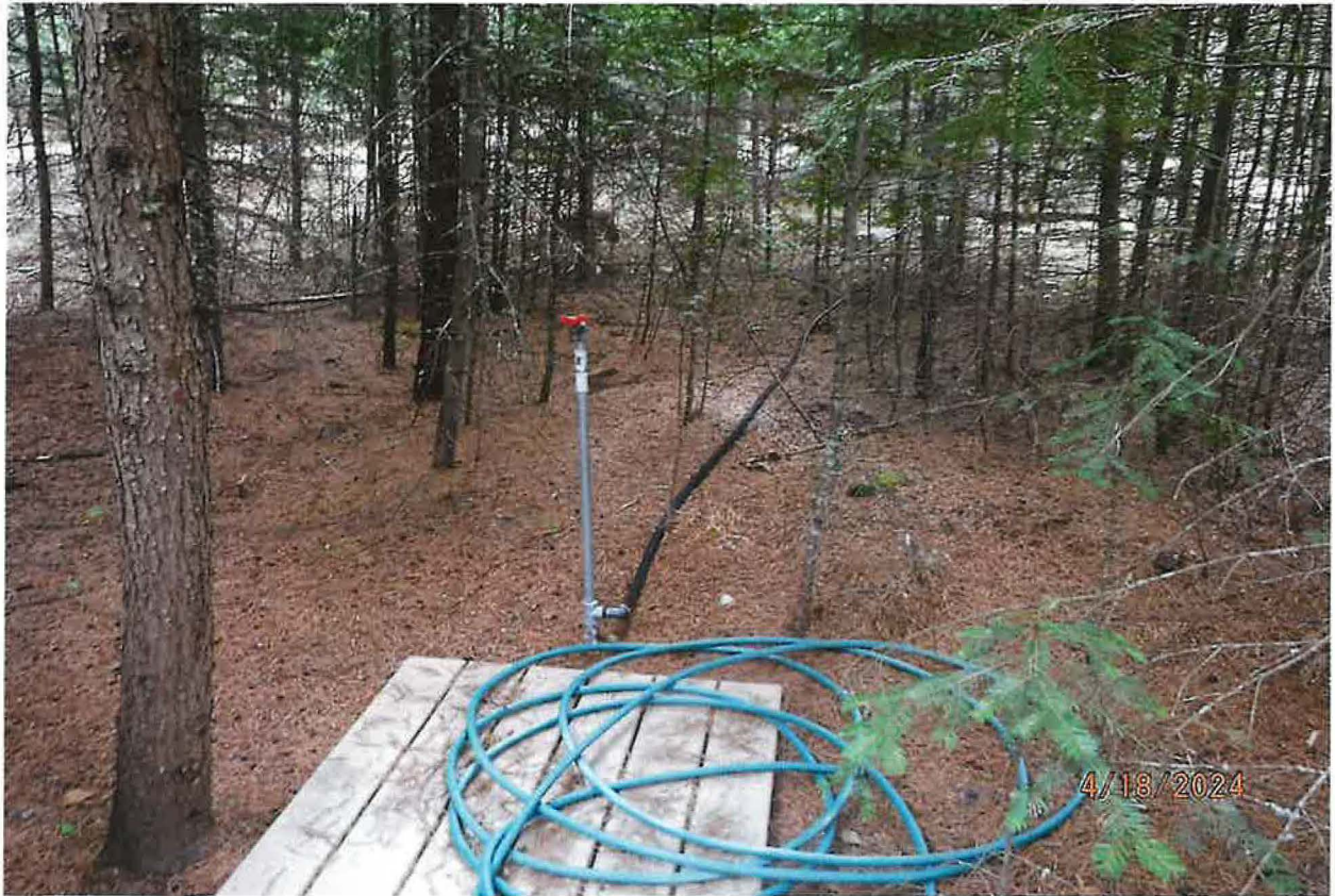
1 OF 3 FROST-FREE HYDRANTS INSTALLED IN WATER SYSTEM
