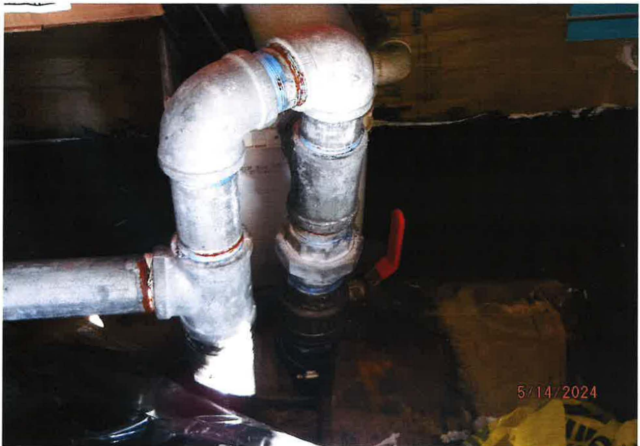
INFLOW FROM WELL TO PUMP STATION (L/H PIPELINE) AND OUTFLOW TO WATER DELIVERY SYSTEM WITH MANUAL SHUTOFF VALVE (R/H)
