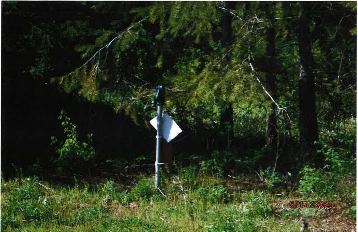
MULTIPLE FROST-FREE HYDRANTS INSTALLED OFF WATER MAIN LINE FOR LAWN/LANDSCAPE IRRIGATION ON LOT 4
