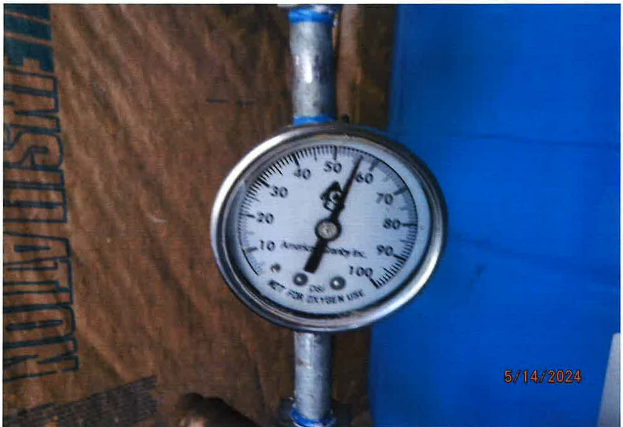
WATER SYSTEM STATIC PRESSURE HOLDS AT 55 PSI
