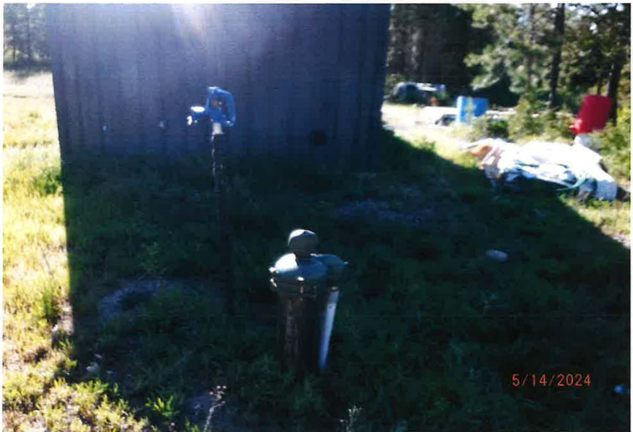
POD – GW WELL AND PUMP STATION IN BACKGROUND
