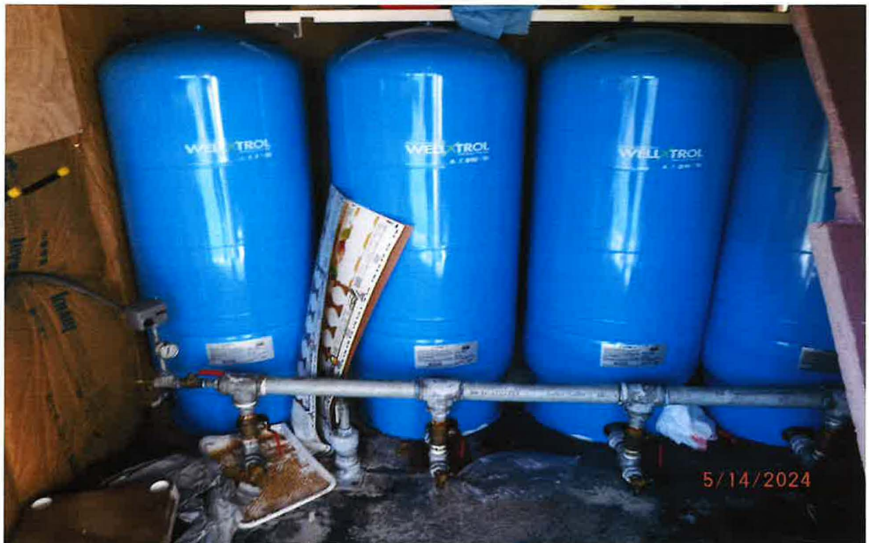
SIX PRESSURE TANKS ASSOCIATED WITH THIS WATER SYSTEM; NO STORAGE INCORPORATED
