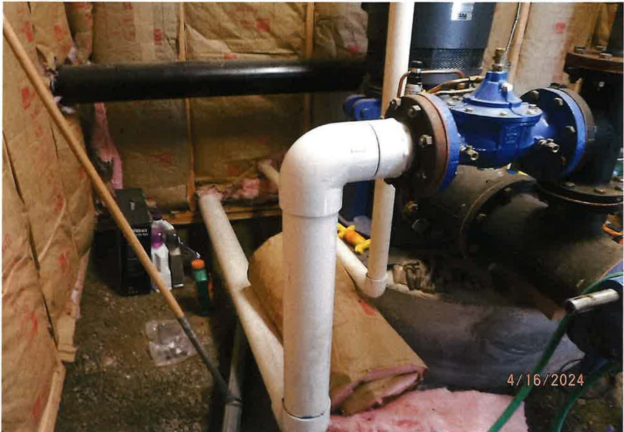
TWO PVC PIPE RUNS OVERFLOW FROM SYSTEM AND WELL PUMP TO STORAGE PIPELINES USE TO FILL POND
