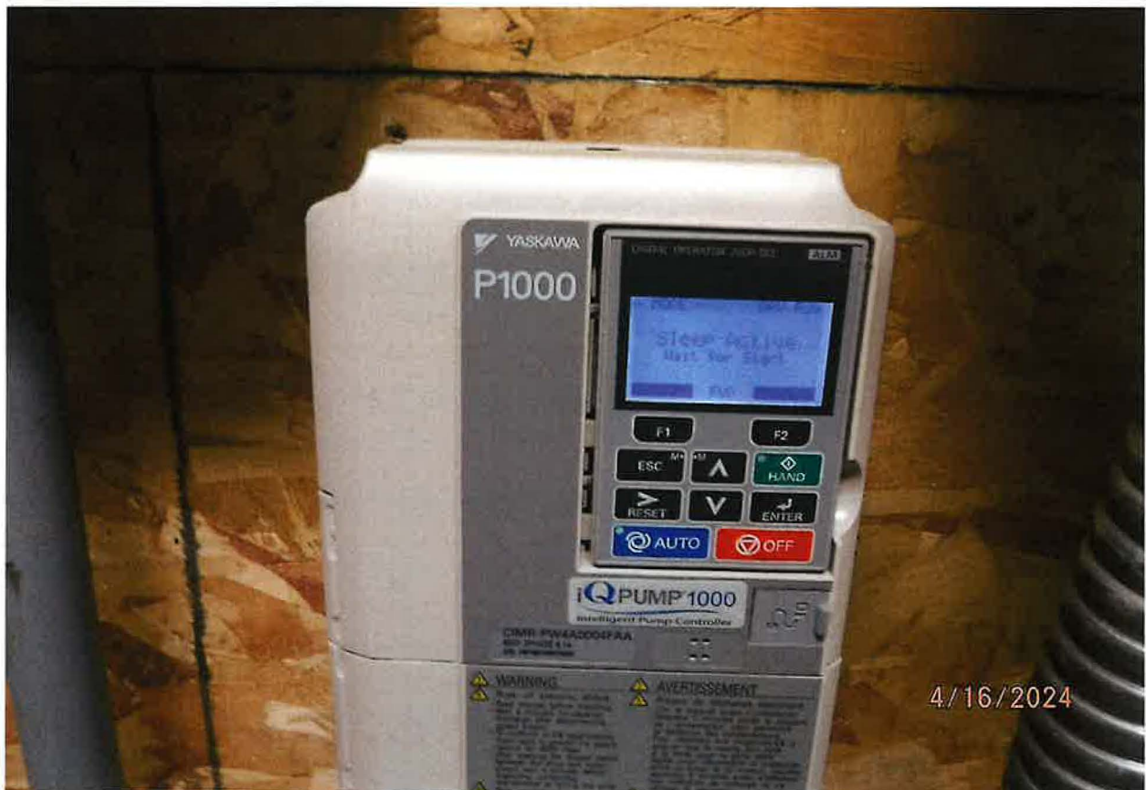
IRRIGATION FROM STORAGE PUMP RELAY CONTROL PANEL
