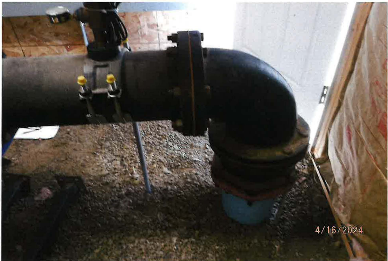
MAIN PIPELINE OUTFLOW TO FIRE PROTECTION SYSTEM
