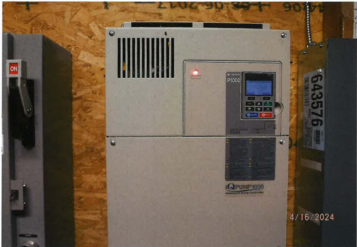
ONE OF THREE PUMP RELAY CONTROL PANELS (FIRE PUMP, WELL PUMP, IRRIGATION PUMP)
