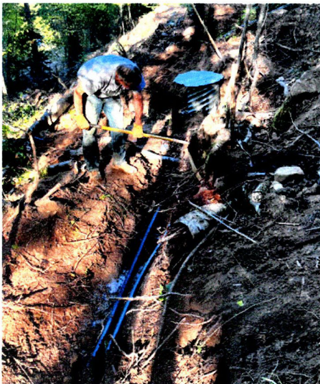
Figure 4: Spring Box Diversion Pipes to Cistern
