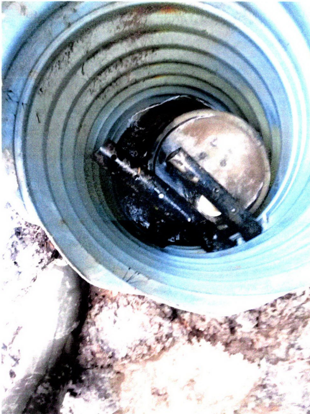
Figure 4: Inside Cistern View; Inlet pipes at top, then overflow and outlet pipe is in one gallon tube.
