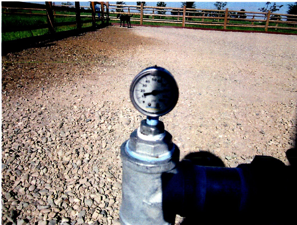
Figure 4. Photograph of pressure gauge near attached to the well. The permit holder informed me it was not working properly and therefore did not give a proper reading.
