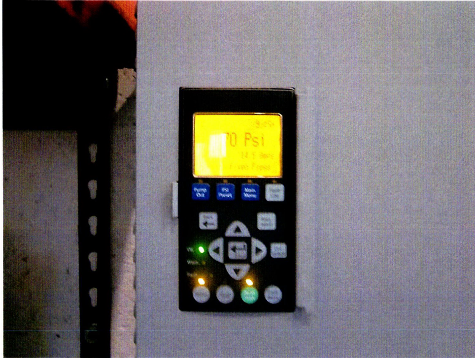
Figure 5. Photograph of pump controlling unit displaying operating pressure and Hz.
