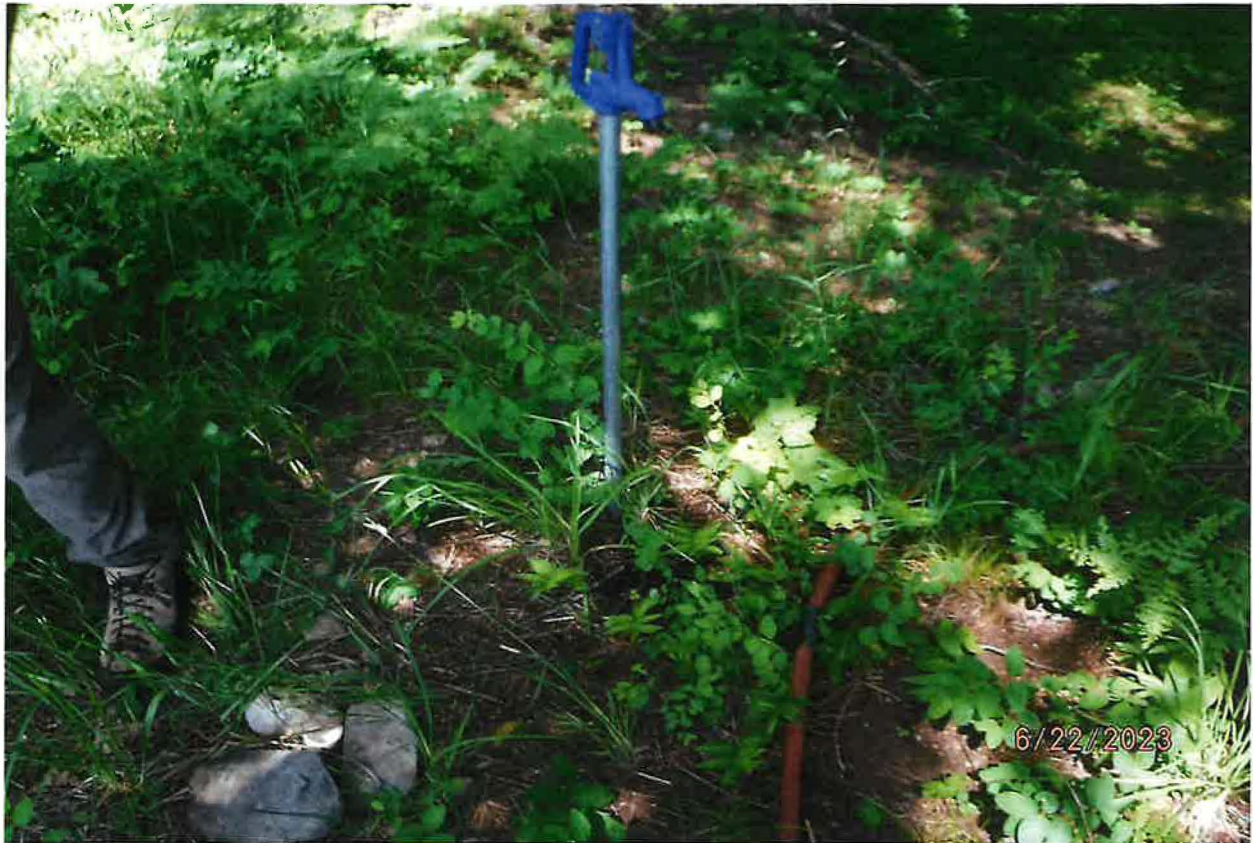
FROST FREE HYDRANT OFF MAIN GROUNDWATER SOURCE PIPELINE – GRAVITY FLOW OPERATIONS
