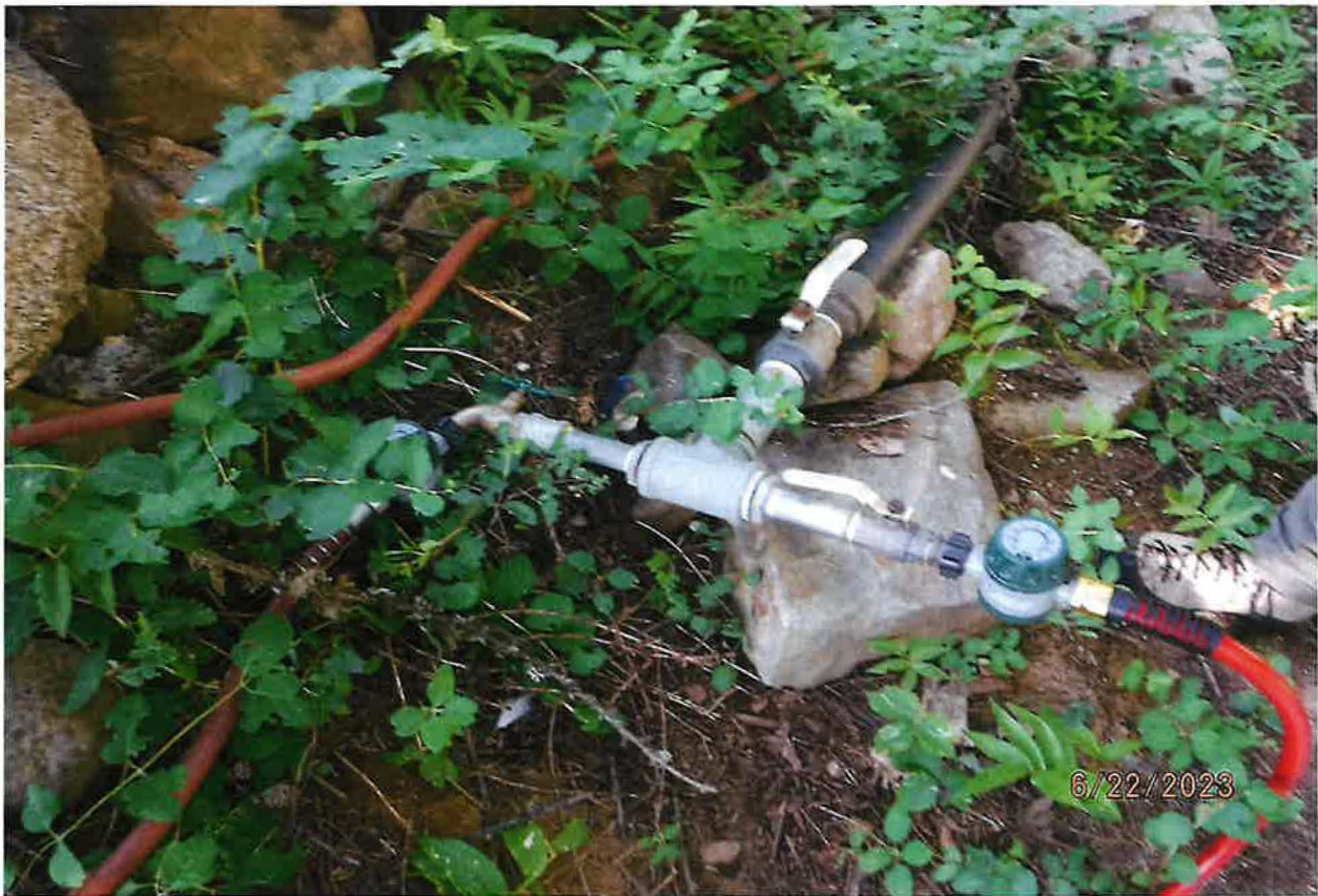
END RUN OF POLY-PIPE TO TWO GARDEN HOSE ATTACHEMENTS
