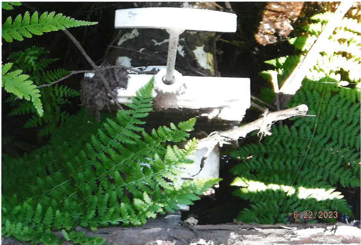
MANUAL SHUTOFF VALVE AT POD - UNNAMED STREAM WATER CONVEYED BY POLY-PIPE RUN TO IRRIGATION SYSTEM
