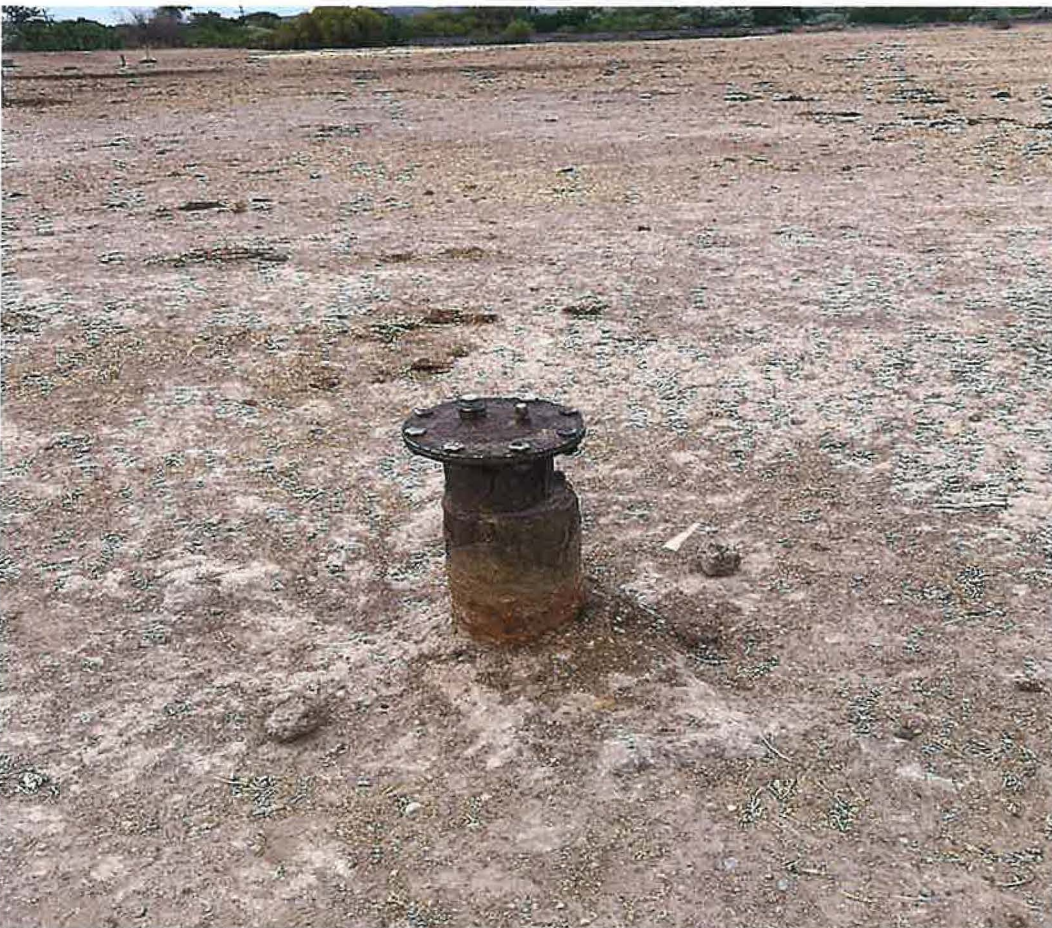
Fig. 6 – Artesian well with 8" casing from 1-40 ft, 6" casing from 1.5-617 ft, and a 4.5" casing from 605-945 ft. This well supplies water to a trough that is West of the coral.
