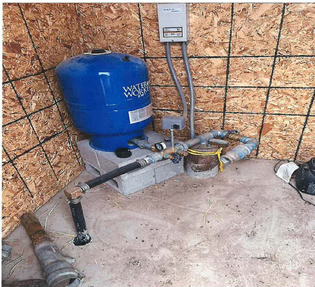
Fig. 2 – Well with 8" casing from 1-40 ft, completed to a depth of 295 ft. Drilling completed on 10/7/93. A 1-hp pump delivers water into the ~20 gallon pressure tank, then to the middle trough in the coral, or it can be diverted to hand lines for irrigation directly from the well. This is the only well that supplies the irrigation use.
